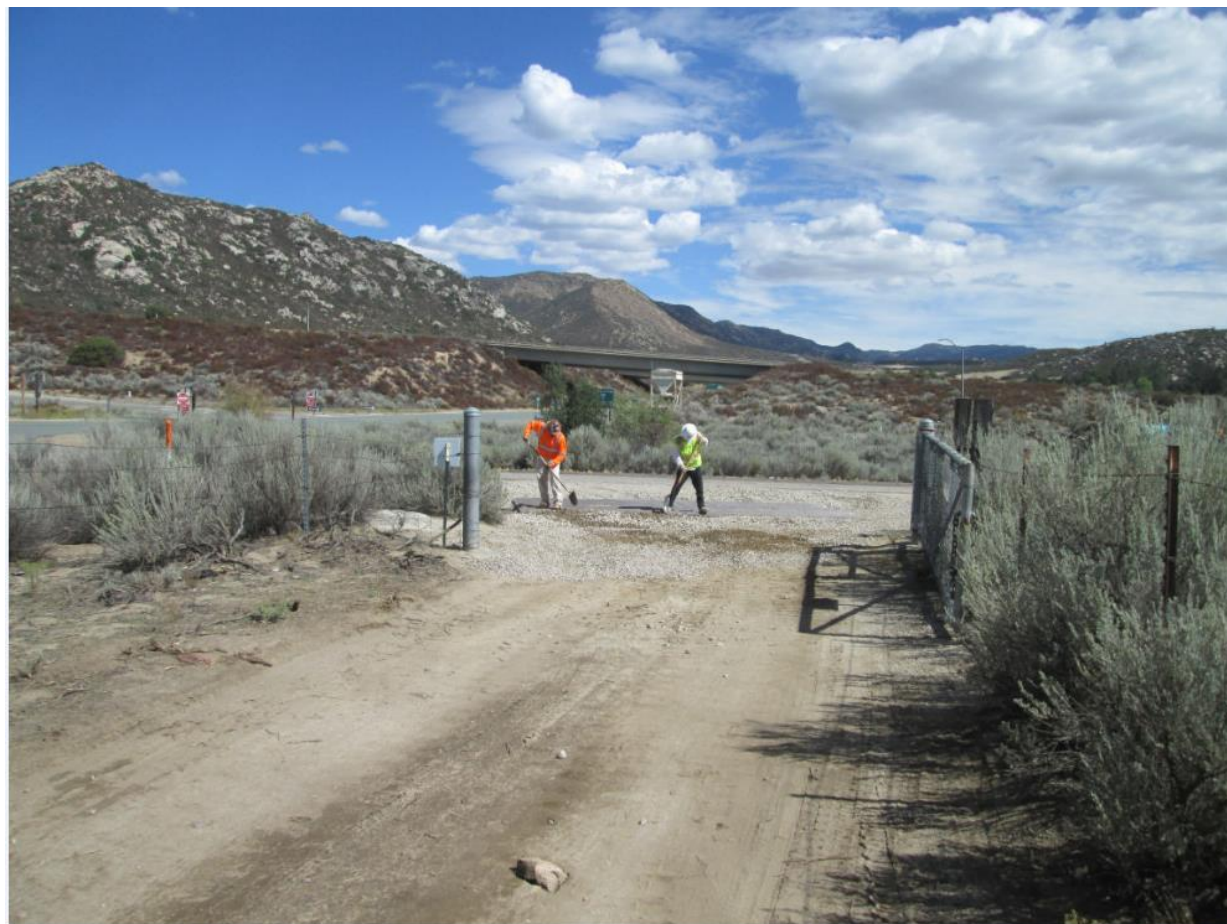
Photo 2: Crews were observed cleaning the rumble plates of sediment and debris at the entrance of the Kitchen Creek Staging Yard in accordance with the SWPPP (APM HYD-05, MM BIO-7, MM HYD-1) and ensuring pavement on was free of track out (APM-AIR-04).
