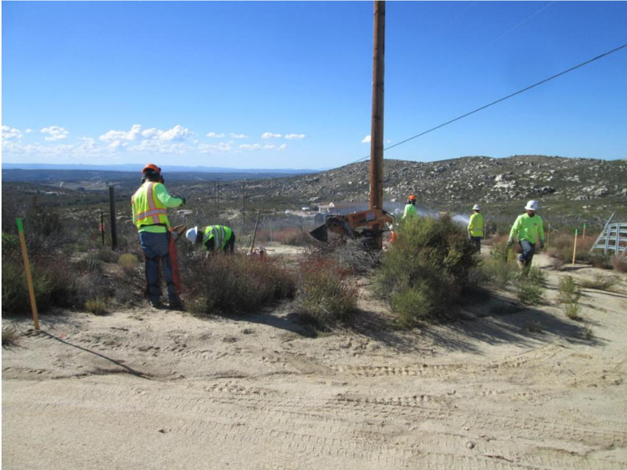
Photo 5: Crews were observed clearing brush and vegetation (manually and by using a chipper) around approved work sites (TL 629E, above) prior to SWPPP BMP installation. Areas were watered down and fire tools were staged adjacent to work areas in accordance with the CFPPP (MM FF-1).
