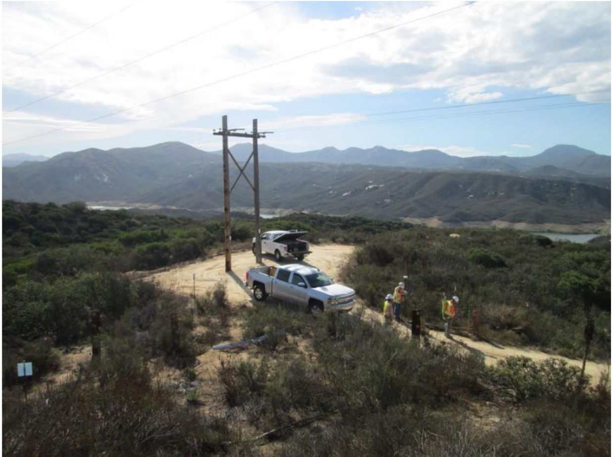
Photo 3: Prior to any work occurring at pole sites, resource crews were observed surveying and staking approved work spaces in the field (TL 625B, above) in accordance with MM BIO-1.
