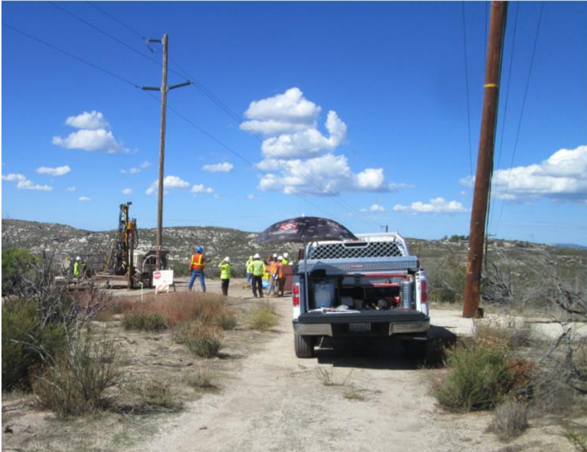
Photo 7: Subsequent to surveying, clearing, and BMP installation, equipment used for steel pole micro pile foundations was mobilized on site. At the work sites, vehicles were observed carrying required fire equipment (5-gallon backpack pump, shovel, Pulaski, and fire extinguisher) and a fire box containing fire equipment was observed staged adjacent to the immediate work areas in accordance with the CFPPP.
