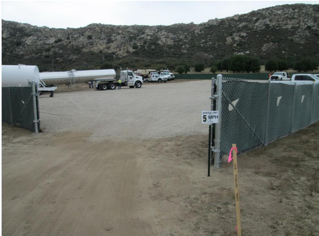
Photo 1: Establishment of the Kitchen Creek Staging Yard included delineating work limits and ESAs, laying gravel foundation, installing a perimeter fence and placing opaque screening material (APM VIS-2). Speed limits were posted at the entrance of the yard, which were less than 15 mph in accordance with APM AIR-03 and MM BIO-24.
