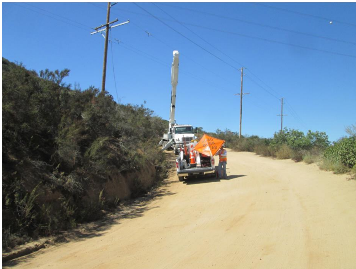
Photo 4: During pole preparation activities within TL 625B access roads, crews were observed using traffic signage to maintain a safe transportation corridor during construction in accordance with APM-TRANS-02.
