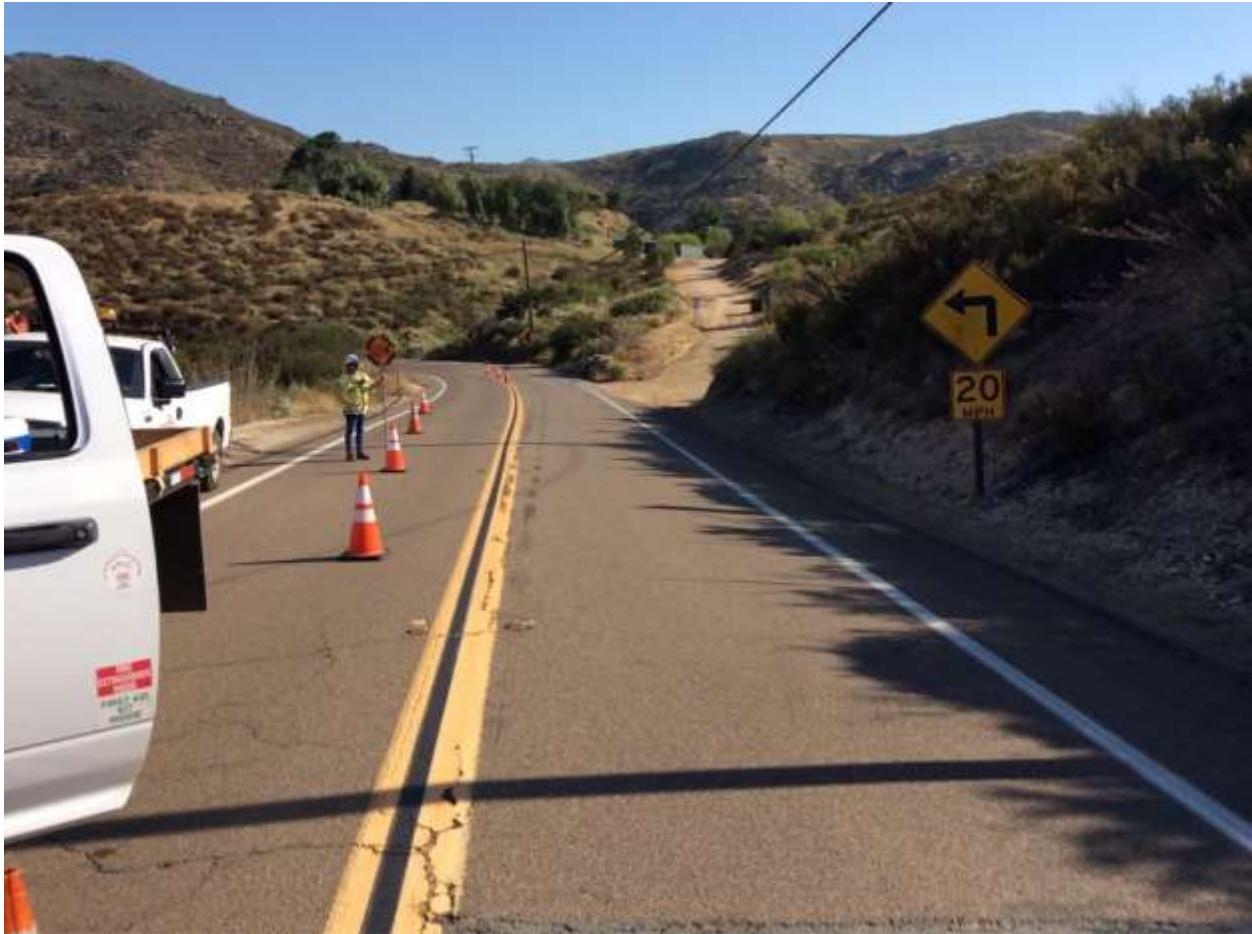
Photo 6: Traffic control flag persons were utilized to direct traffic on Japatul Road around construction equipment accessing a pole site along TL 625B in accordance with APM TRANS-02.
