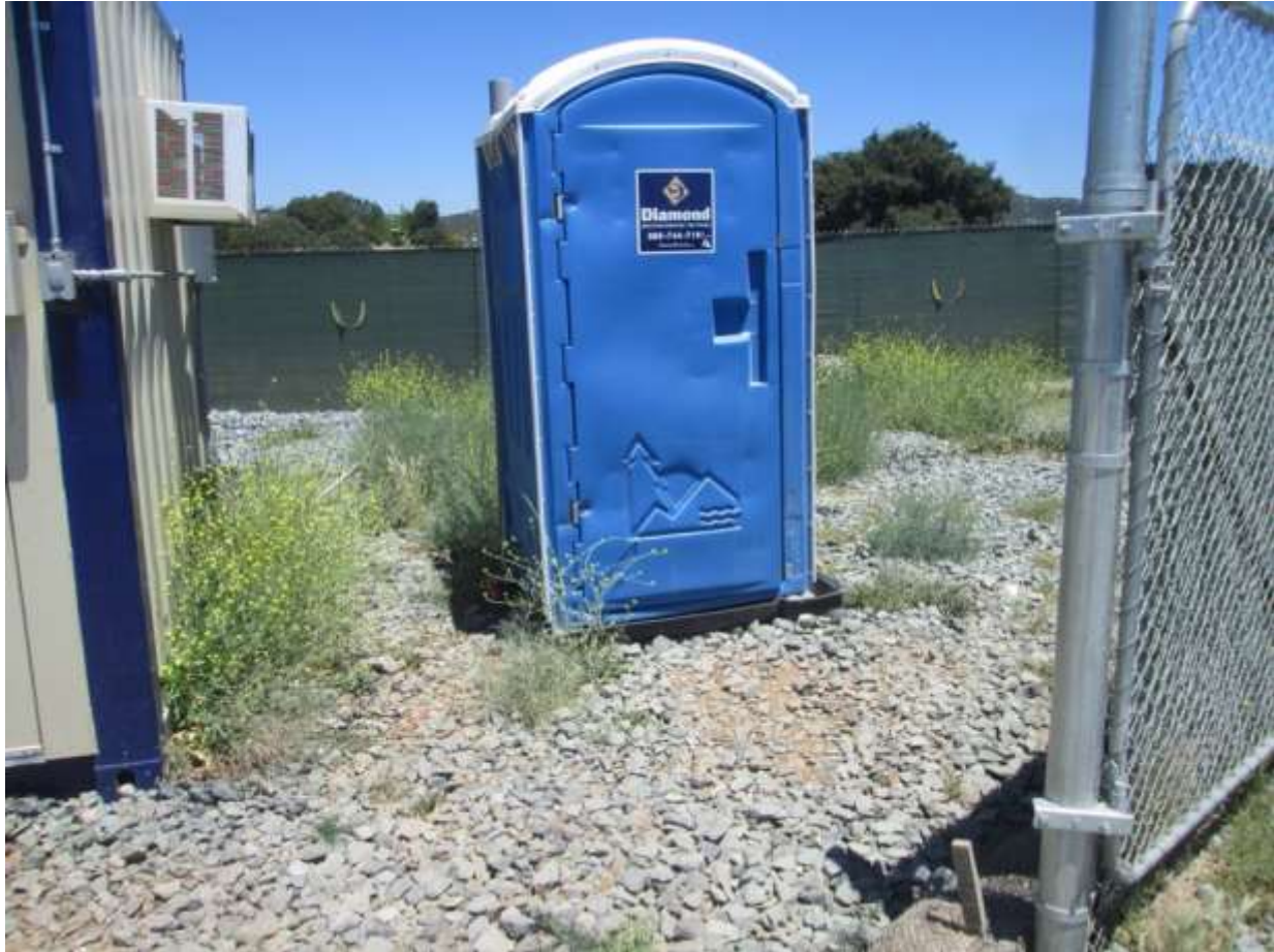
Photo 5: Secondary catchment observed beneath a portable restroom facility at the Japatul Spur Staging and Fly Yard in accordance with the project SWPPP.
