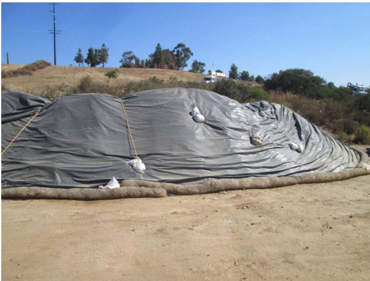
Photo 2: During PAR wire stringing at Pole Z135623 and Loveland Substation, erosion control BMPs were observed being implemented for a dirt stockpile and included the use of a cover and perimeter fiber rolls in accordance with the SWPPP (MM HYD-1 and APM HYD-09).
