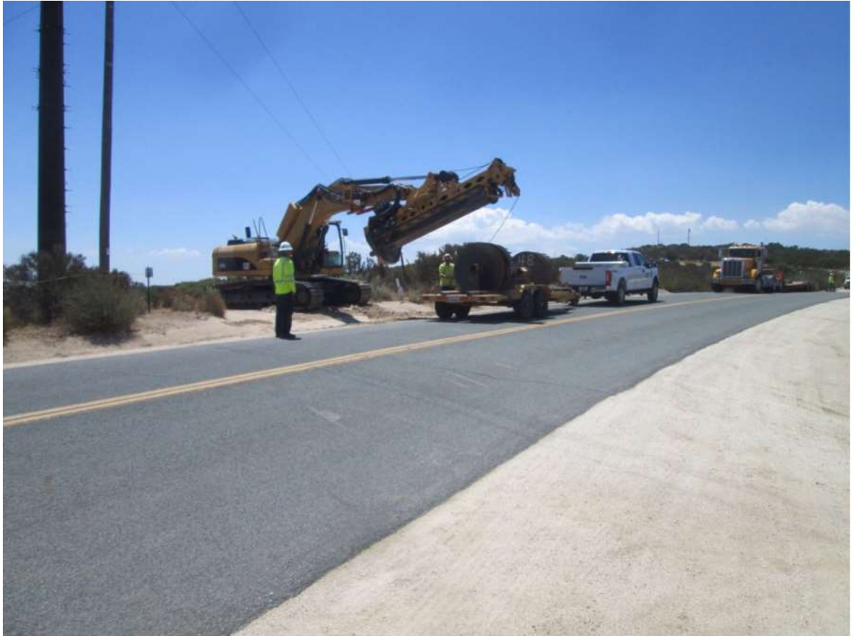
Photo 6: A construction crew was observed transporting a drill to the ROW at Pole Z44270. Traffic control flag persons were utilized along Tierra del Sol Road in accordance with APM TRANS-02.
