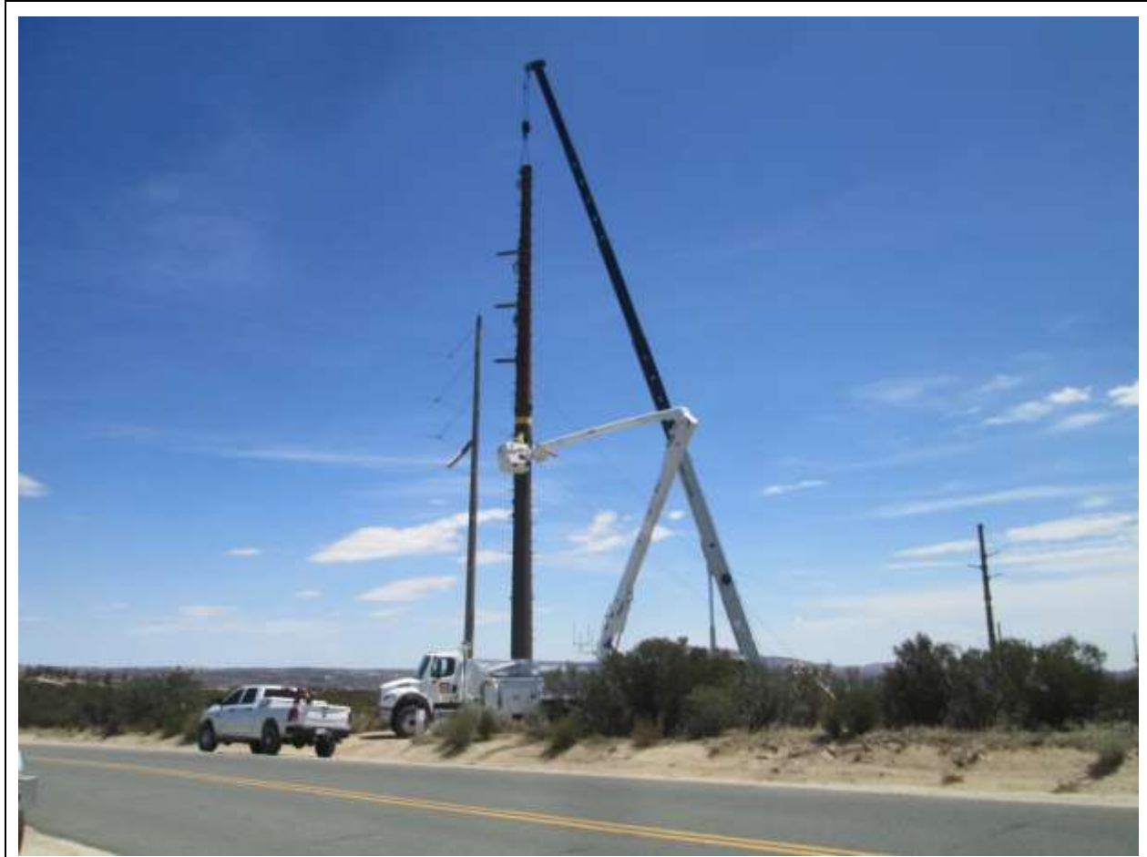
Photo 1: A construction crew observed installing a new pole at Pole Z44270 (TL 6931).
