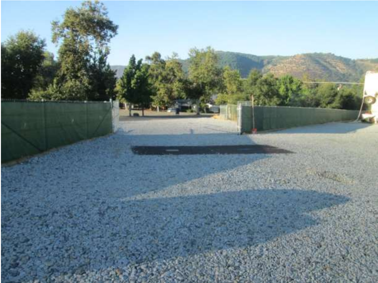
Photo 6: In accordance with the SWPPP (MM HYD-1, APM HYD-09, and MM BIO-7), rattle plates and gravel aggregate were installed at the ingress and egress of Orchard Staging Yard (TL 682) to prevent dirt/mud from being tracked onto public roadways. In accordance with APM VIS-02, opaque mesh material was installed around the perimeter of the yard as a visual screening measure.
