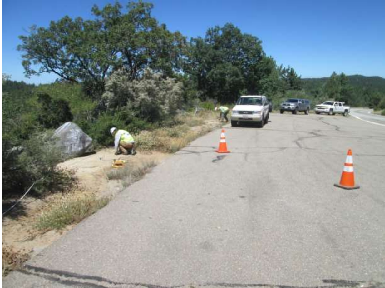
Photo 2: Seismic Refraction Testing observed being performed at seismic line S12 for the C 440 underground distribution line along Sunrise Highway.
