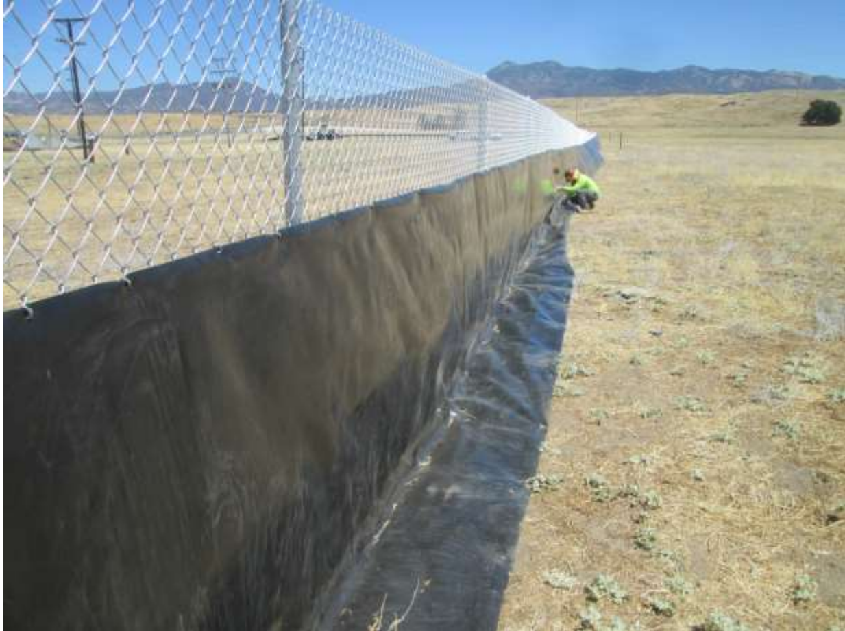
Photo 3: In accordance with MM BIO-31, a construction crew was observed installing Stephens' kangaroo rat exclusion barrier around the perimeter of Warner Substation Staging Yard (TL 682).
