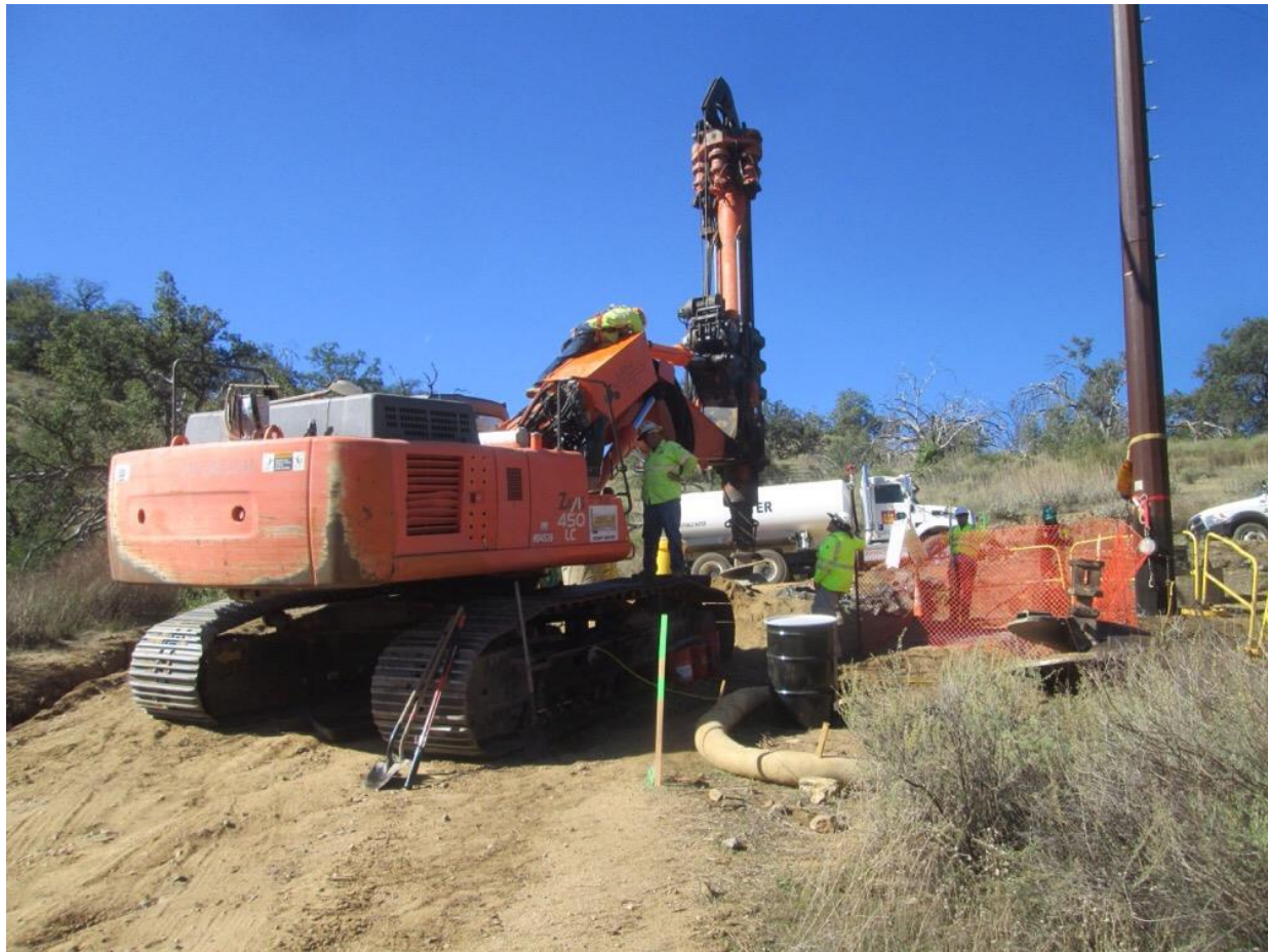
Photo 3: A drilling crew was observed repairing a hydraulic fluid leak on a drill rig and conducting stained soil cleanup. Absorbent pads and drip pans were observed being utilized, and stained soils were placed in a drum for disposal in accordance with the Spill Response and Notification Plan and MM-PHS-2.
