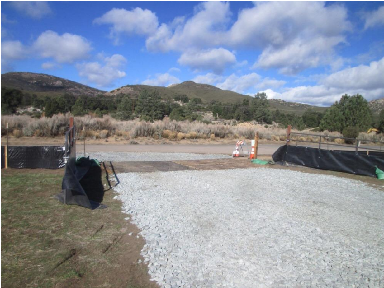
Photo 4: Track-out control BMPs, such as rattle plates and a rock apron were observed at the ingress and egress of Creekside Staging Yard in accordance with the SWPPP, Erosion Control Plan, MM-HYD-1, MM-BIO-7, and APM-HYD-09.
