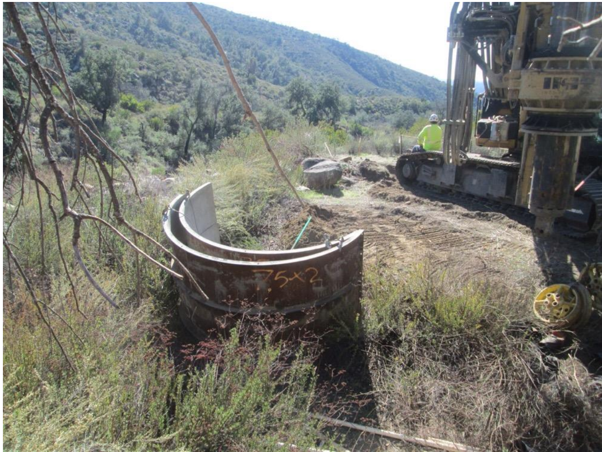
Photo 1: During drill site set up at Z118018 (TL 682), a foundation form was observed being staged approximately three feet outside of the delineated workspace. The LEI was notified, who contacted the crew foreman and had the form brought back inside the approved workspace (MM-BIO-1).
