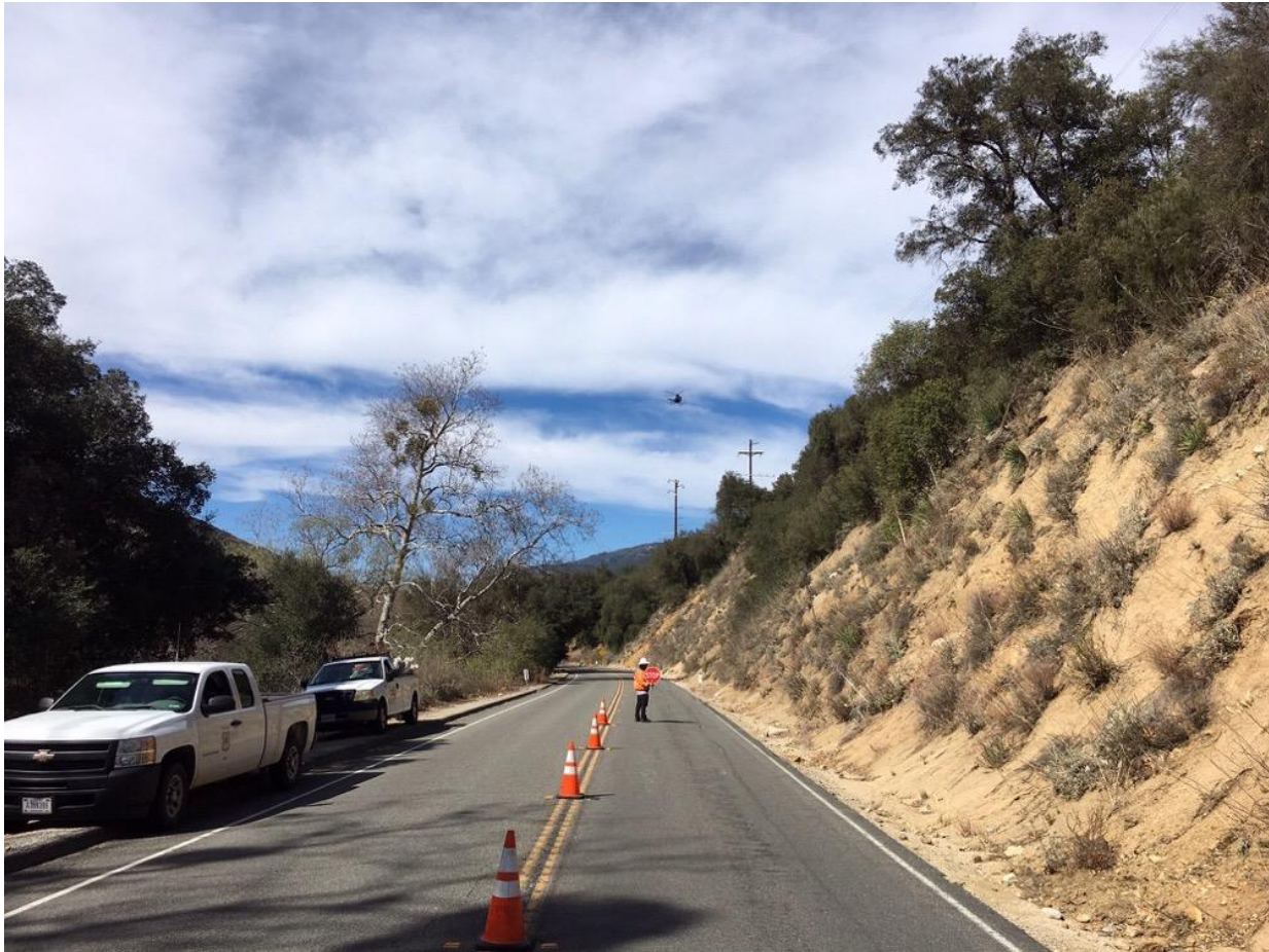
Photo 5: During steel pole installation with helicopter assistance, traffic control was setup in multiple locations along Highway 76 to temporarily stop traffic when work occurred adjacent to the highway in accordance with MM-TRANS-2.
