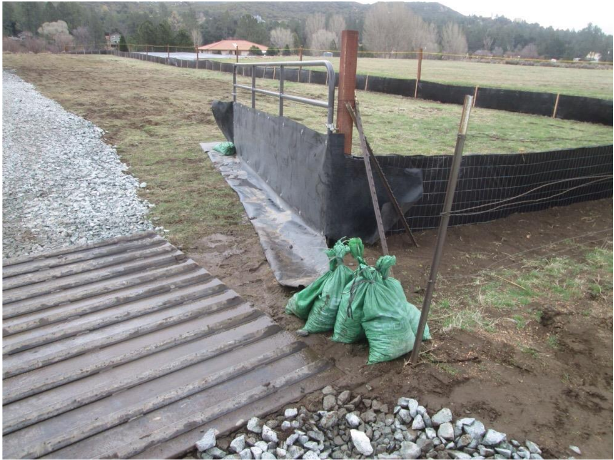
Photo 2: At the recommendation of the authorized biologist, arroyo toad protective measures for exclusionary purposes, such as the use of silt fencing around the yard and a rubber flap and gravel bags at the yard entrance, were observed being implemented at Creekside Staging Yard (Section 2.11 - Streambed Alteration Agreement).
