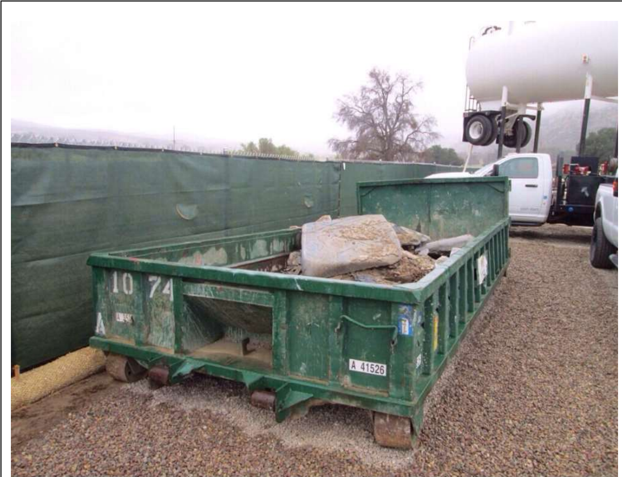
Photo 3: Concrete was disposed in designated waste bins at the Kitchen Creek Staging Yard in accordance with the SWPPP (APM HYD-05, MM BIO-7, and MM HYD-1).
