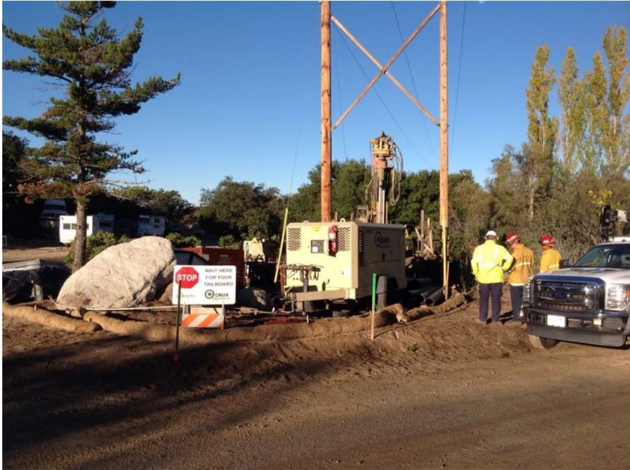
Photo 4: A dedicated fire patrol was present at Pole Z44210 for welding activities and remained on site for one hour after welding was complete. The surrounding area was regularly wet down, all required fire tools were present per the appendix in the CFPPP (MM FF-1).
