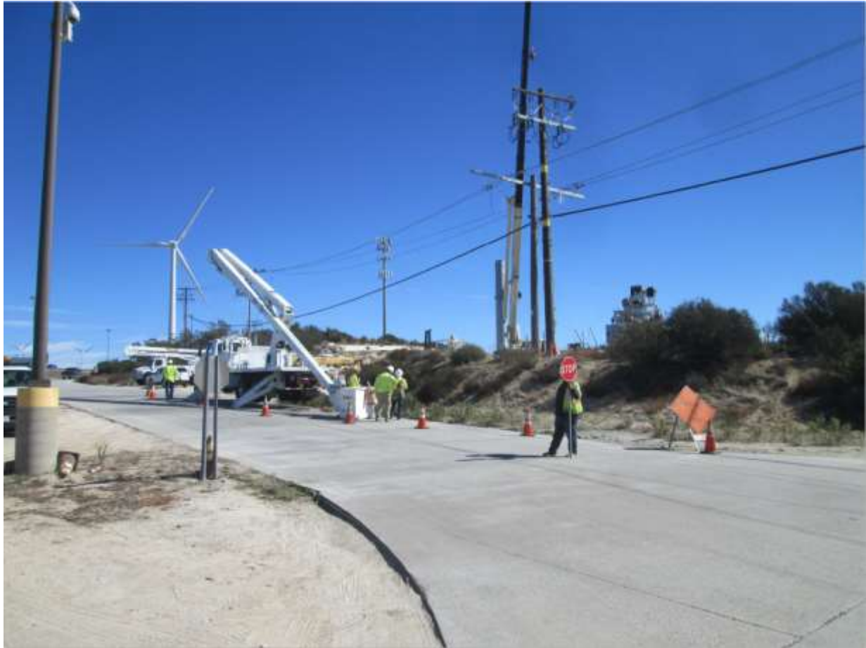
Photo 5: Traffic notification/safety signage was observed along Old Highway 80 in accordance with the Project's TCP (APM-TRANS-05) and APM-TRANS-02 during steel pole installation and transferring of conduit to a new steel pole at P174081.
