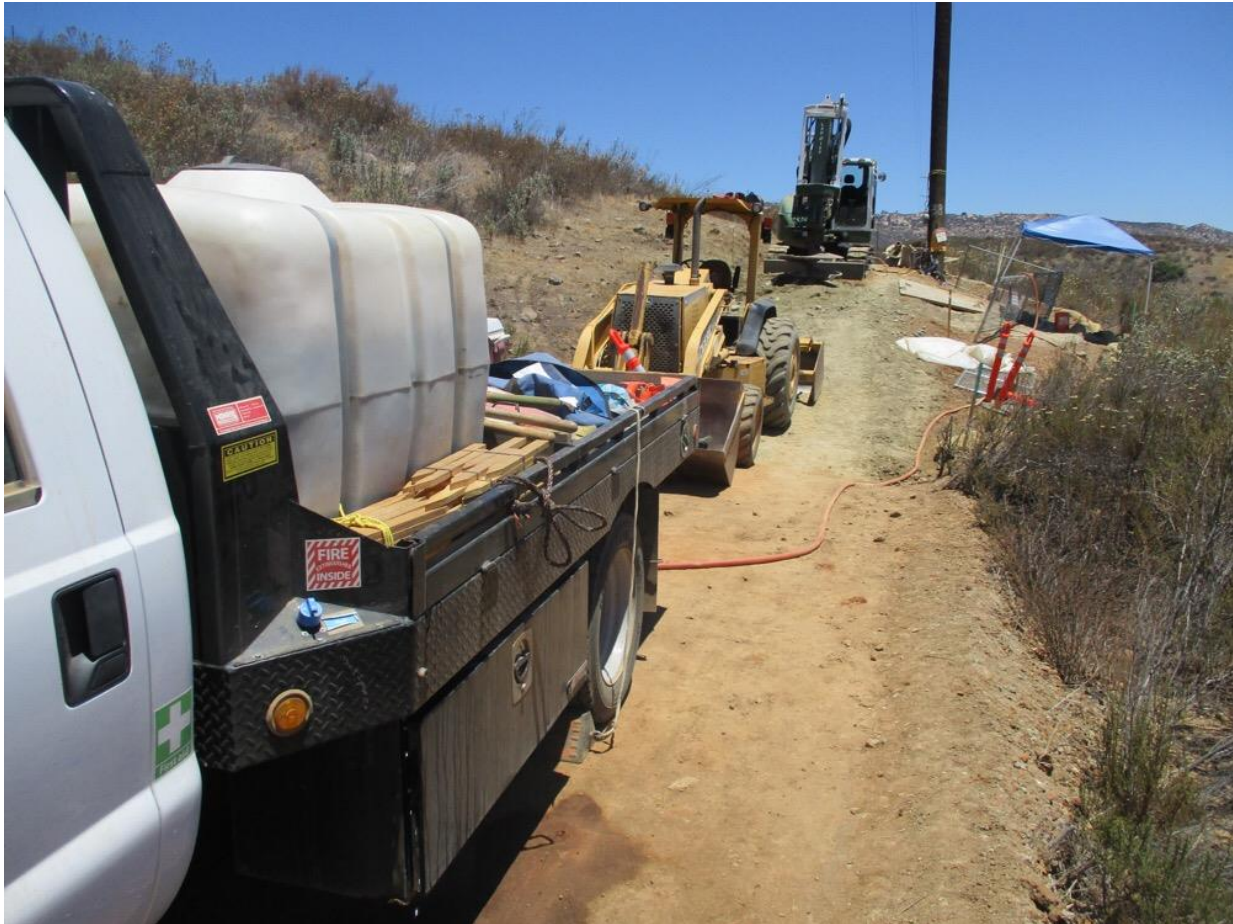
Photo 6: During grounding installation at Z571447 (TL6957), a truck-mounted water tank with over 150 gallons of water, including a pump and a hose, was observed on-site (in addition to the standard required fire tools) to satisfy CFPPP fire prevention matrix requirements for trenching work off CNF land with an elevated FPI
