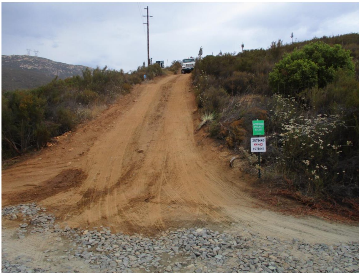
Photo 2: During pole hole drilling at Z571441 (TL 6957), crews were observed using approved access roads (marked with signage) in accordance with MM BIO-1.
