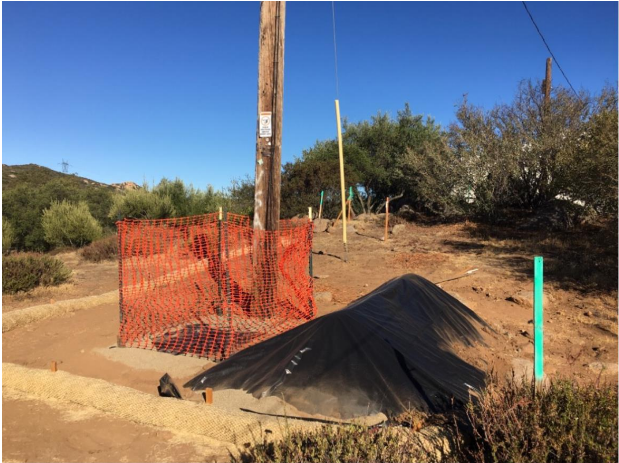
Photo 4: Hand-digging that occurred at pole P971138 (TL 6957) during the previous work day was observed completed. To prevent wildlife entrapment per MM BIO-23, the hole was covered and fenced and spoils were covered with black visqueen to prevent erosion in accordance with the Erosion Control Plan (ECP) and the SWPPP (MM HYD-1, MM BIO-7). Straw wattles installed around the site were observed in good condition.
