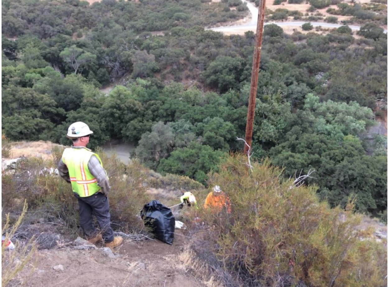
Photo 3: A Biological Monitor was present during vegetation removal at Pole Z118090 (TL 682) in accordance with MM BIO-3.
