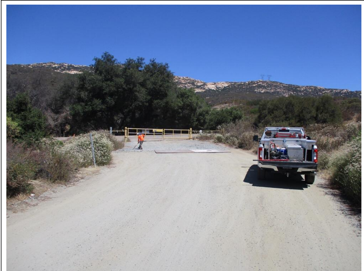
Photo 1: To prevent sediment trackout onto Lyons Valley Road a worker was observed maintaining the rock apron and clearing debris from the rattle plate installed at the ingress/egress point to the Swat Yard, in accordance with the Erosion Control Plan and SWPPP (MM HYD-1, MM BIO-7). Track-out was not observed (APM AIR-05).
