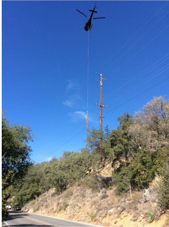
Photo 5: During old wooden pole removal at Pole Z118109 (TL 682), helicopter external load operations were observed being utilized in accordance with the ASP and MM PHS-5.
