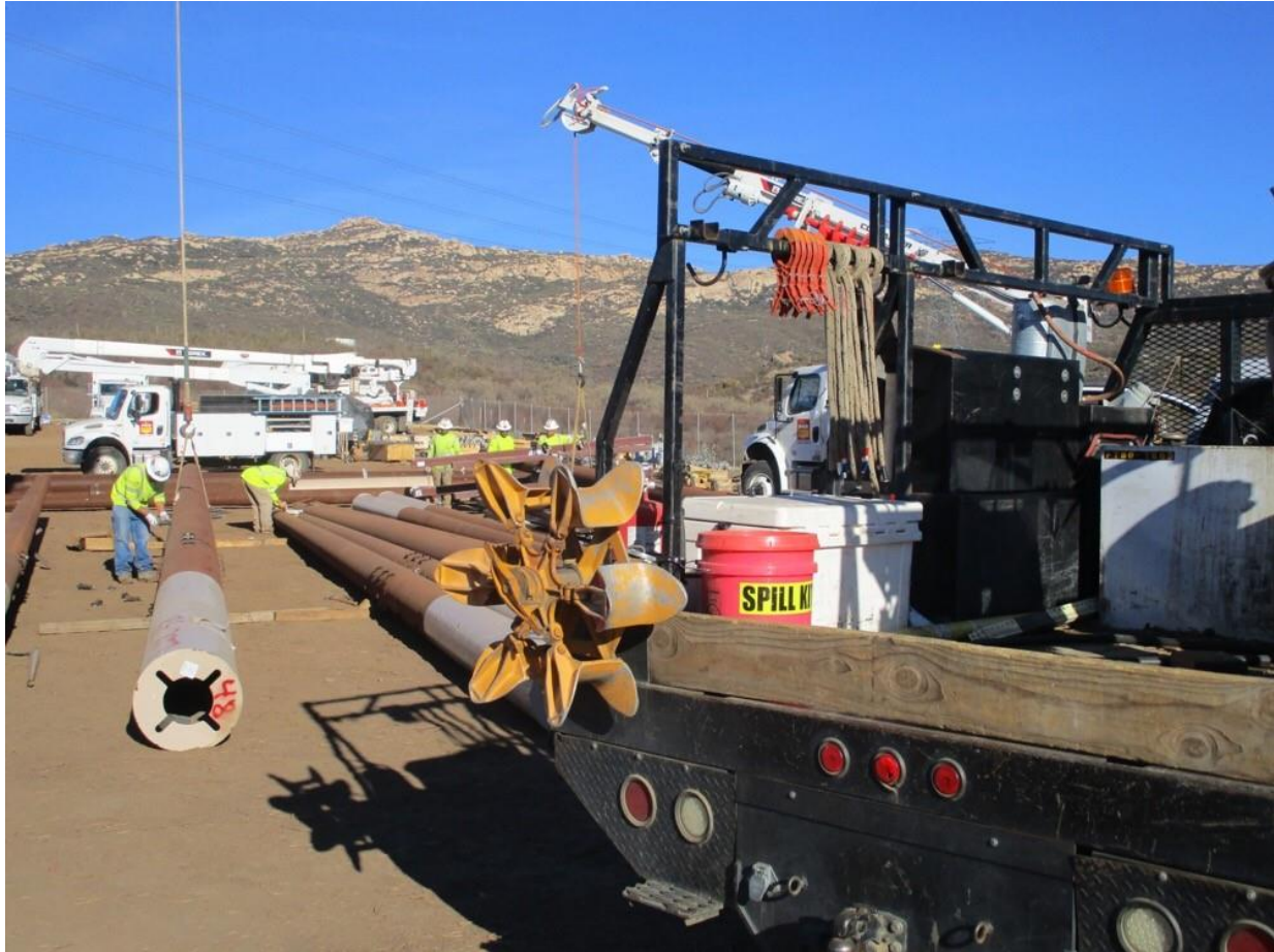
Photo 6: During pole assembly and framing at Swat Staging Yard (C 157), a spill kit was observed in a crew truck for potential spill cleanups in accordance with the SRNP and MM PHS-2.
