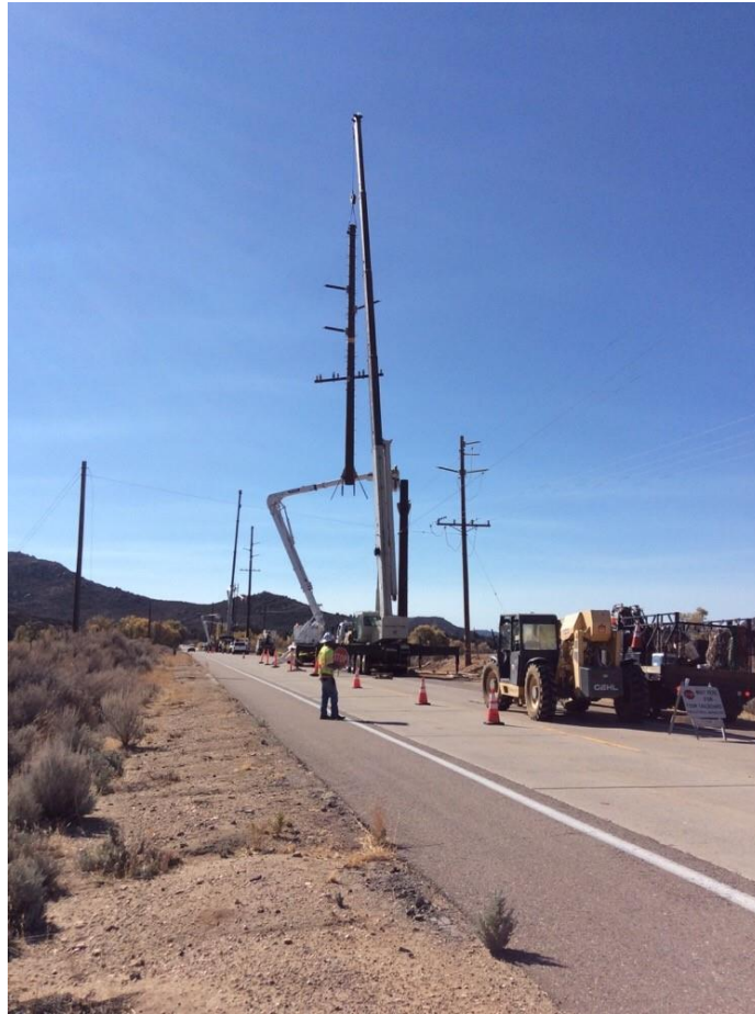
Photo 4: During pole installation at Pole Z40553 (TL 629C), traffic control personnel were observed safely flagging motorists around equipment staged within the south bound lane of Old Highway 80 in accordance with APM TRANS-02.
