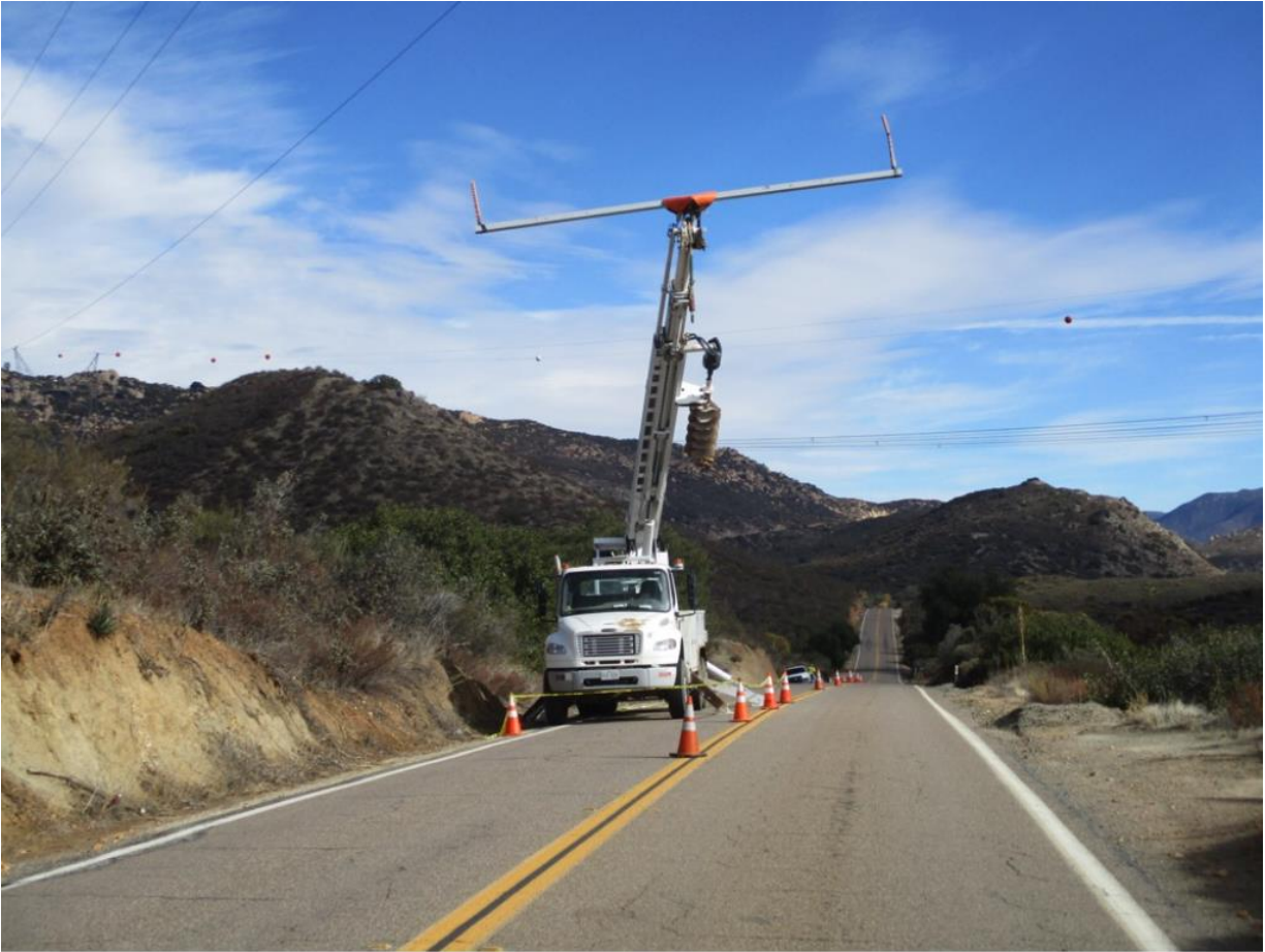
Photo 6: In accordance with APM TRANS-02, Pro Traffic flaggers closed one lane of Lyons Valley Road to allow the staging of a PAR guard structure during fiber optic stringing between Z571432 and Z571451 (TL 6957).
