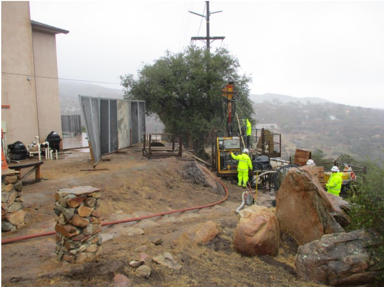
Photo 5: A noise barrier was observed being utilized at Z571469 (TL 6957) in accordance with MM NOI-1 and equipment was observed positioned as far away from the house as possible in accordance with APM NOI-02.
