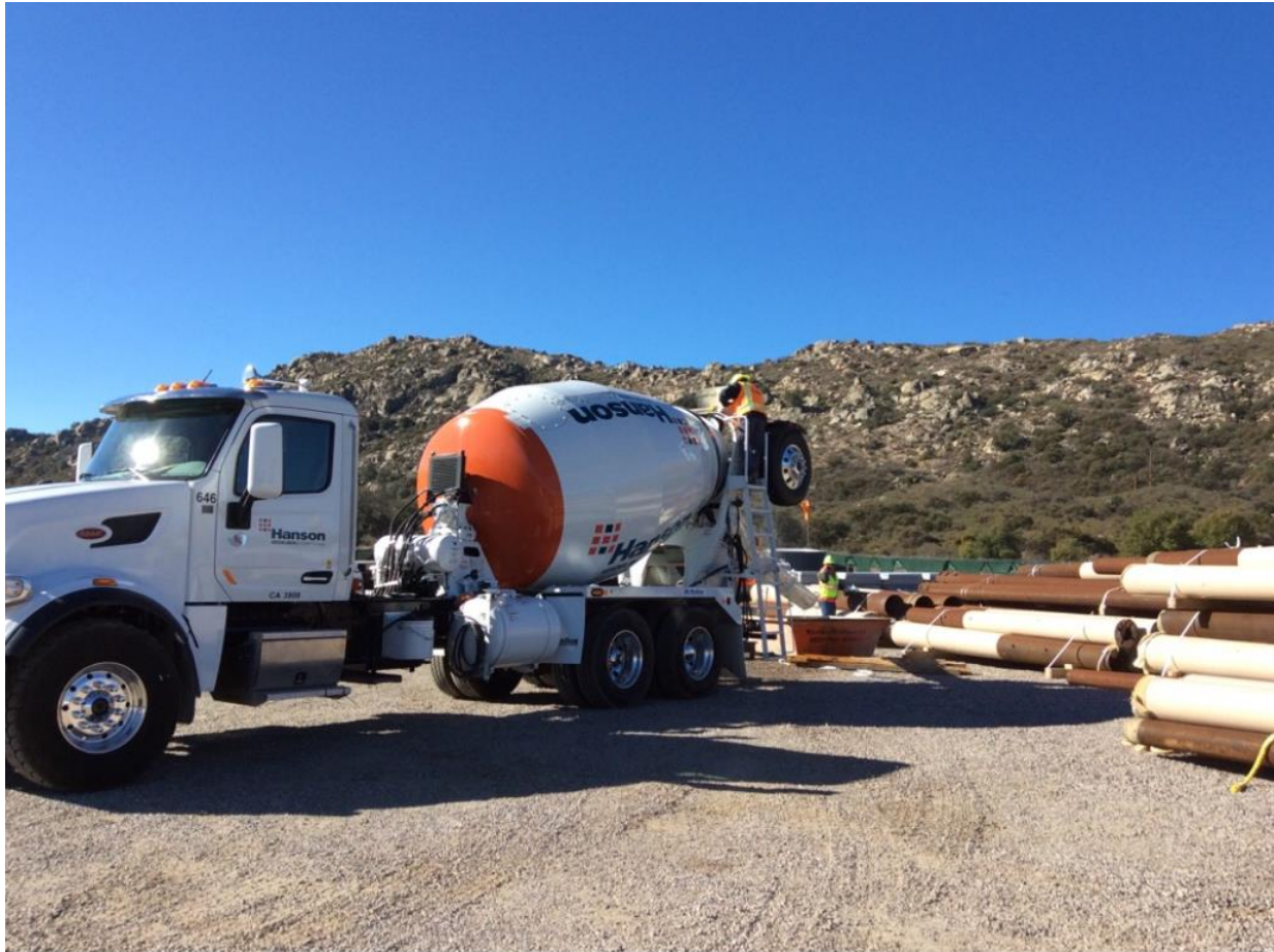
Photo 4: In accordance with APM HYD-01, concrete washout was observed to be taking place at a designated concrete washout station at Kitchen Creek Staging Yard.
