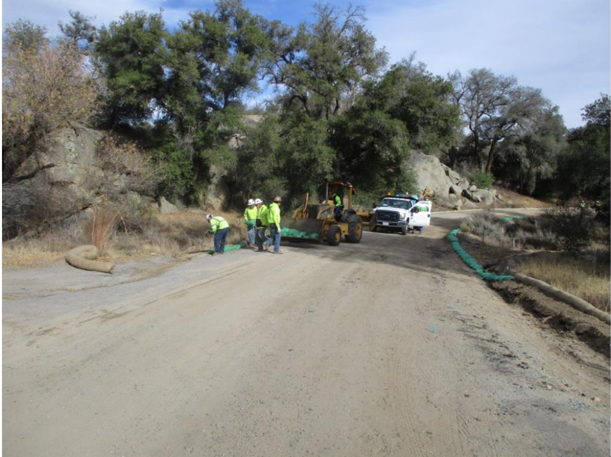
Photo 3: Crews were observed trenching for the installation of silt fence, installing fiber rolls, and installing gravel bag berms along a drainage swale/area of higher velocity flow along Morena Stokes Valley Road in accordance with the ECP, SWPPP (MM HYD-1, MM BIO-7) and APM-HYD-09.
