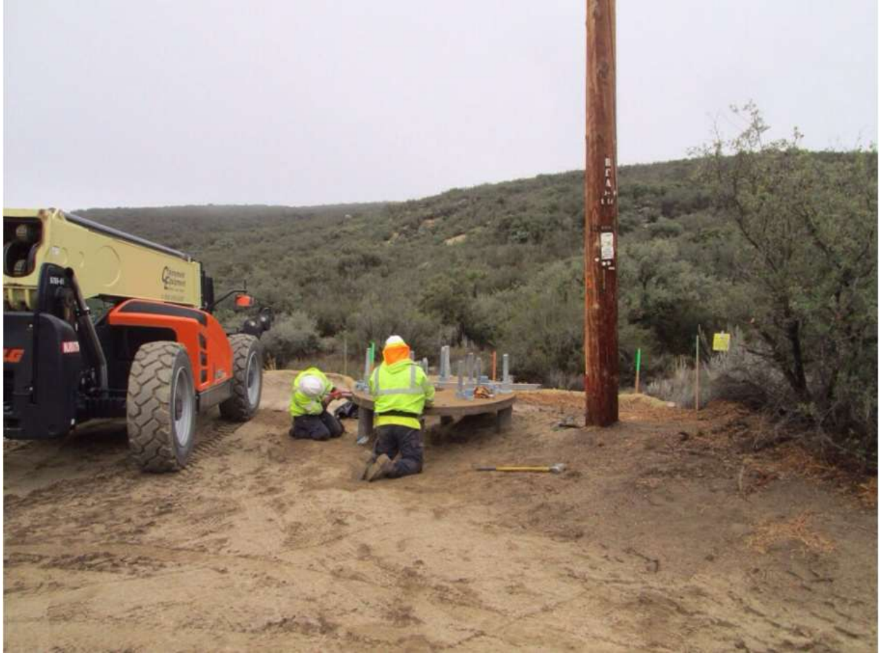
Photo 3: Construction crews were observed installing the micro pile foundation caps at pole sites. All observed work occurred within the delineated work limits in accordance with MM BIO-1 and ESAs were marked and avoided.
