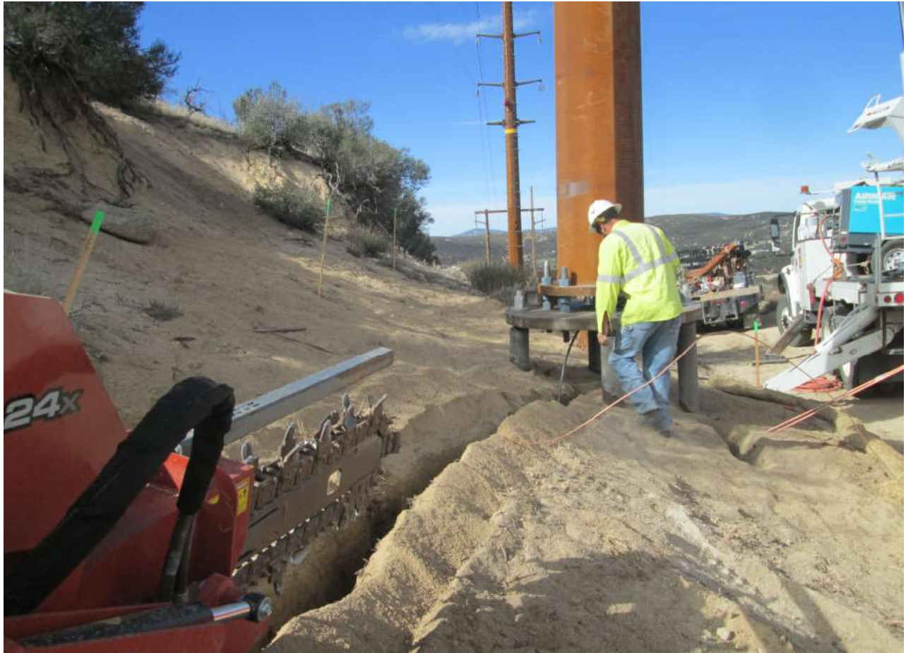
Photo 4: Crews were observed installing ground wire within delineated work limits (MM BIO-1) at new steel structures along TL 629E.
