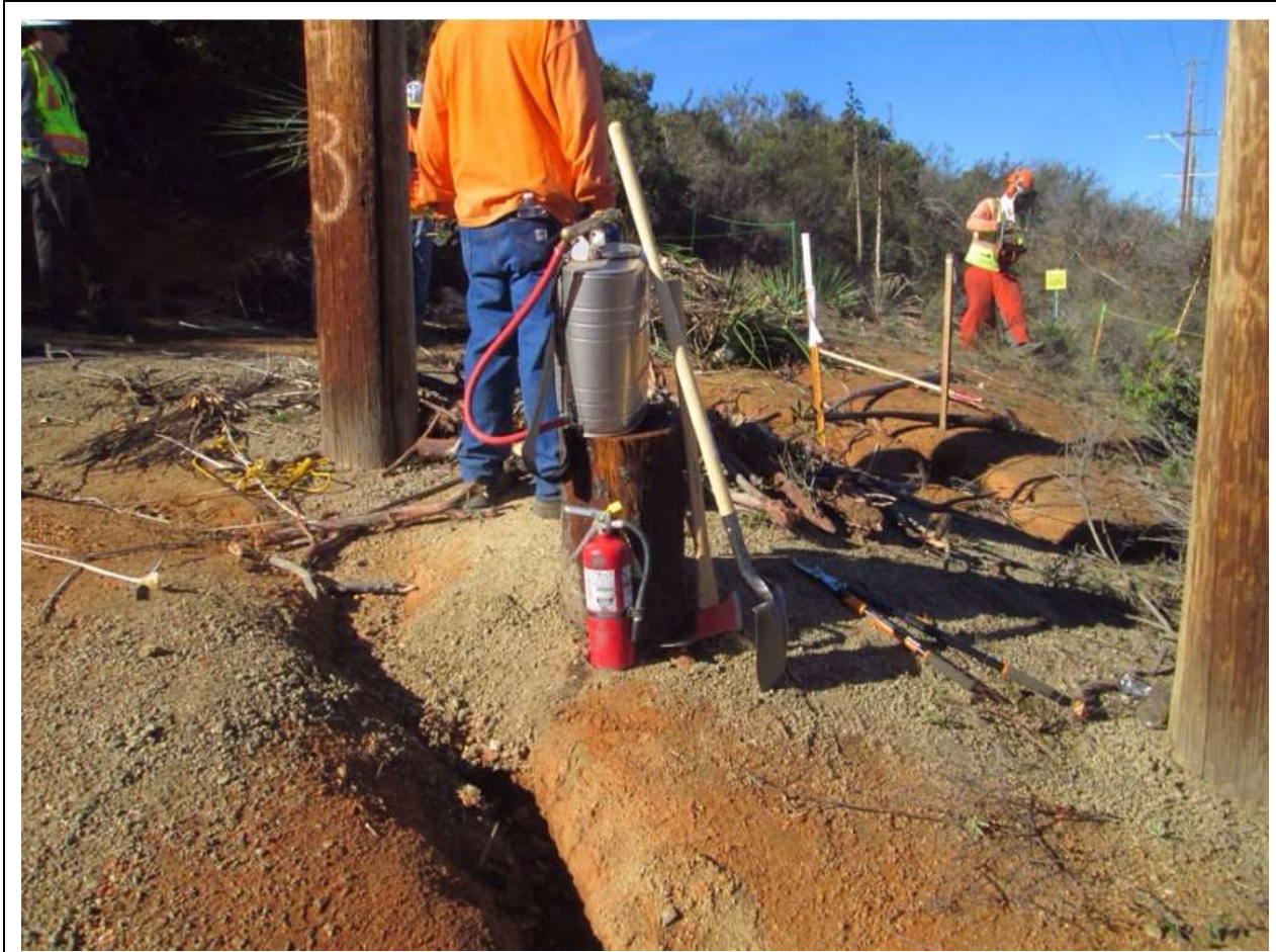
Photo 1: A 5 gallon backpack pump, round point shovel, Pulaski, and 2A10BC fire extinguisher were observed staged on site during vegetation chipping along TL 625B in accordance with the Fire Prevention Matrix in the CFPPP.
