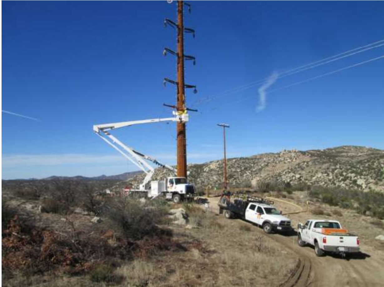
Photo 5: Construction crews were observed transferring wire to travelers along TL 629E. Previously installed SWPPP BMPs were observed in tact at developed micro pile sites (MM HYD-1).
