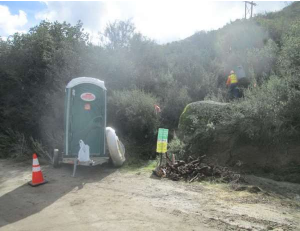
Photo 2: Approved access routes (footpaths) for sites inaccessible by vehicles (TL 625B, pole Z272893, above) were marked prior to vegetation clearing and adhered to in accordance with MM BIO-1. Crews were observed carrying in trash bins to transport removed vegetation via foot.
