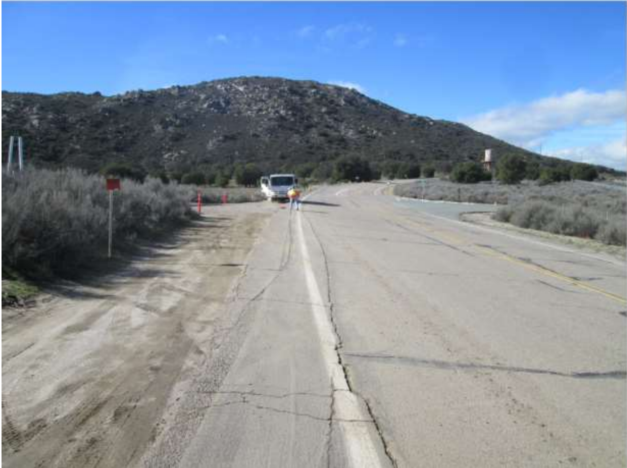
Photo 5: Crews were observed sweeping sediment track-out at the intersection of the Kitchen Creek Staging Yard and Old Highway 80 in accordance with APM AIR-05 and the project SWPPP.
