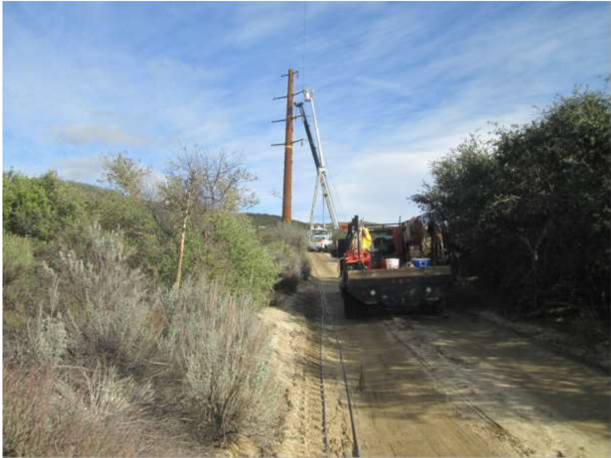
Photo 4: Wire stinging activities occurred along TL629E (transferring wire at Pole Z44186, above).
