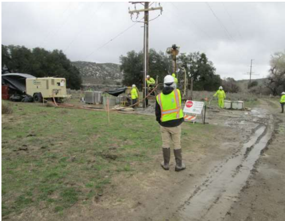
Photo 6: Biological monitors were observed at micropile foundation work areas (TL 629E, Pole Z40582, above) in accordance with MM BIO-22. Where roads were determined too saturated for vehicles, crews walked to sites to prevent rutting and erosion on existing access roads.
