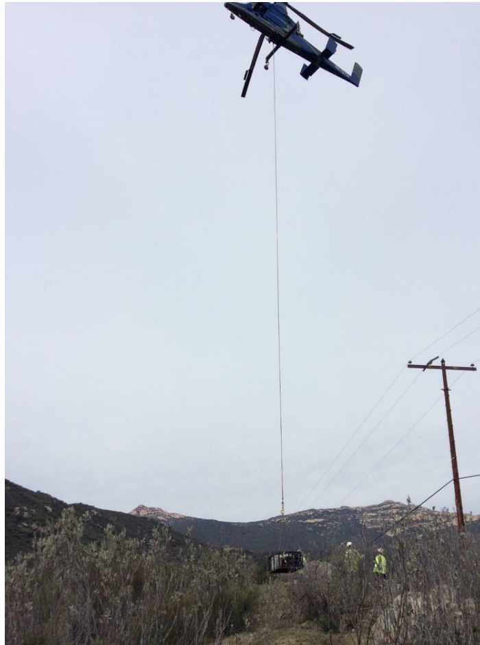
Photo 5: Helicopter external load operations were used to demobilize equipment and remove spoils piles from Pole P278719 (C 157).
