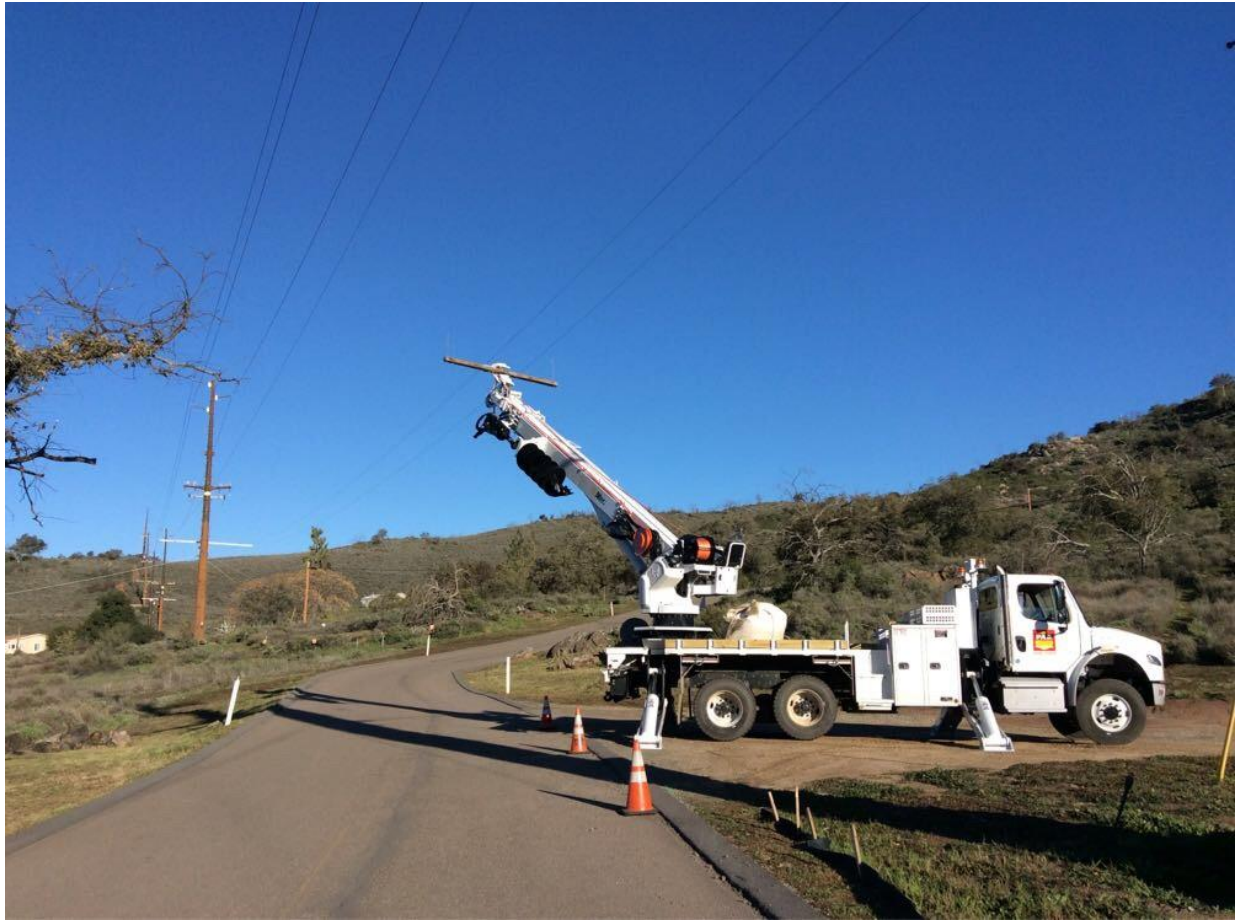
Photo 4: A temporary guard structure was observed near Pole Z118073 (TL 682) to protect the road from wire that may sag during the pulling process.
