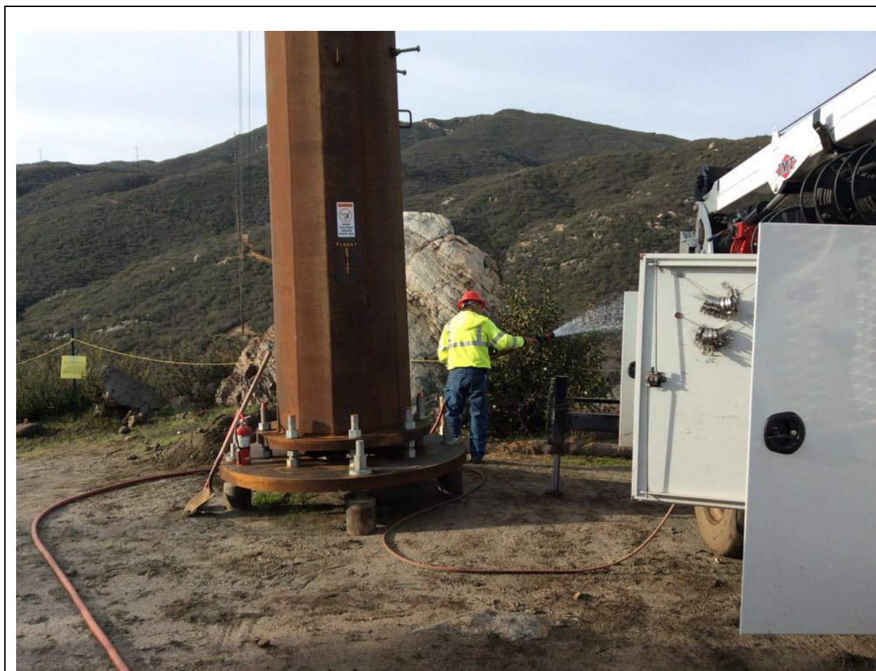
Photo 2: A dedicated fire patrol was observed wetting down surrounding vegetation prior to the commencement of hot work at Pole Z571453 (TL 6957), in accordance with the CFPPP Fire Matrix.
