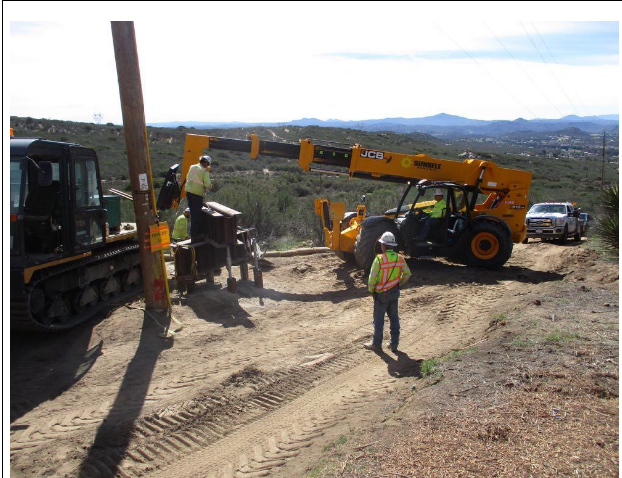
Photo 3: A construction crew was observed removing steel beams used for micropile foundation proof testing at Z40997 (TL 6958).
