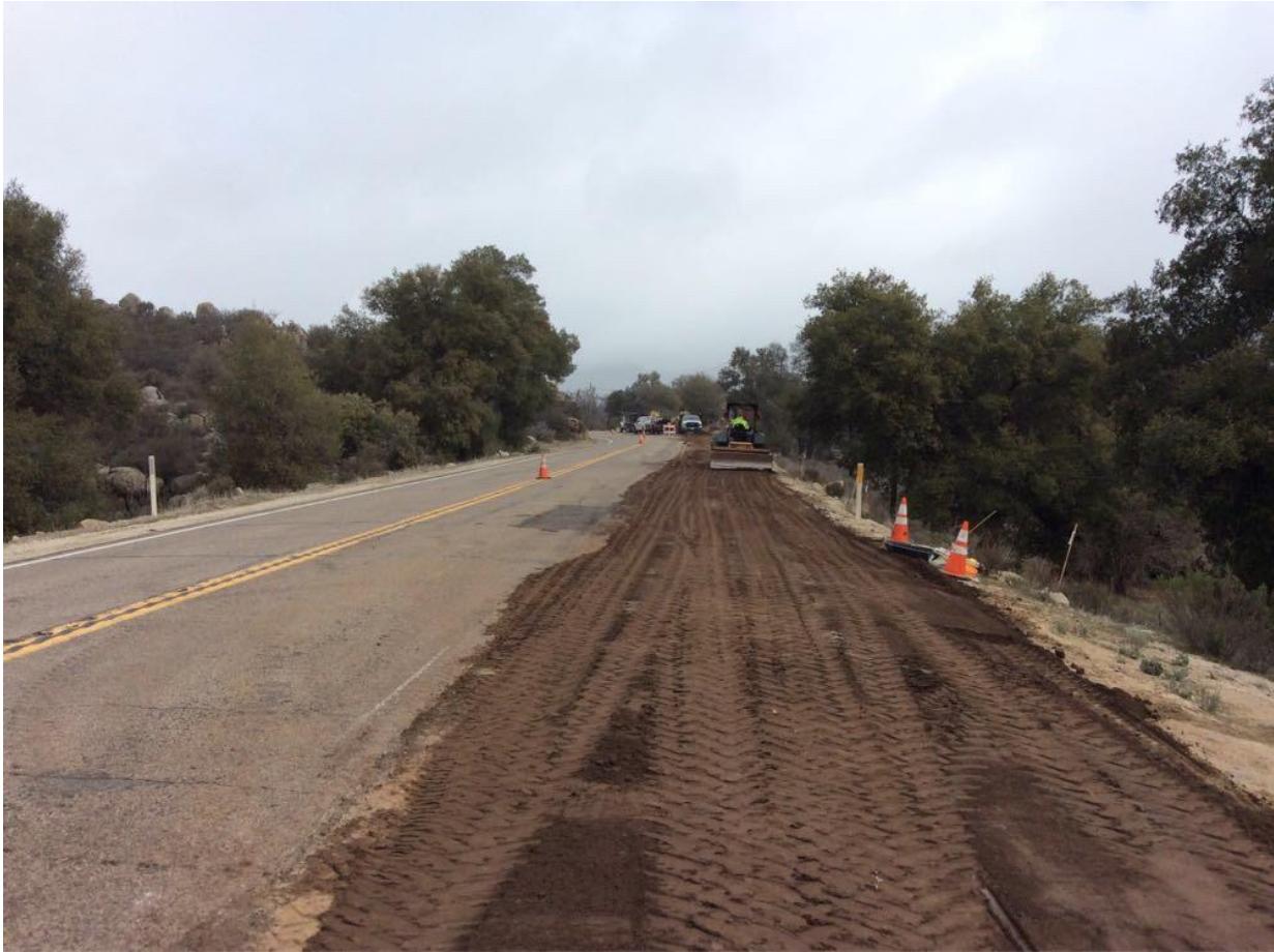
Photo 6: A construction crew was observed backfilling and grading along Buckman Springs Road following trenching and underground installation.
