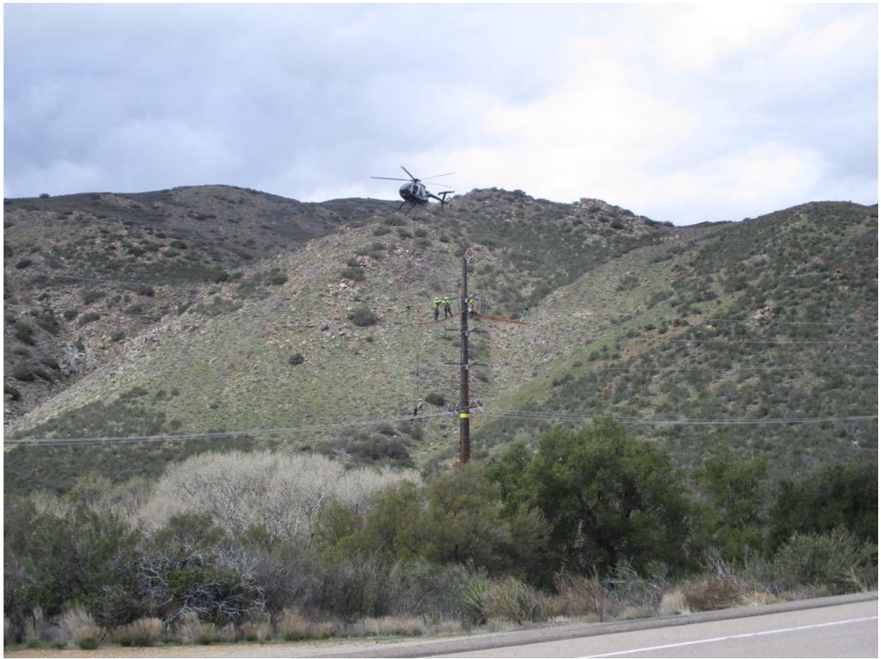
Photo 1: A construction crew was observed conducting human external cargo operations to assist with dead ending the 69 kV line at Z40509 (TL 629C).
