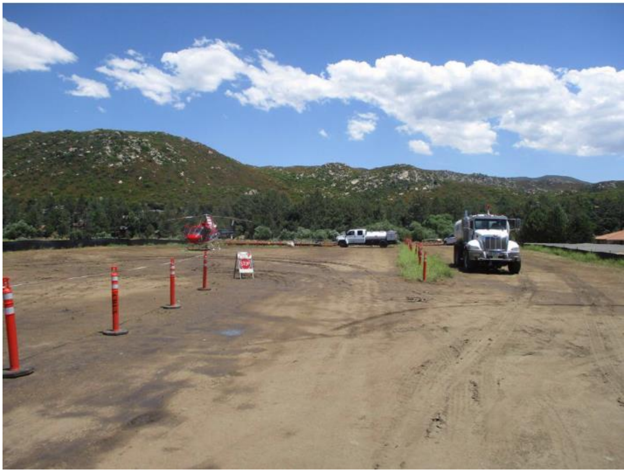
Photo 1: Helicopter activities supporting Geo Pacific brushing work at Z173122 (TL 629A) was observed being conducted out of Creekside Staging and Fly Yard. A water truck watered the designated and delineated helicopter landing area to prevent dust emissions in accordance with the Aviation Safety Plan (MM PHS-5) and APM AIR-02.
