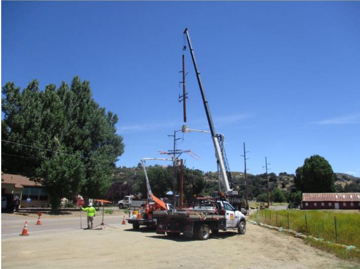
Photo 6: A crew was observed directing traffic along Viejas Boulevard while setting a pole top at Z373147 (TL 629A) in accordance with the TCP (APM TRANS-05).
