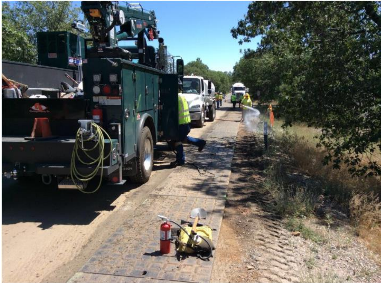
Photo 5: A dedicated fire patrol was observed wetting down the area near 439+50 (C 440) prior to hot work (welding), and a complete set of fire tools was observed within 50 feet of the activity in accordance with the CFPPP for the day's fire conditions (PAL C on CNF land).
