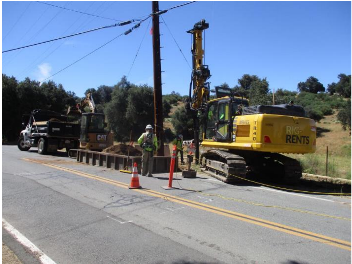
Photo 2: A crew was observed drilling a pole foundation hole at Z163042 (TL 629A), and exporting dirt spoil off-site. The haul truck exporting dirt spoil utilized a load cover to prevent dust in accordance with APM AIR-02.
