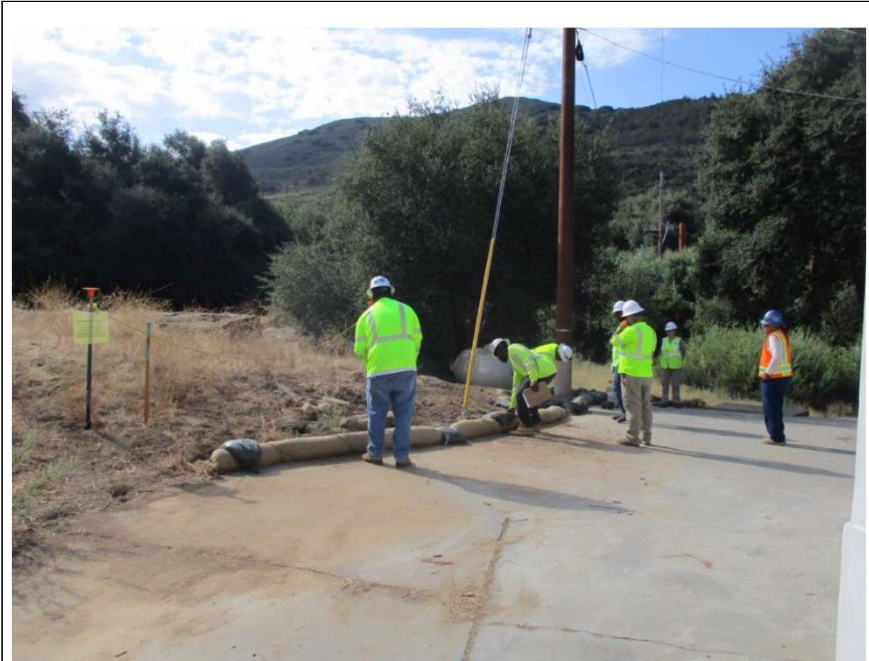
Photo 2: During fiber roll installation at TL 629A, two cultural monitors were present, a cultural resources ESA was delineated along the eastern perimeter of the work space, and gravel bags were used to weigh down the fiber rolls instead them being dug into the ground in accordance with the HPMP (MM CUL-1), APM CUL-03, and APM CUL-04.
