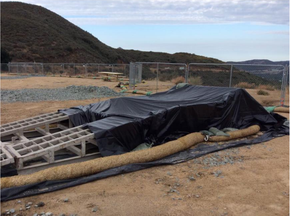
Photo 6: The concrete washout bin at Staging Area 2A (C 440) was observed to be covered in preparation for forecasted rain in accordance with the SWPPP.
