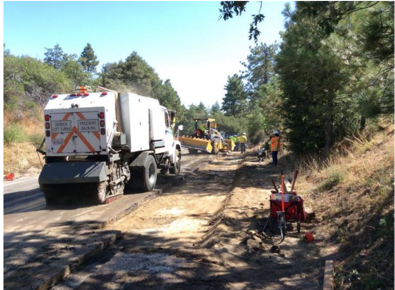
Photo 5: A street sweeping machine was observed cleaning up debris associated with asphalt removal near 406+50 (C 440) in accordance with the SWPPP.
