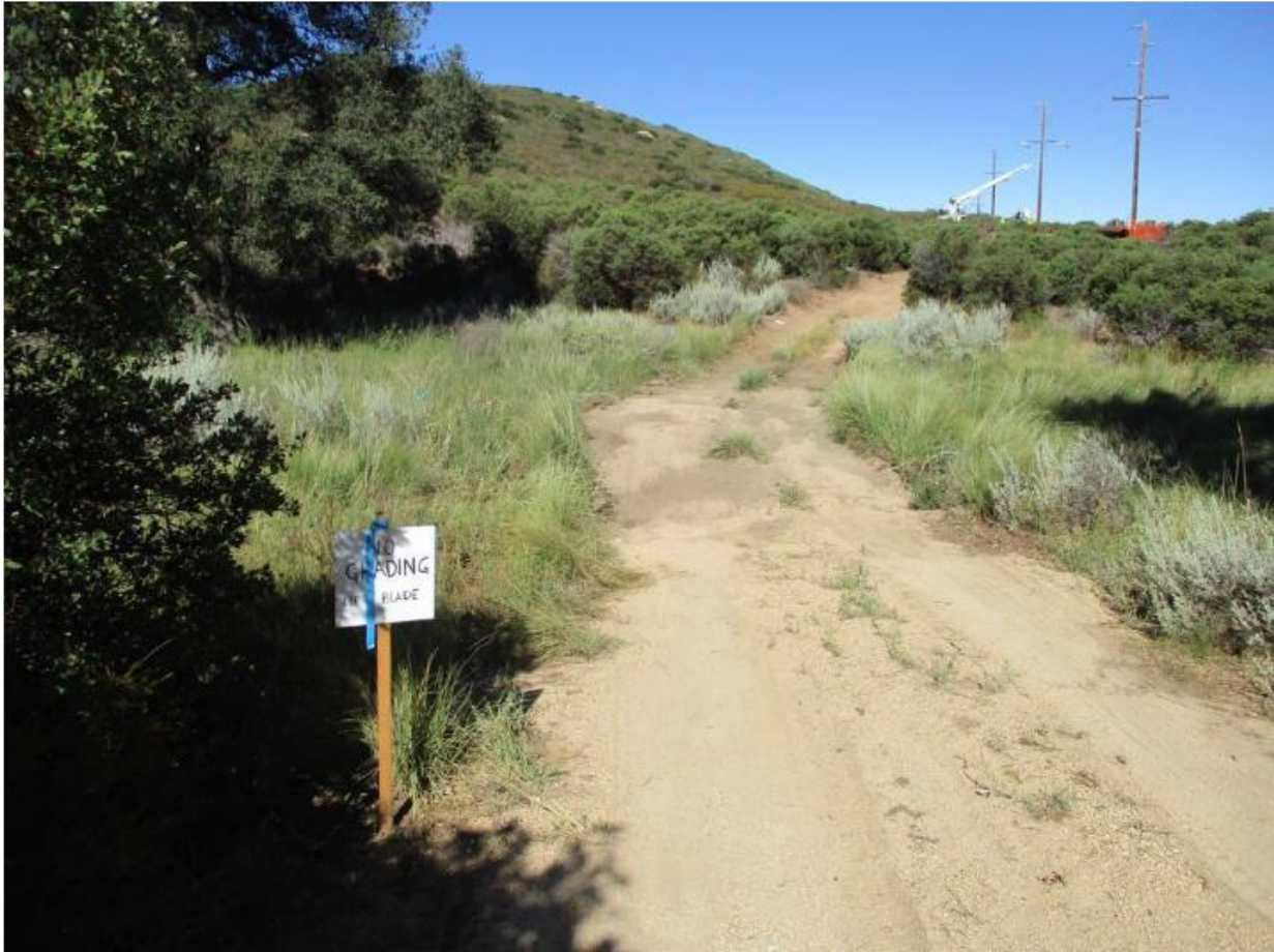
Photo 4: During pole setting at Z276641 (TL 629A), a hydrological resource was observed flagged along the approved road to the site, and a sign stating 'no grading, lift blade' was posted to minimize impacts to the stream in accordance with APM HYD-06.
