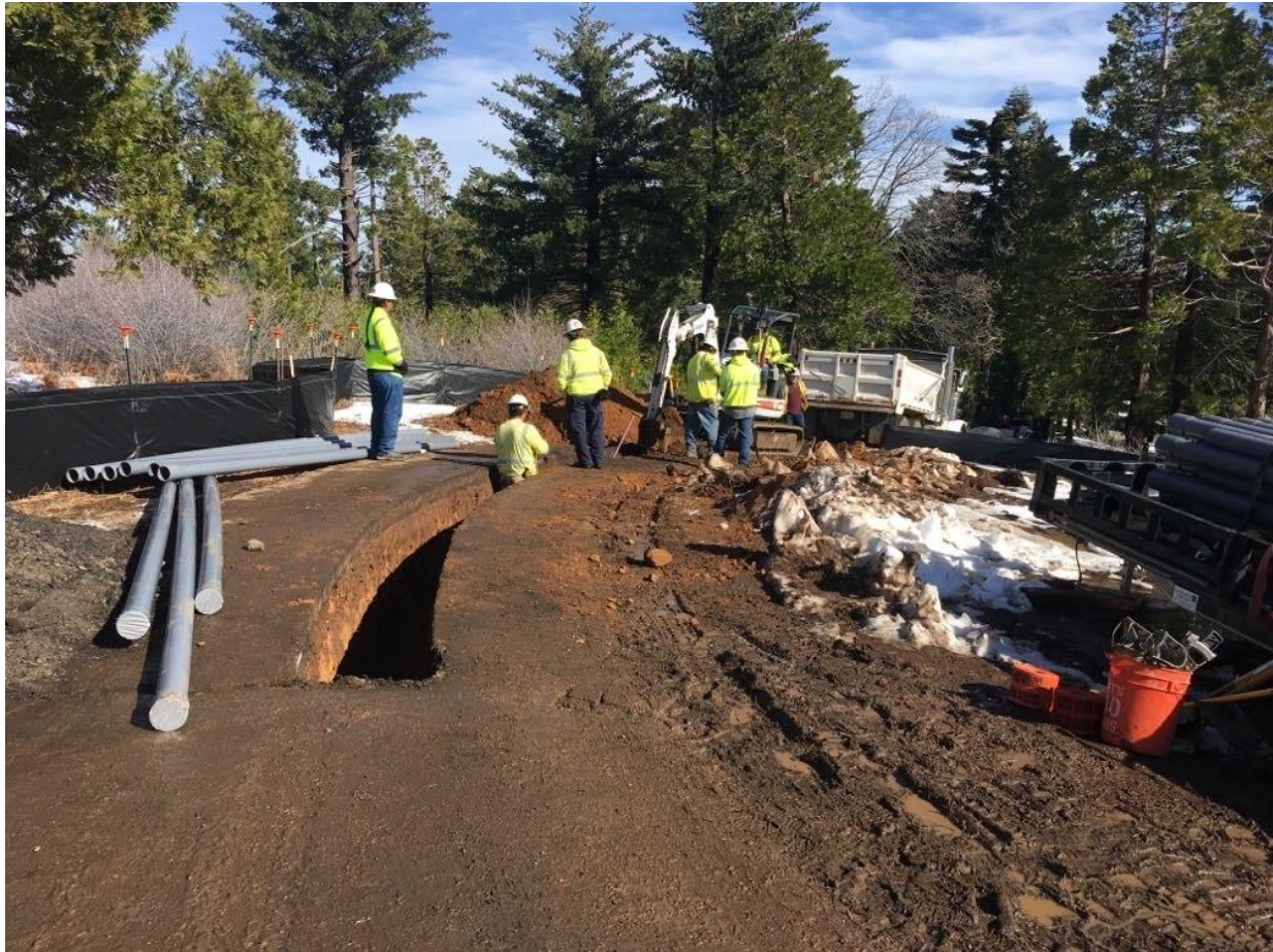
Photo 3: Along C 79A near station 36+00, during trenching, soil export, and conduit installation, cultural monitors were observed inspecting excavated soils and viewing trench sidewalls to prevent unauthorized impacts to potentially buried cultural resources in accordance with the HPMP, MM CUL-1, and APM CUL-04.
