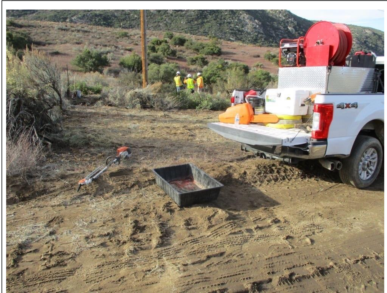
Photo 4: To prevent leaks and spills from being discharged into the soil during vegetation clearing work at Pole Z46583 (TL 6923), the construction crew refueled equipment over a drip pan in accordance with the SNRP and MM PHS-2.
