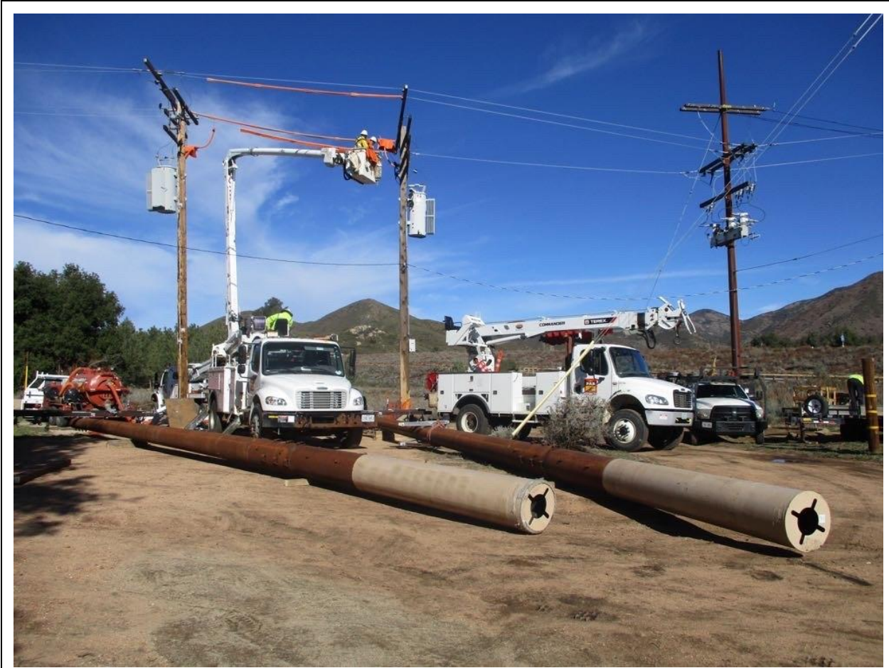
Photo 1: A line crew observed conducting overhead wire work and installing wire protectors in preparation for pole setting at Poles P164041 and P164042 along TL 629A.
