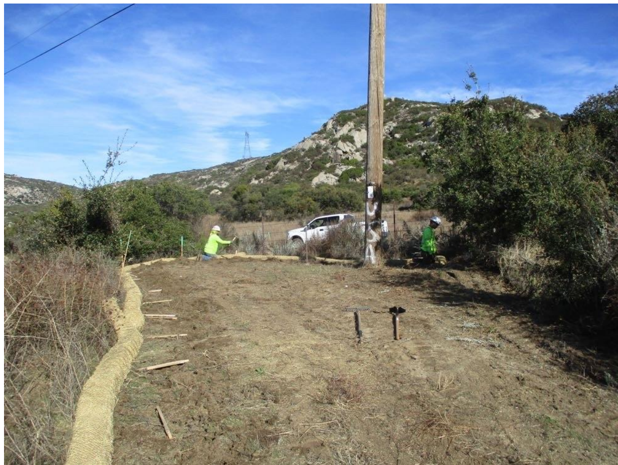
Photo 5: A construction crew observed installing straw wattles for erosion and sediment control around the workspace perimeter at Pole Z46583 (TL 6923) in accordance with the ECP and SWPPP.
