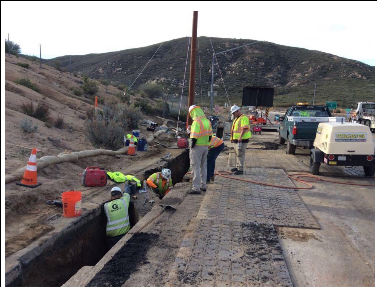
Photo 2: While construction crews installed conduit package near Vault 1 along C 440, a biological monitor was observed inspecting the site to ensure compliance with MMs, APMS, and permit conditions in accordance with MM BIO-22.
