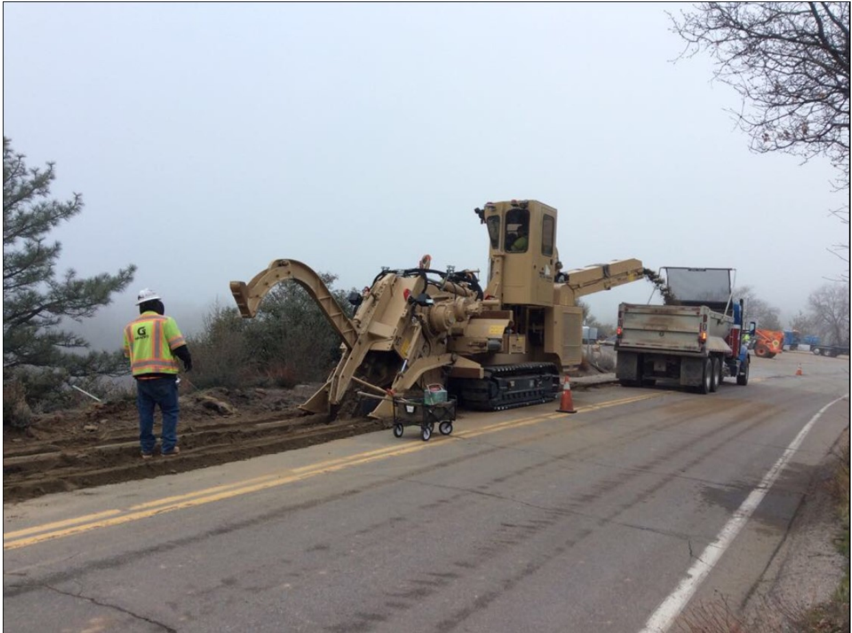
Photo 5: During excavation along C 440 Phase I, a complete set of fire tools per the CFPPP (MM FF-1) was observed on site.
