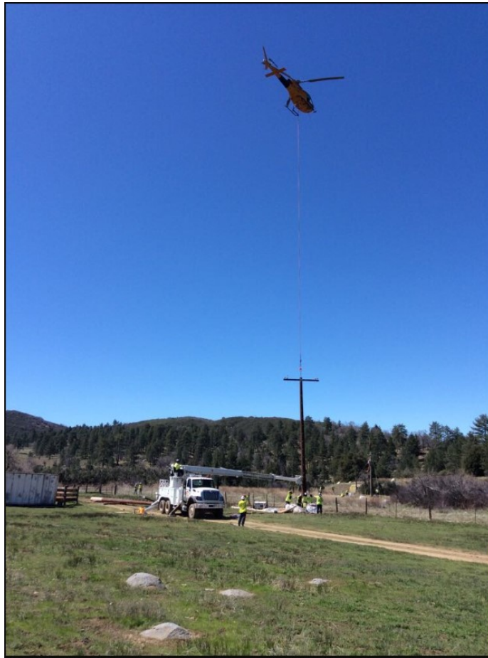
Photo 1: A crew was observed using helicopter external load operations to set P258404 (C 440 Phase I). The associated line truck was observed on the approved access road in accordance with MM BIO-1.
