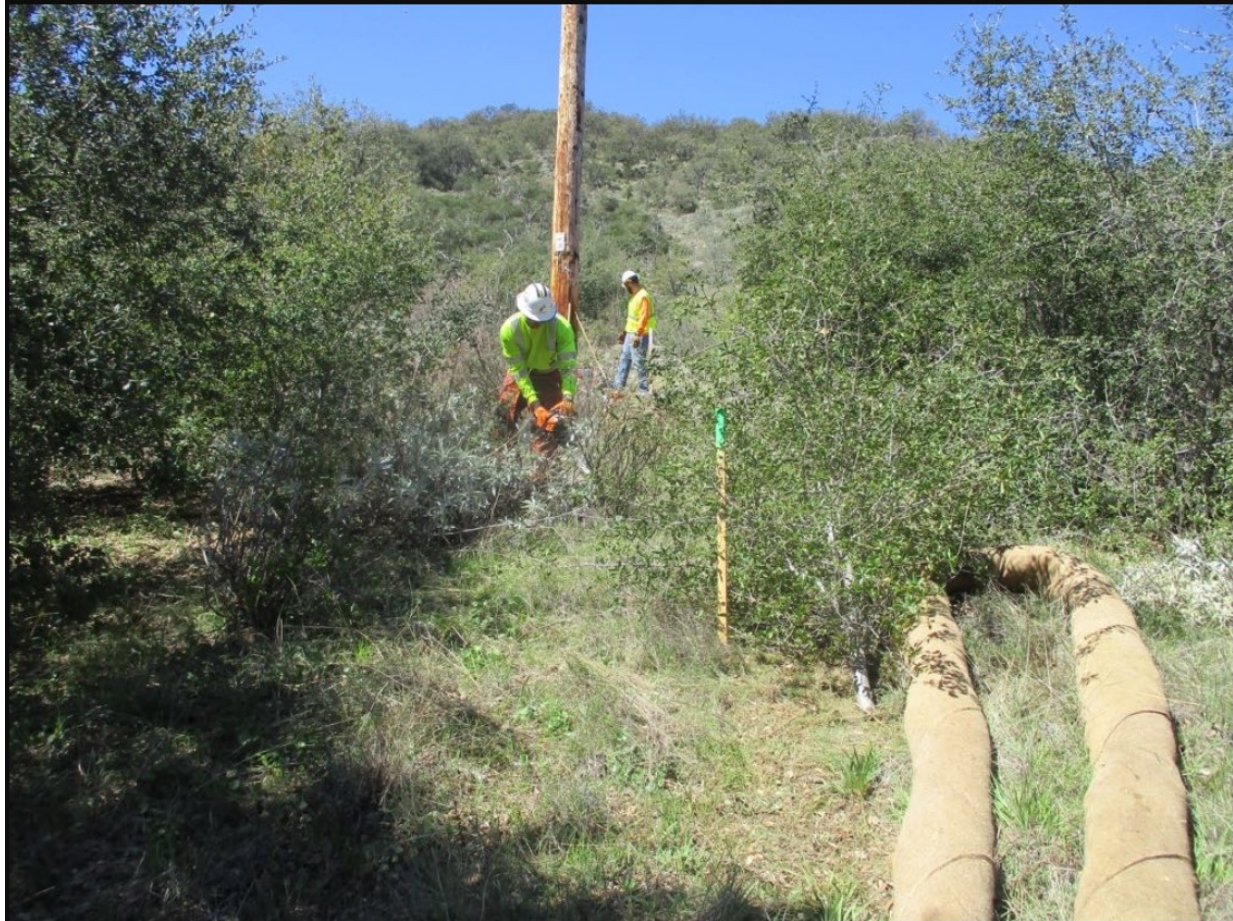
Photo 2: Vegetation clearing crews at P259357 (TL 626 Conversion North/C 222) were observed avoiding Engelmann oak within the work space in accordance with MM BIO-13 and MM BIO-14, and a biological monitor was observed on site during vegetation clearing in accordance with MM BIO-3.
