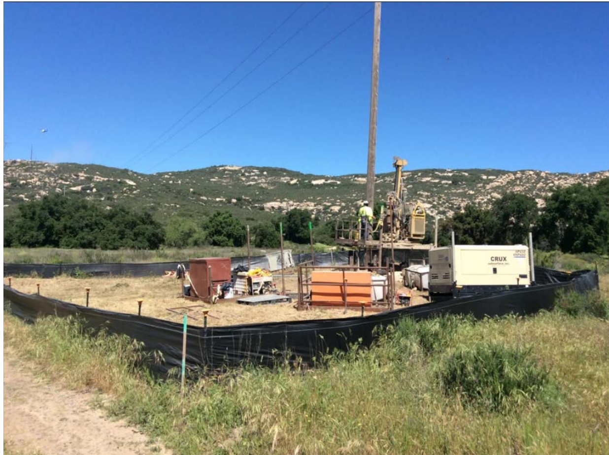
Photo 2: A crew was observed demobilizing drilling equipment and preparing it for transport from Z972842 (TL 6923). Exclusion fencing for arroyo toad observed in good condition in accordance with project requirements.
