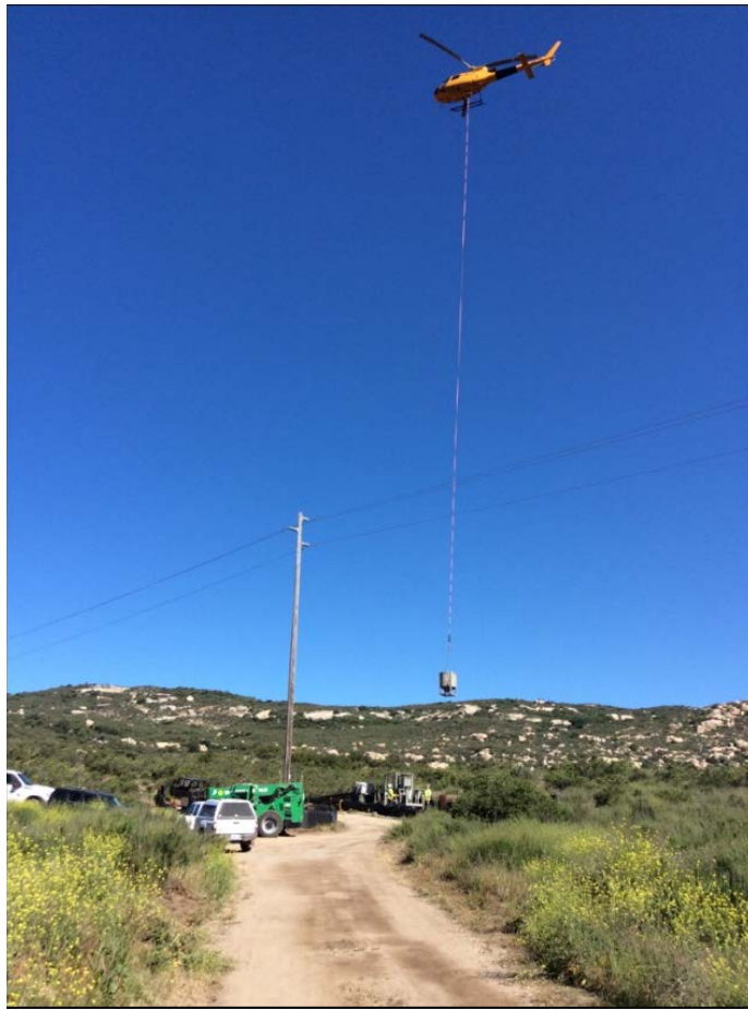
Photo 1: A crew was observed using helicopter external load operations in support of pressure grouting at Z972840 (TL 6923). Vehicles and equipment were observed to be staged on approved access roads in accordance with MM BIO-1.
