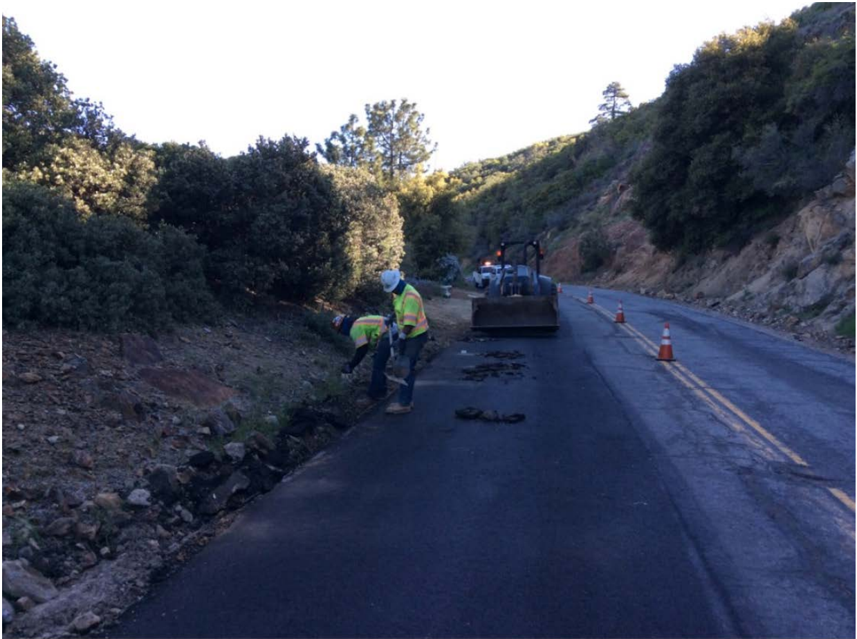
Photo 6: A crew was observed conducting cleanup and punch-list activities near 200+00 (C 440). One-way traffic was directed around the work area via signage, cones, and flagpersons in accordance with the Traffic Control Plan (APM TRANS-05) and APM TRANS-02.
