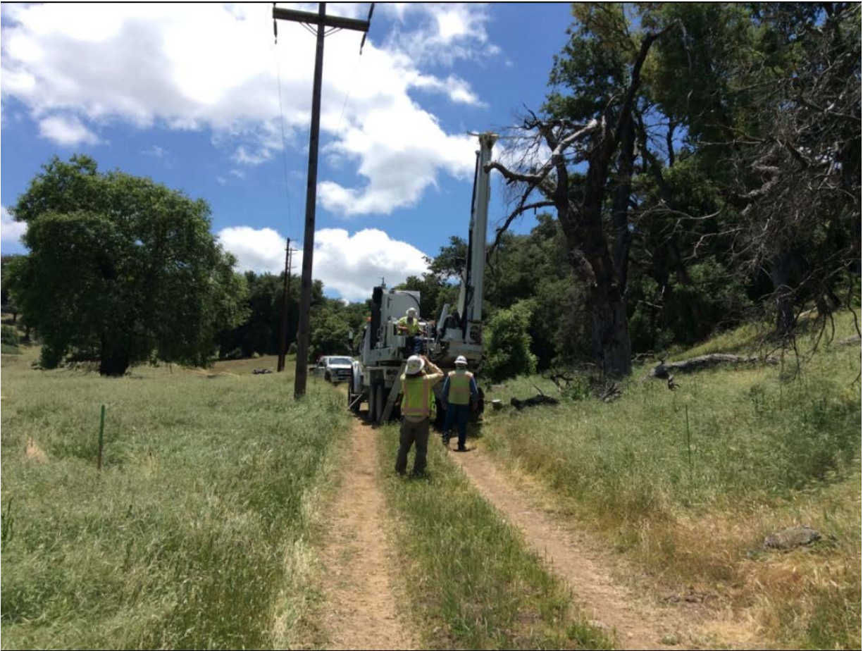
Photo 4: A crew was observed drilling a direct-bury pole hole at P259355 (TL 626 Conversion North (C 222)). A qualified biologist, who had conducted bat surveys and identified active bat roosts nearby in accordance with MM BIO-30, was present to monitor the roosts during construction activities.
