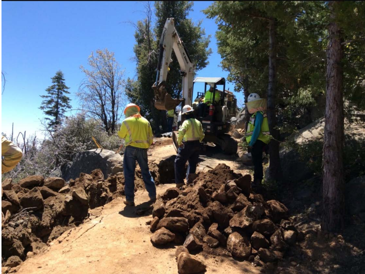
Photo 3: A biological monitor was observed monitoring trench excavation near 20+00 (C 79A) in accordance with MM BIO-22.
