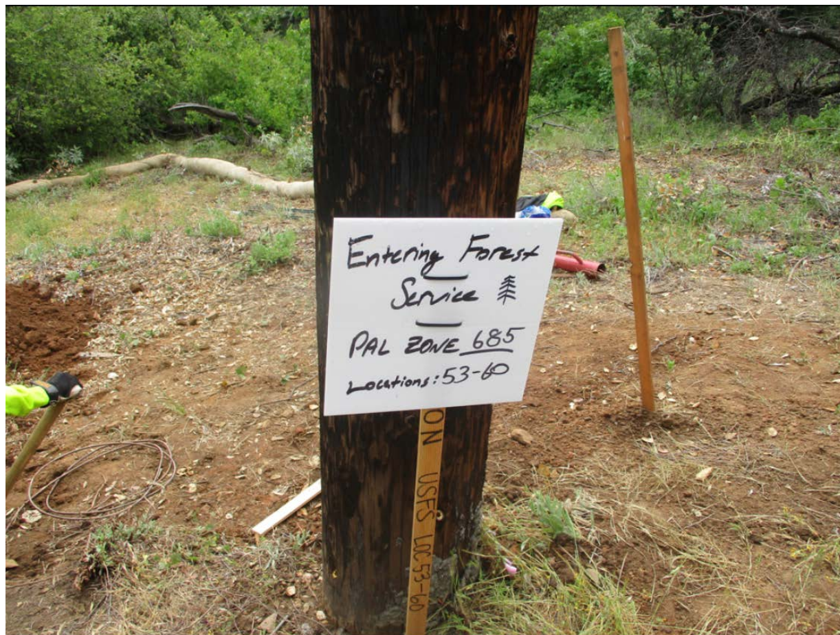
Photo 5: At P259359 (TL 626 Conversion North (C 222)) where a crew was observed digging a pole hole, the location was clearly marked to ensure compliance with the CFPPP fire prevention matrix compliance (MM FF-1), and required tools were at the site.
