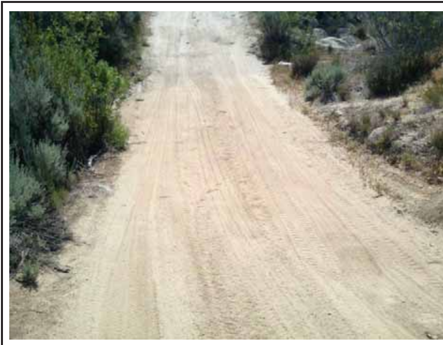
Photograph 12: View of steep vertical curves at the water crossing on AR-7 where installation of a temporary dip section and wire mesh fencing to catch fill is required.
