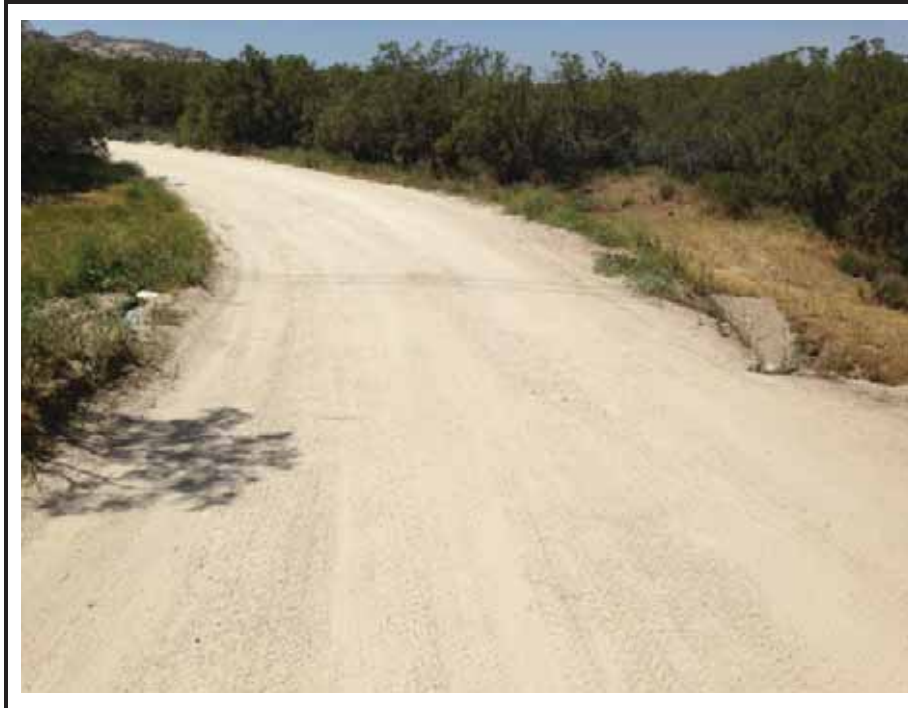
Photograph 9: View of erosion on Access Road- (AR-) 1 at the culvert crossing, which requires repairs to the rock retaining wall, filling of eroded areas to rebuild and widen the road, and placement of steel plating to protect the culverts.
