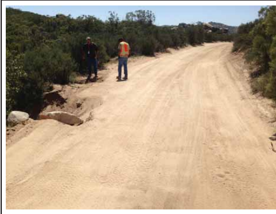
Photograph 11: View of erosion on AR-4, which requires filling eroded areas to rebuild and widen the roadway and placement of steel plating to protect the culvert.
