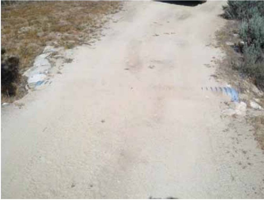
Photograph 13: View of erosion at the crossing of a shallow, narrow culvert on AR-11, which requires installation of a dip section and removal of the existing culvert.
