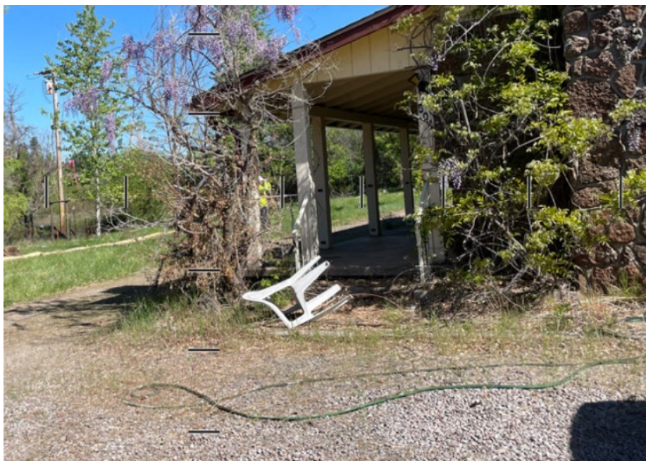
Photo 5: An EM was observed monitoring status of active nest on one of the structures to be demolished in accordance with APM BIO-7.
