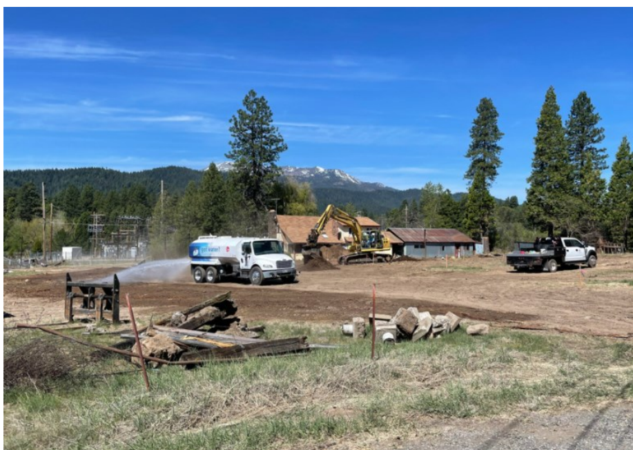
Photo 6: During site preparation activities, water trucks were observed on site applying water to soils to control particulate matter emissions in accordance with APM AQ-1.
