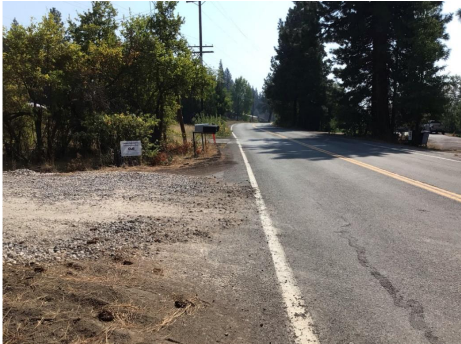
Photo 3: The stabilized construction entrance (gravel base) was observed in compliance with the SWPPP (APM WQ-1).
