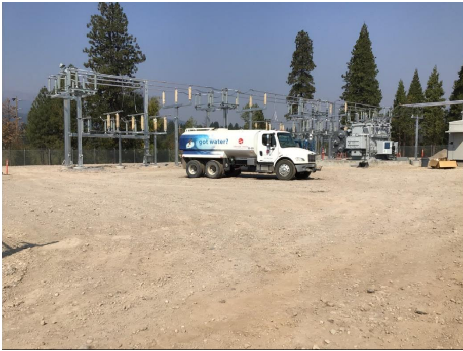
Photo 1: A water buffalo was observed on site and has been actively wetting roads and unpacked construction areas, in compliance with SWPPP and dust (APM AQ-1).
