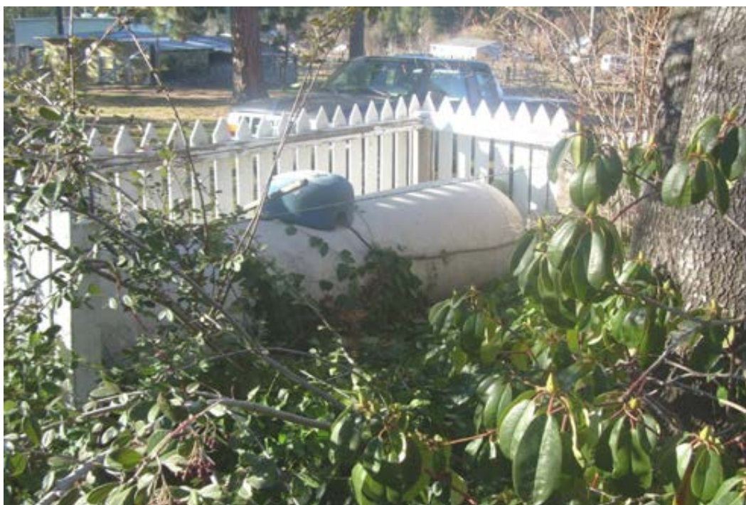
Photo 8. View of the propane aboveground storage tank.
