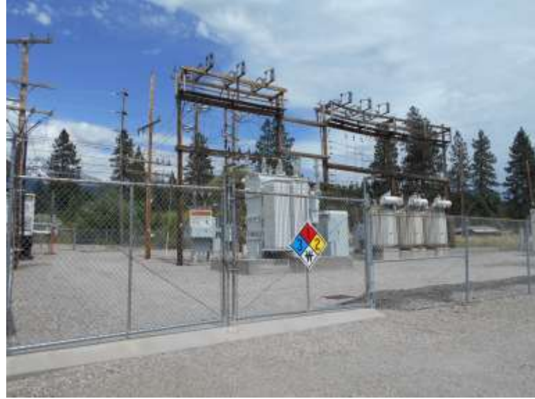
Photo 6. View of the existing Mount Shasta Substation at 404 South Old Stage Rd.
