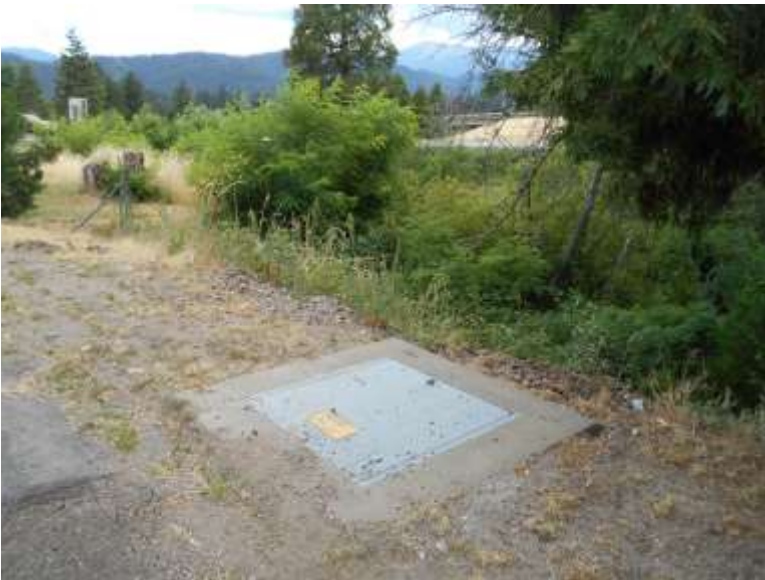
Photo 7. View of the underground distribution area near The Tree House Motor Inn at 111 Morgan Way.
