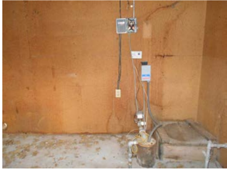
Photo 6. Interior view of the well shed located at 506 South Old Stage Road.
