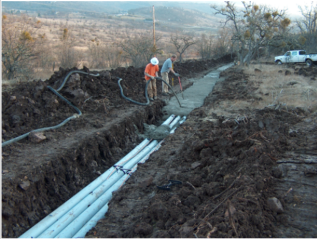
This shallow trench filled with 2000 psi FTB set in soil of high thermal resistivity met PacifiCorp's specified ampacity, while other approaches were prohibitively expensive.
