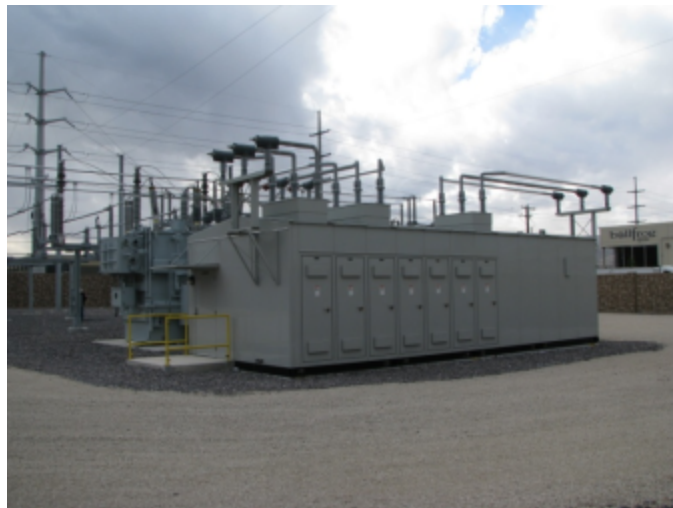
Figure 1—Typical Metalclad Switchgear at a Substation
