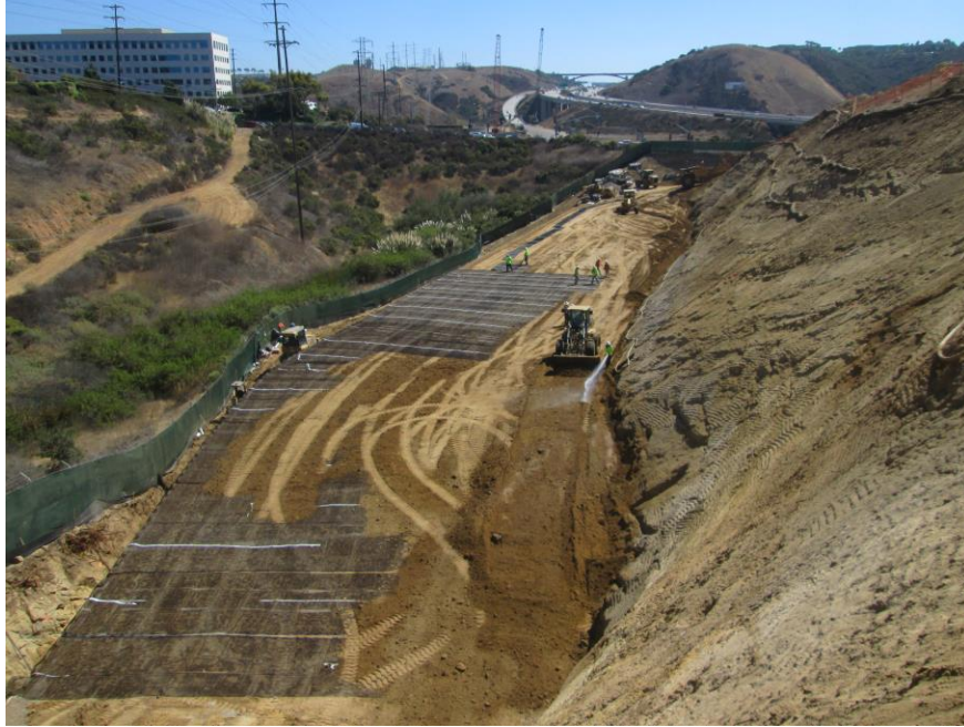
Photo 1: Overview of the Mira Sorrento Substation looking south from Mira Sorrento Place. Crews can be seen placing geogrid fabric associated with the retaining wall construction.
