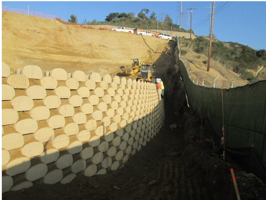
Photo 2: Construction of the retaining wall along the eastern project limits. Construction crews reported that the top of the retaining wall is up to an elevation of approximately 150.5 feet AMSL.
