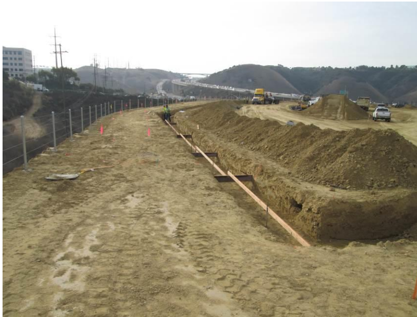
Photo 1: Construction crews initiated work associated with the foundation for the perimeter screening wall during this reporting period.
