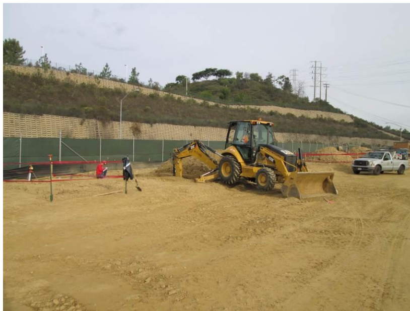
Photo 2: Excavation associated with construction of a getaway where existing distribution lines will be connected to substation facilities.
