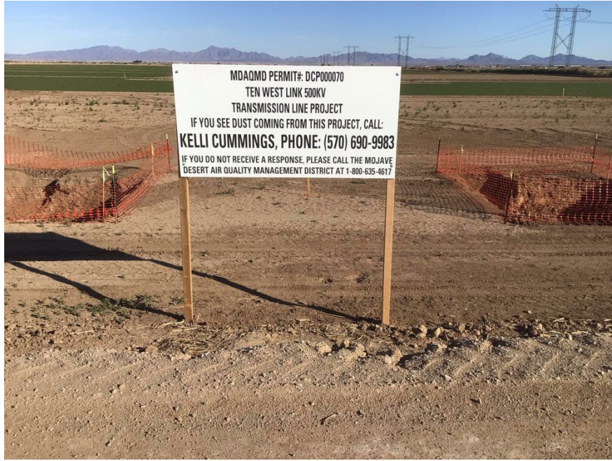
Photo 1: Dust and air quality sign installed in accordance with APM-AQ-01.
