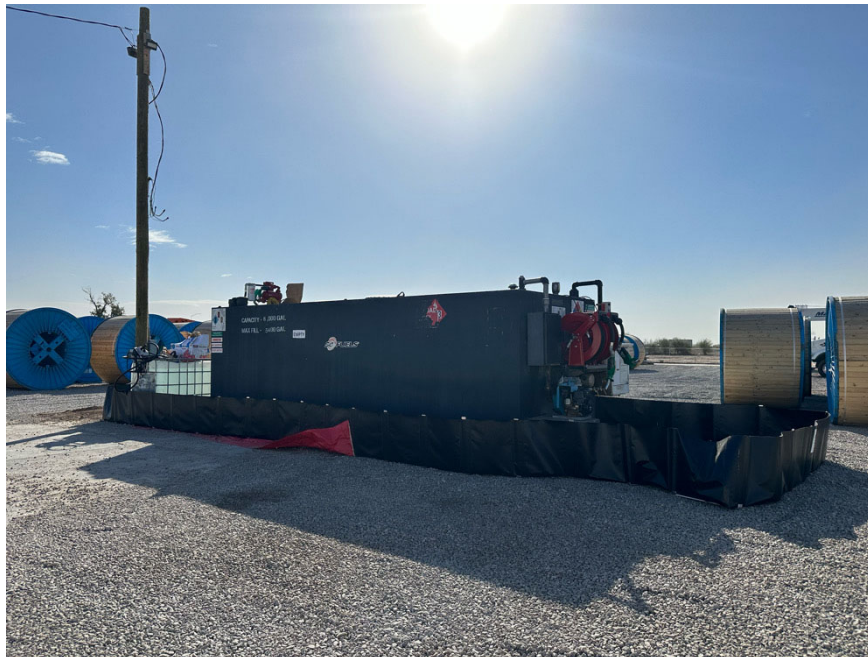
Photo 2: Secondary containment installed under fueling station at the laydown yard in accordance with BMP-BIO-34.
