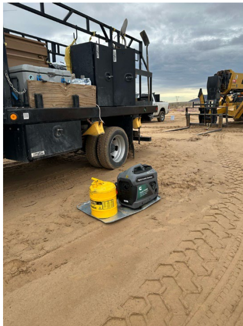
Photo 4: Drip pan installed under gas can and power equipment.
