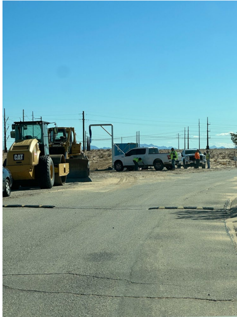
Photo 1: Crew members using weed wash station prior to entering the ROW in accordance with BPM BIO-12 and LUPA BIO-10.
