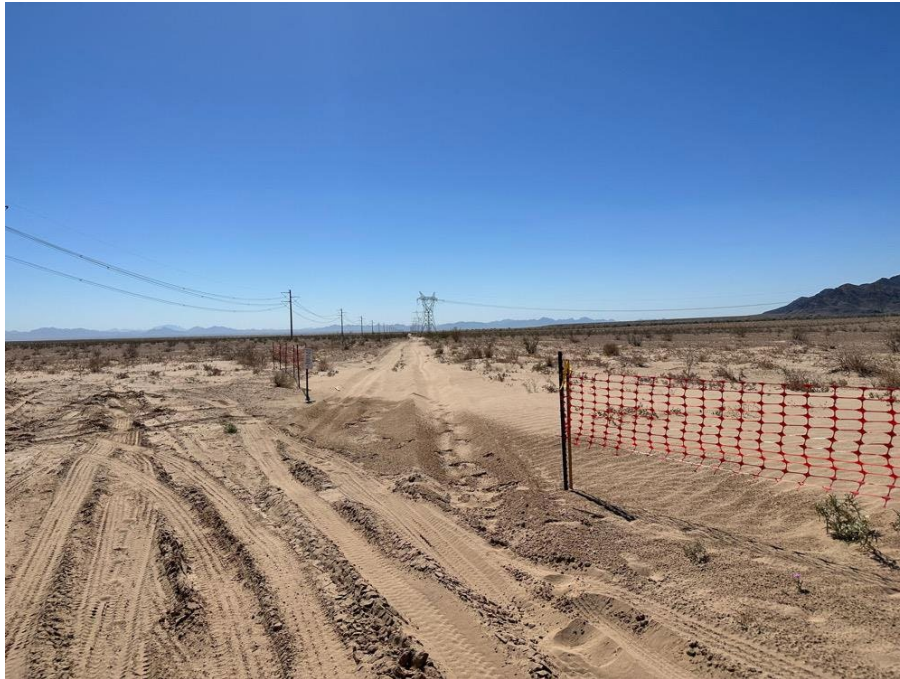
Photo 2: Snow fencing installed on site and not deterring the natural flow of the sand and grade in accordance with BMP BIO-54.
