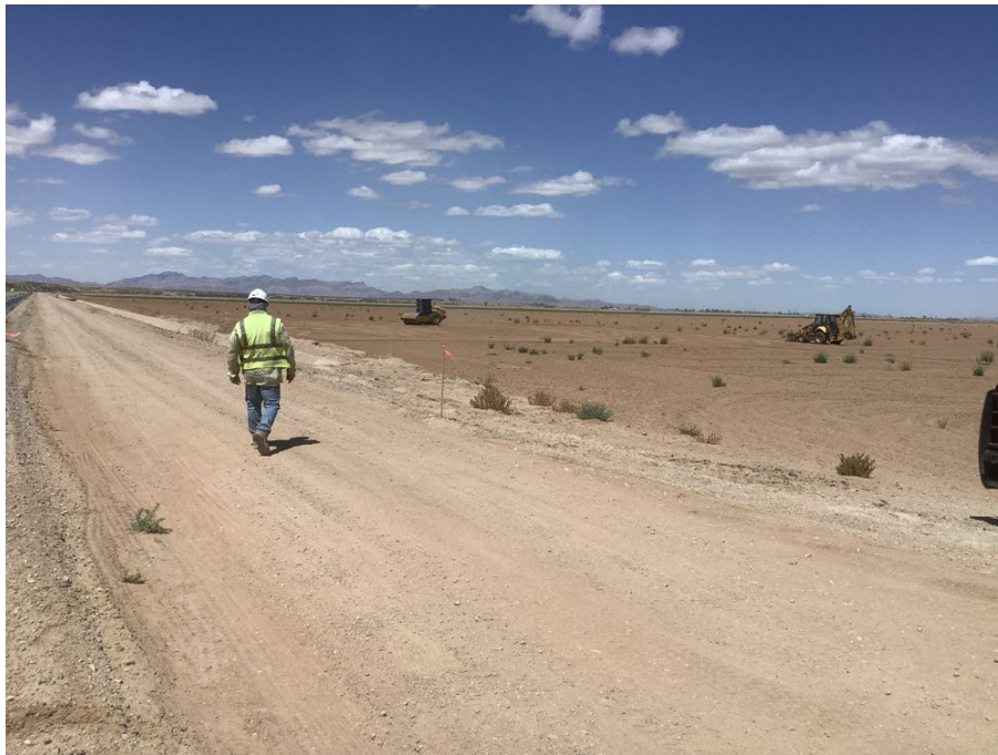
Photo 2: Approved biologist observed sweeping work areas for wildlife during construction activities tower pad 407 in accordance with BMP BIO-23 and BIO-49.
