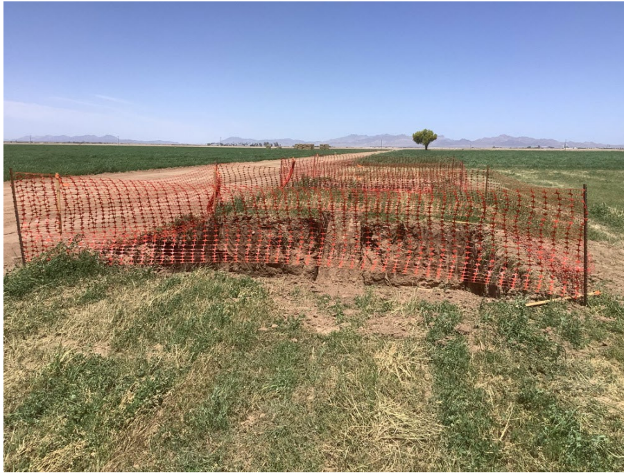
Photo 1: Wildlife escape ramp present at the excavation site and area clearly marked off to avoid any fall incidents BPM BIO-09.
