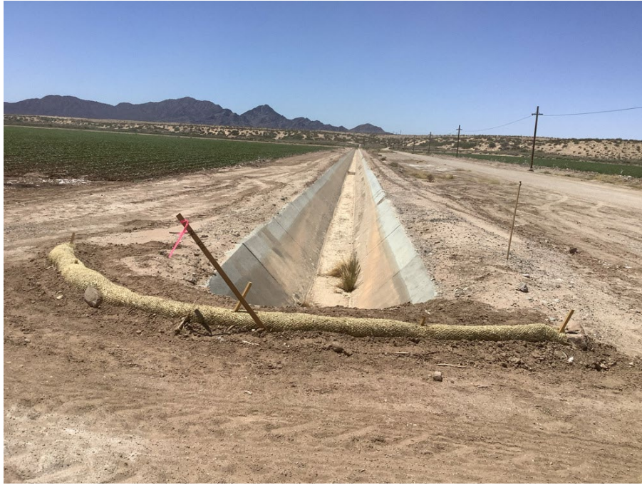
Photo 5: BIO-10 BMP installation in good condition.
