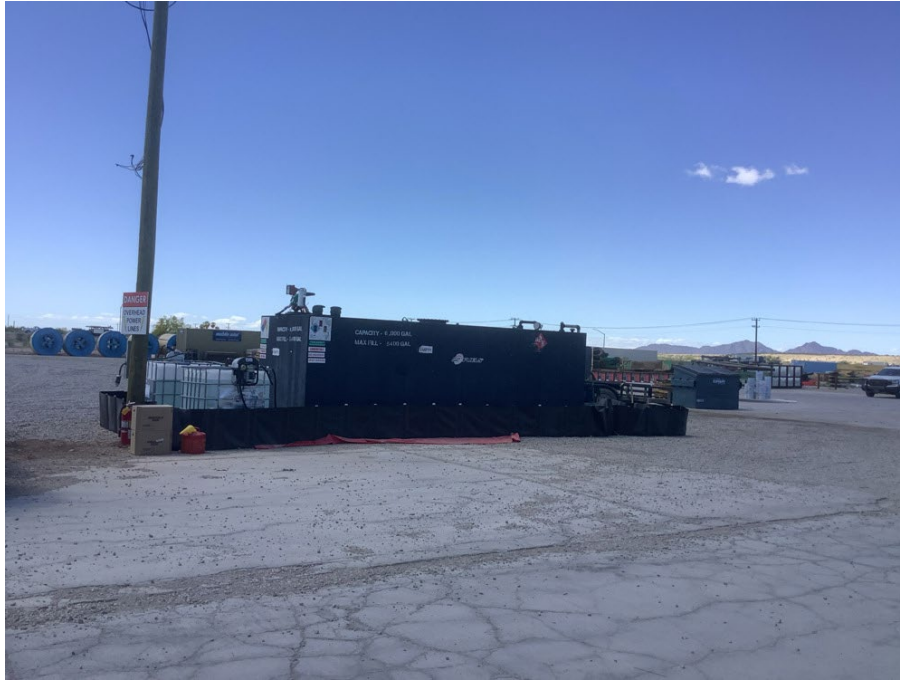
Photo 3: Secondary containment present for fuel storage in accordance with HAZ-01.
