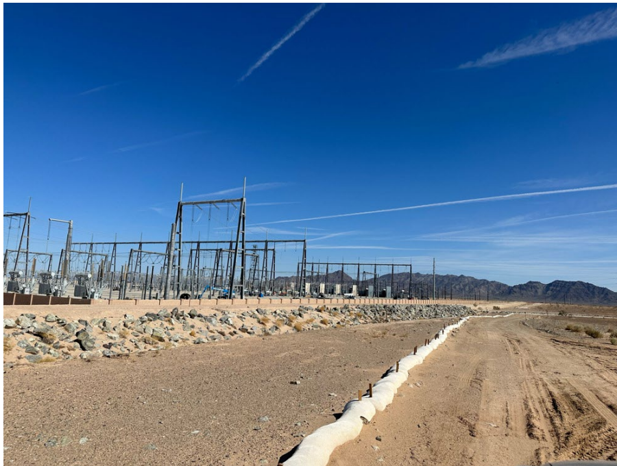
Photo 2: Straw waddles near 421 fully functioning in accordance with APM-GEO-01.
