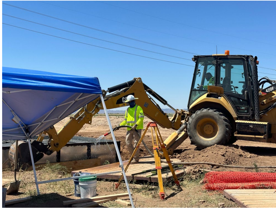
Photo 5: Backfilling activities being watered to control fugitive dust in accordance with Q-01, APM BIO-10, BMP BIO-34.
