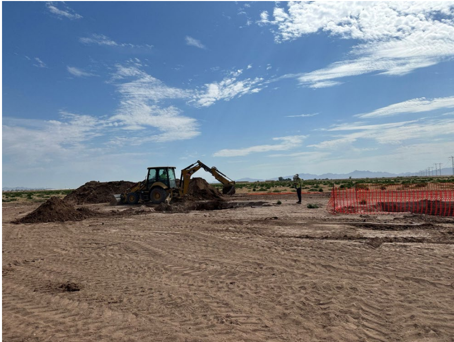
Photo 2: Biologist monitoring digging at an agricultural tower pad in accordance with BIO-25.
