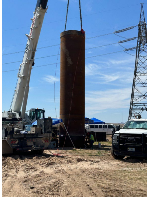
Photo 5: Welding activities and fire Marshall on standby in accordance with DFA-VPL-BIO- FIRE-1.
