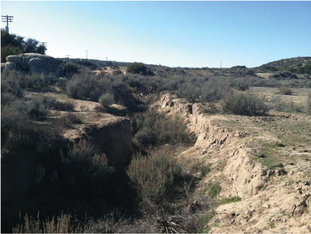
Photograph 9: Feature H Facing upstream (generally northwest) along western edge of Boulevard Staging Yard.
