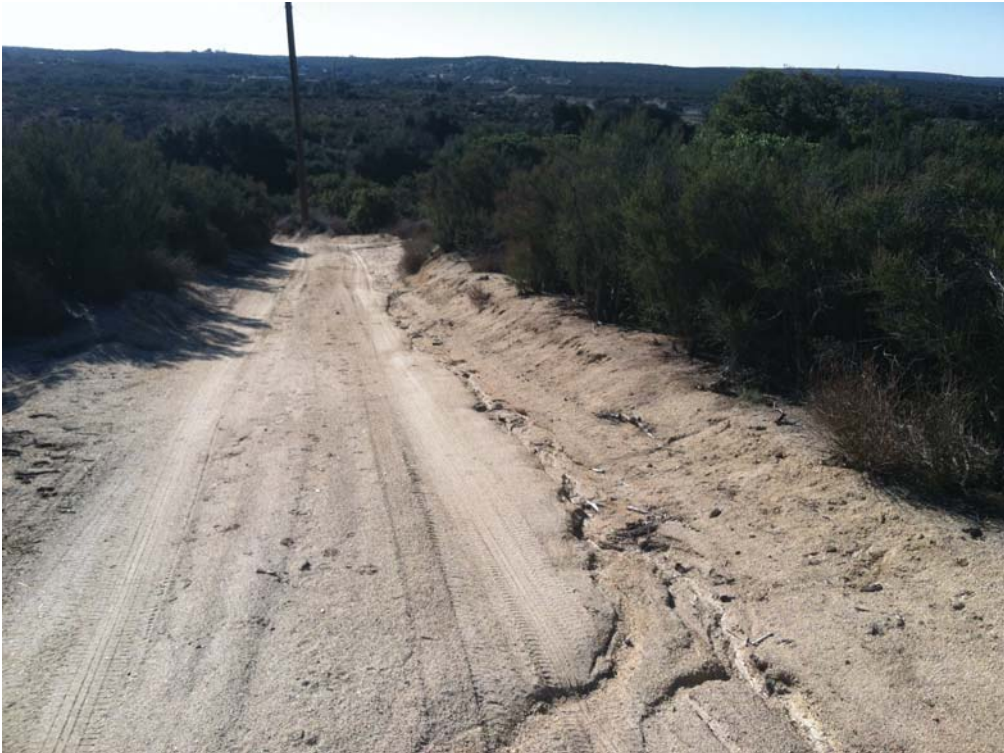
Photograph 10: Erosional Feature Erosional feature common along existing roadways through the Study Area. Facing generally south.
