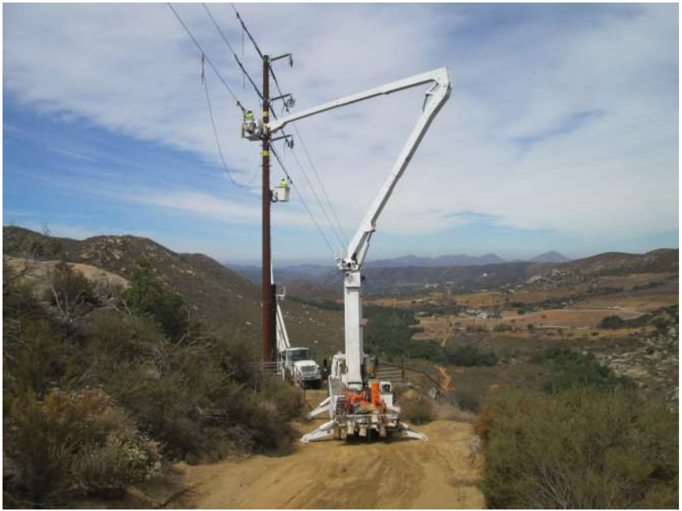
Photo 1: Construction crews were observed conducting wire stringing activities, which included dead-ending and sagging the wire (pictured above). Crews were observed staying on existing approved roads for this activity.
