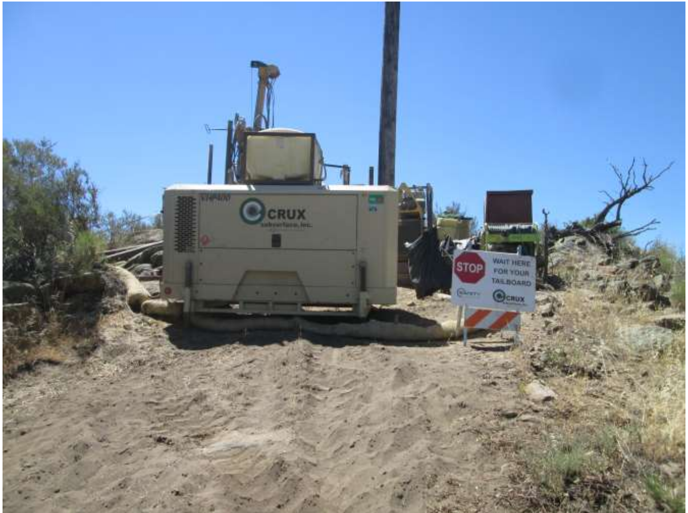
Photo 3: During micropile activities, erosion control features such as straw wattles were installed around project equipment and remained in-tact. Signage reminding crews of additional safety requirements (briefings) prior to entering the work area was observed at the edge of work limits.
