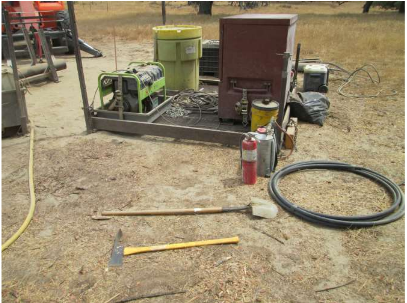
Photo 8: During micropile activities, in accordance with the Project Fire Plan and APM HAZ-2, fire suppression tools (Pulaski, shovel, fire extinguisher, and 5-gallon water pump) were observed staged at work locations. Secondary containment was observed staged under generators in accordance with the SWPPP.
