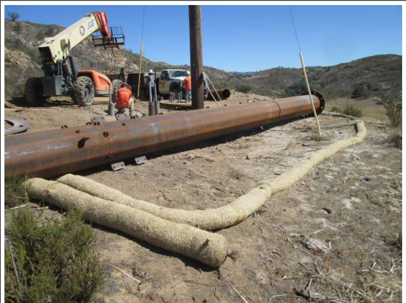
Photo 4: Crews were observed de-mobilizing micropile foundation equipment once foundations were completed and steel poles were staged at pole replacement locations. Erosion control features such as straw wattles (pictured above) remained in-tact and were observed being inspected by aquatic monitors (APM HYD-4).
