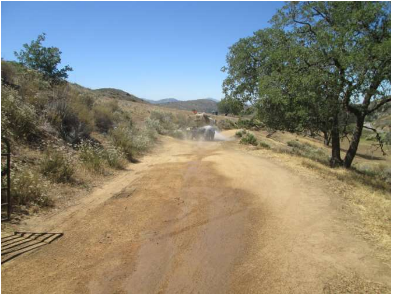
Photo 7: Project access roads were observed being watered in order to prevent fugitive dust in accordance with APM BIO-1.
