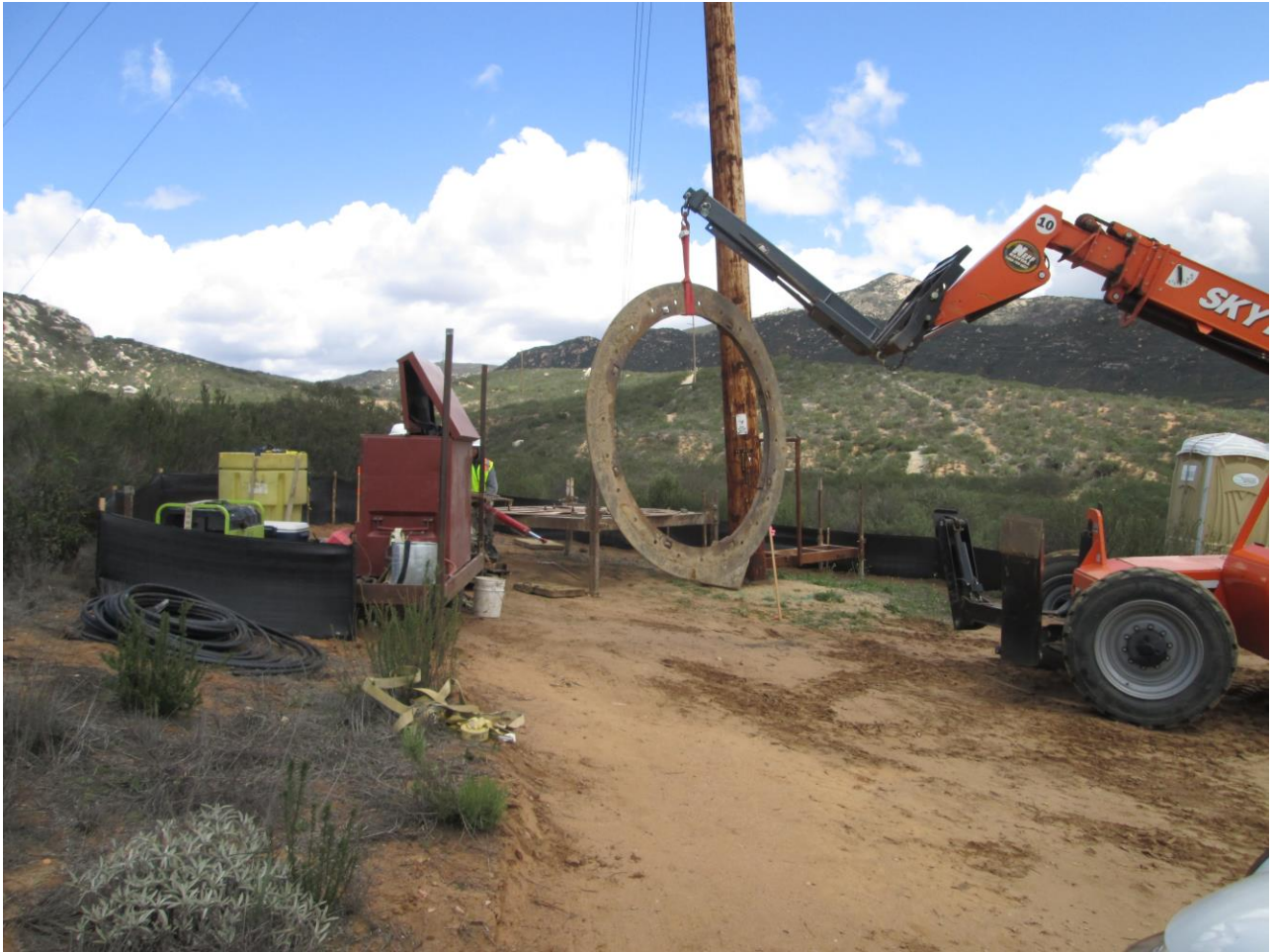
Photo 1: Crews were observed setting up drill platforms for micropile sites (Above, Location 30). Silt fencing was observed installed and intact in accordance with the Project SWPPP/APM HYD-1. Portable restrooms were observed staged on secondary containment in accordance the Project SWPPP.
