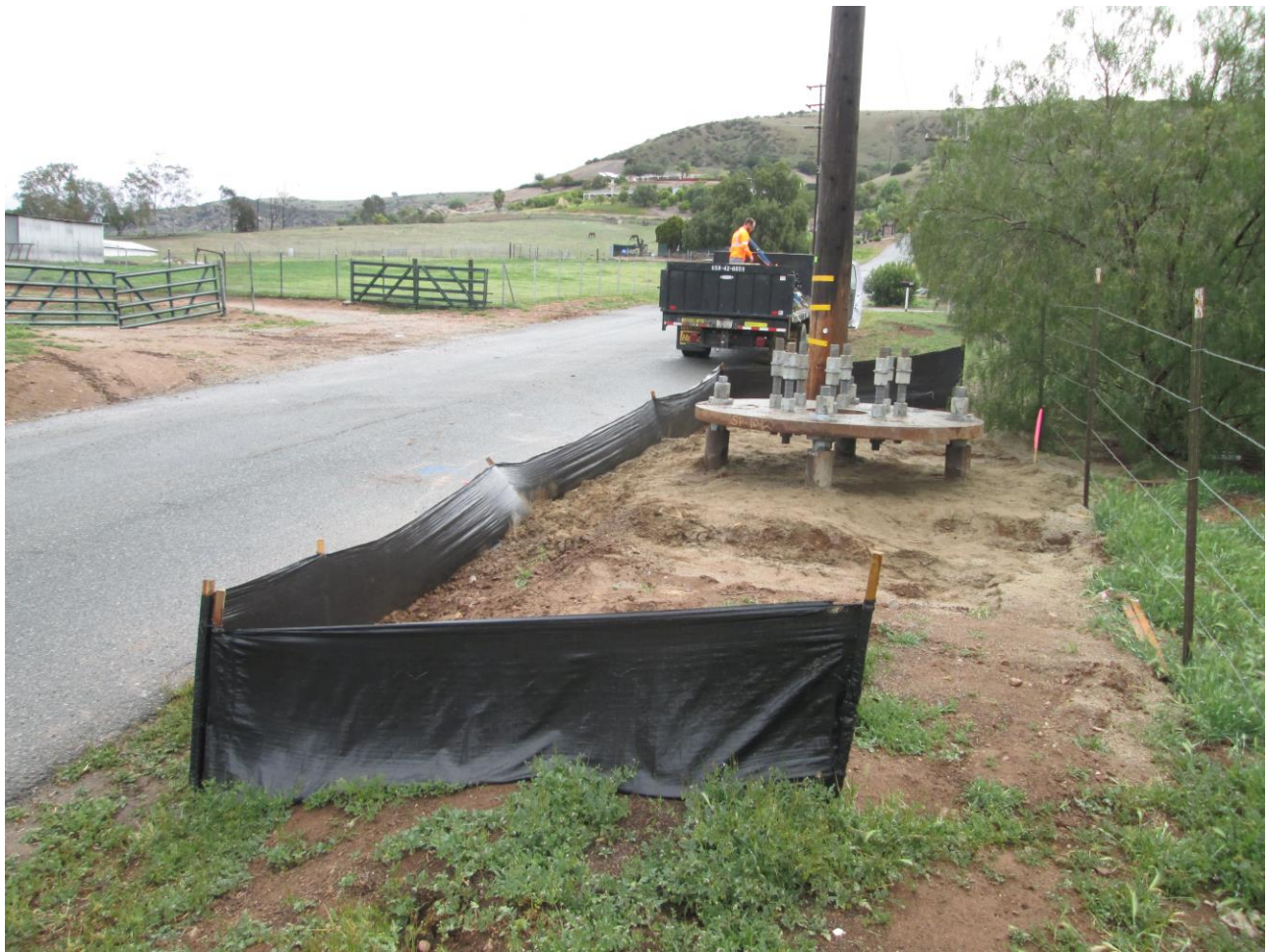
Photo 2: Finished/Capped Micro Pile foundation. Silt fencing was observed installed and intact in accordance with the Project SWPPP/APM HYD-1 and crews were observed cleaning all excess grout with shovels and buckets. Due to this location being situated near a jurisdictional waterway, an aquatic resource monitor was observed present during activities in accordance with MM HYD-4 and the Section 401 Certification.
