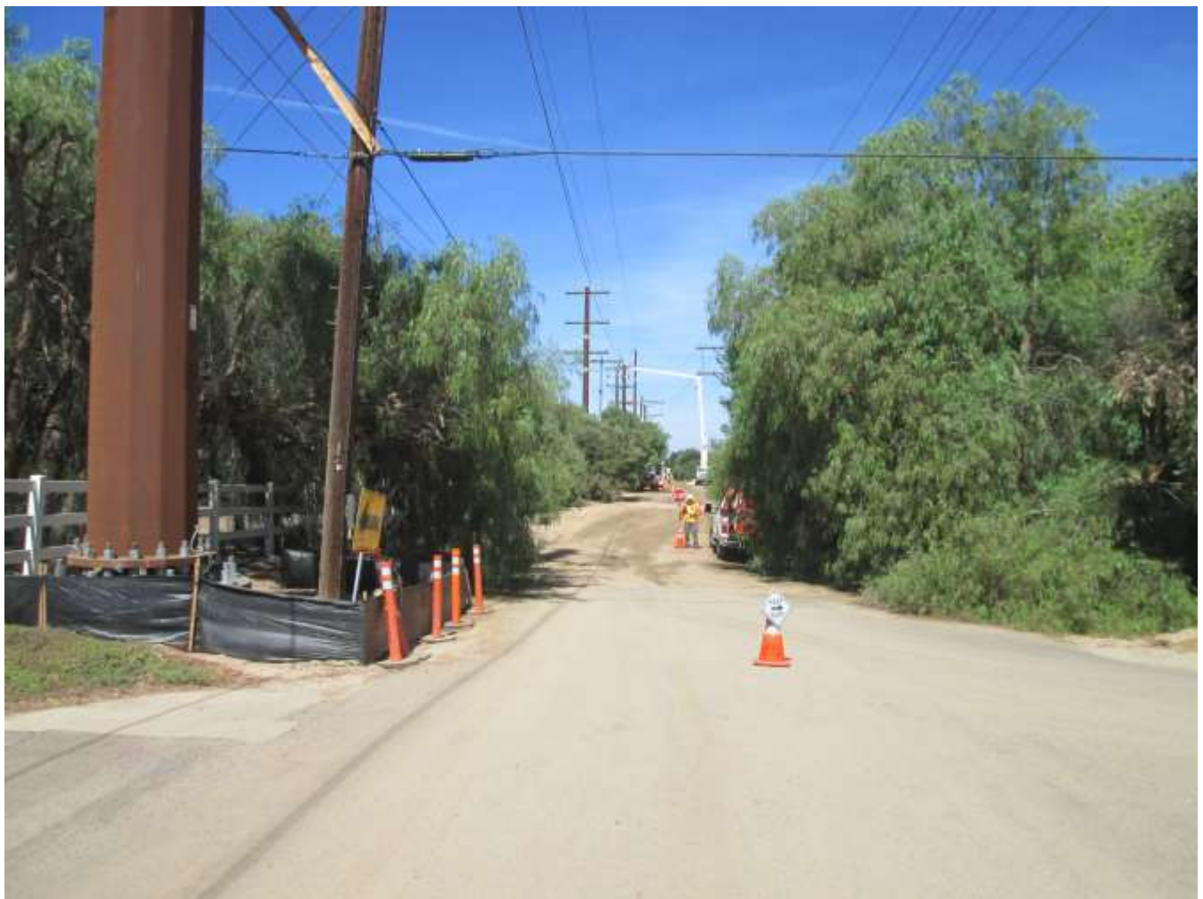
Photo 6: In accordance with APM TRA-1, traffic control crews and cones were mobilized during pole re-framing activities along Creelman Lane. Additionally, biological monitors were observed monitoring a nearby nest during these activities, which was marked with green lathe signage for avoidance (BIO-2).
