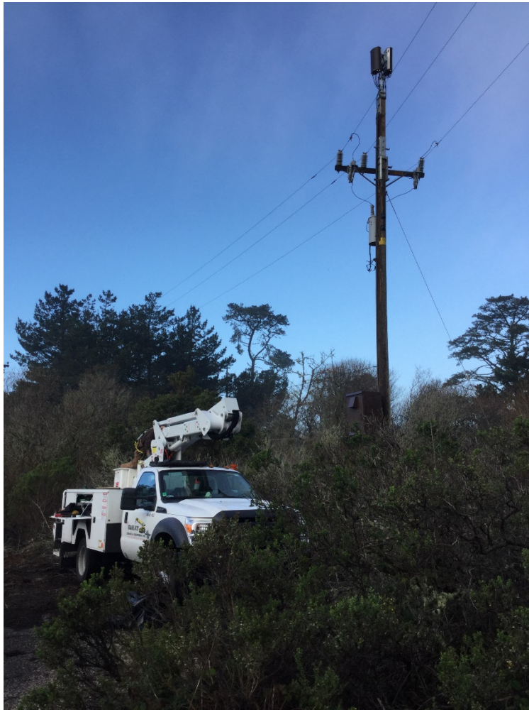
Photo 5: Aerial antennae installation.
