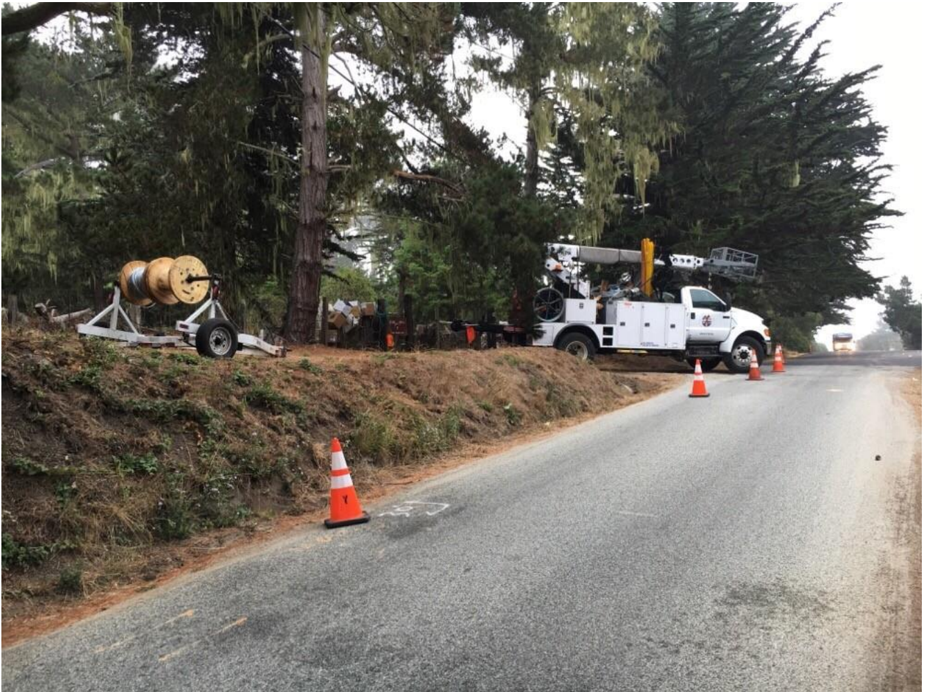
Photo 2: Crews working at north end of Bean Hollow Rd. Road access maintained.
