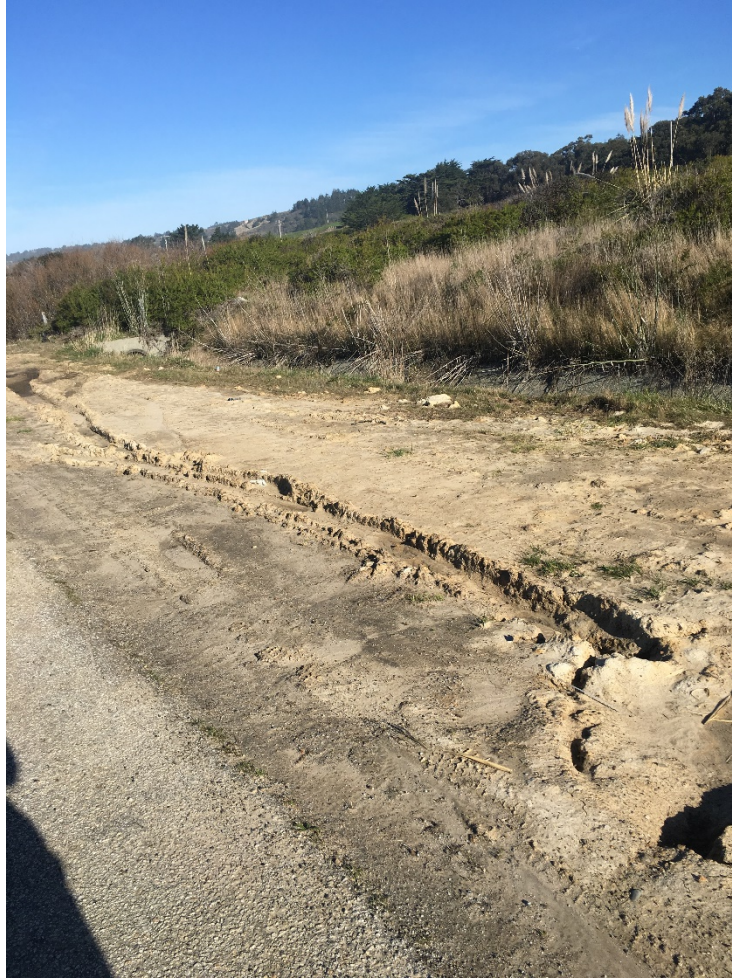
Photo 3: Tire ruts on Highway 1 northbound shoulder, mile marker 5.38.
