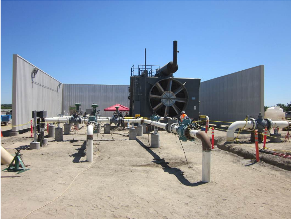
Photo 1: Temporary compressor and sound wall completed at the remote well pad site.
