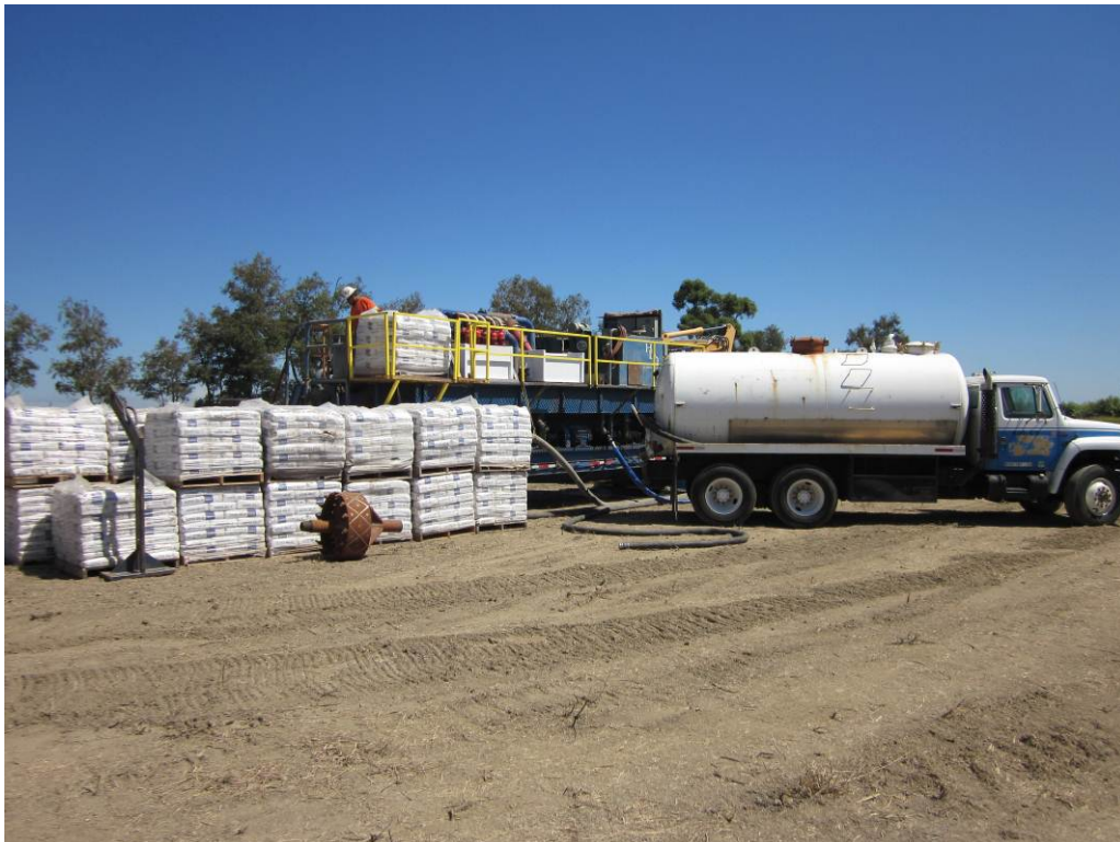
Photo 6: HDD rig setup on the eastern side of the NRCS wetland/Gunnersfield crossing.
