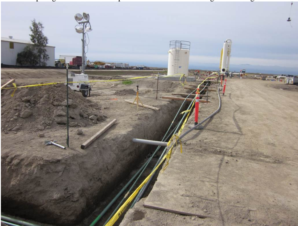
Photo 4: Excavated trench for small-diameter gas lines at the southern end of the Compressor Station site.
