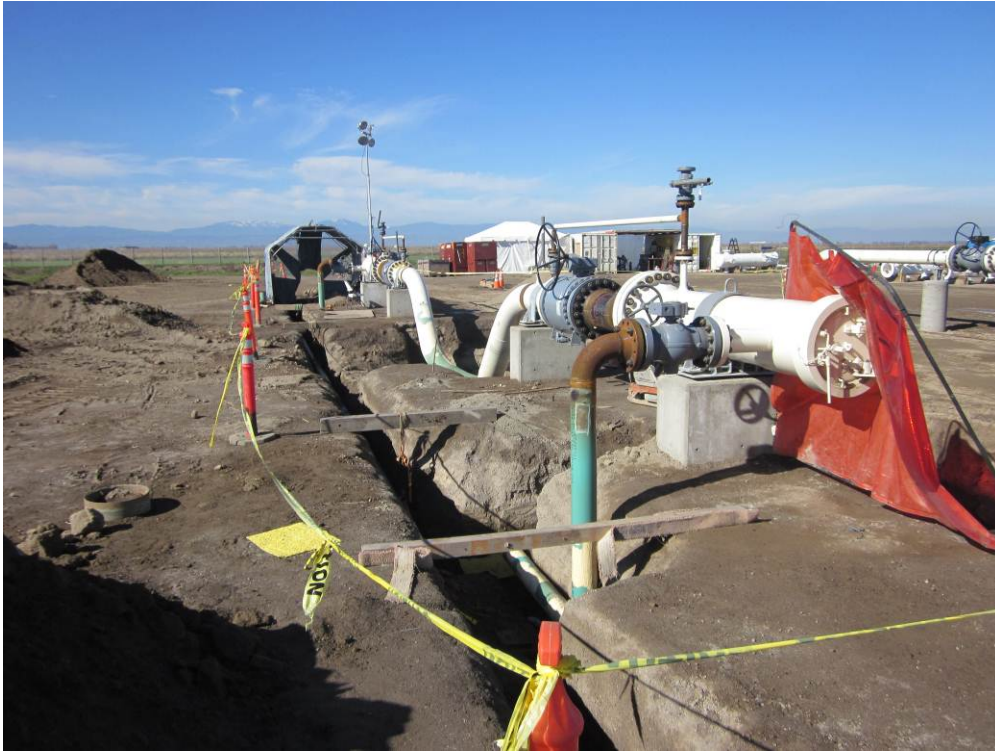
Photo 1: Excavated trench for small-diameter pipe installation at the Remote Well Pad site.
