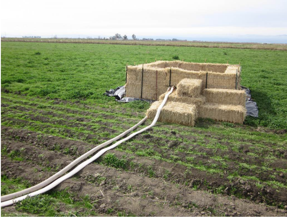
Photo 3: Saltwater tank test water disposal site on adjacent field (Variance 16). Energy dissipating device installed to prevent soil movement during de-watering efforts..
