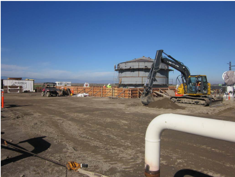
Photo 2: Construction of the saltwater tank has been completed at the Remote Well Pad site.
