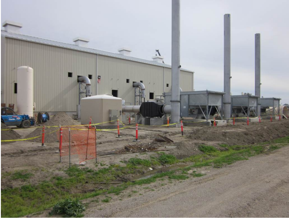
Photo 5: Caterpillar units installed and connected to the west side of the compressor building at the Compressor Station site.
