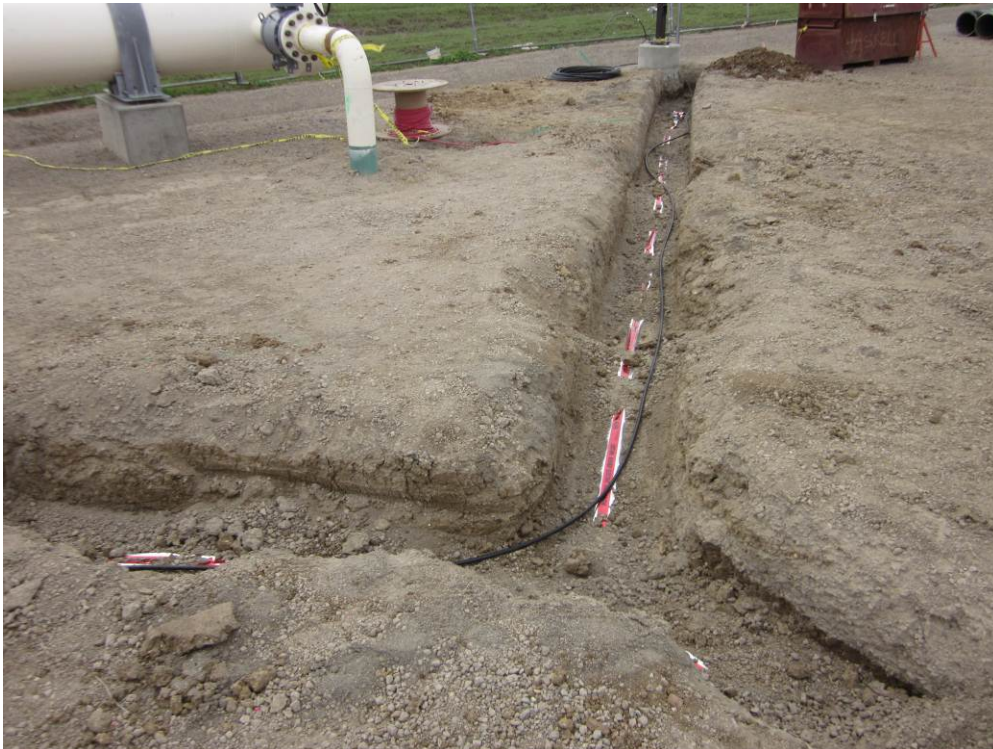
Photo 6: Exposed electrical line trench at the Metering Station. Backfilling of these trenches in other areas of the site was underway.
