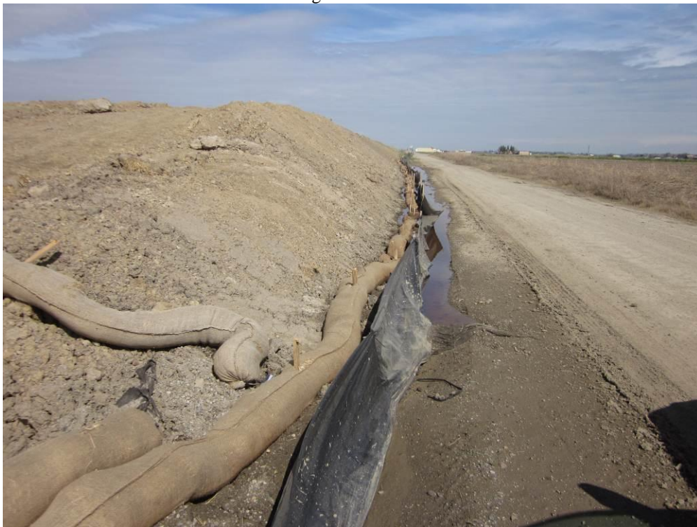
Photo 4: Silt fence and fiber roll places along the edge of the soil stockpile adjacent to McAusland Road.
