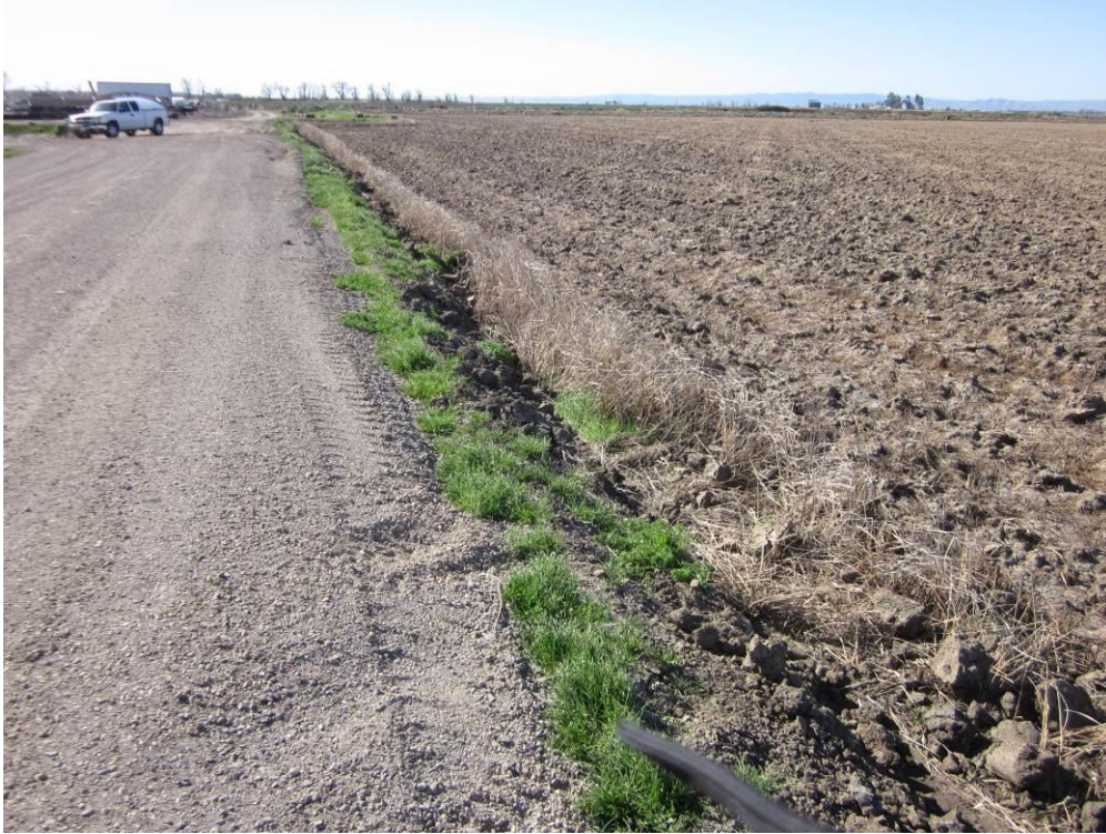
Photo 5: Silt fence has been removed from the western boundary of the Compressor Station site following site review and recommendations by the project QSP.
