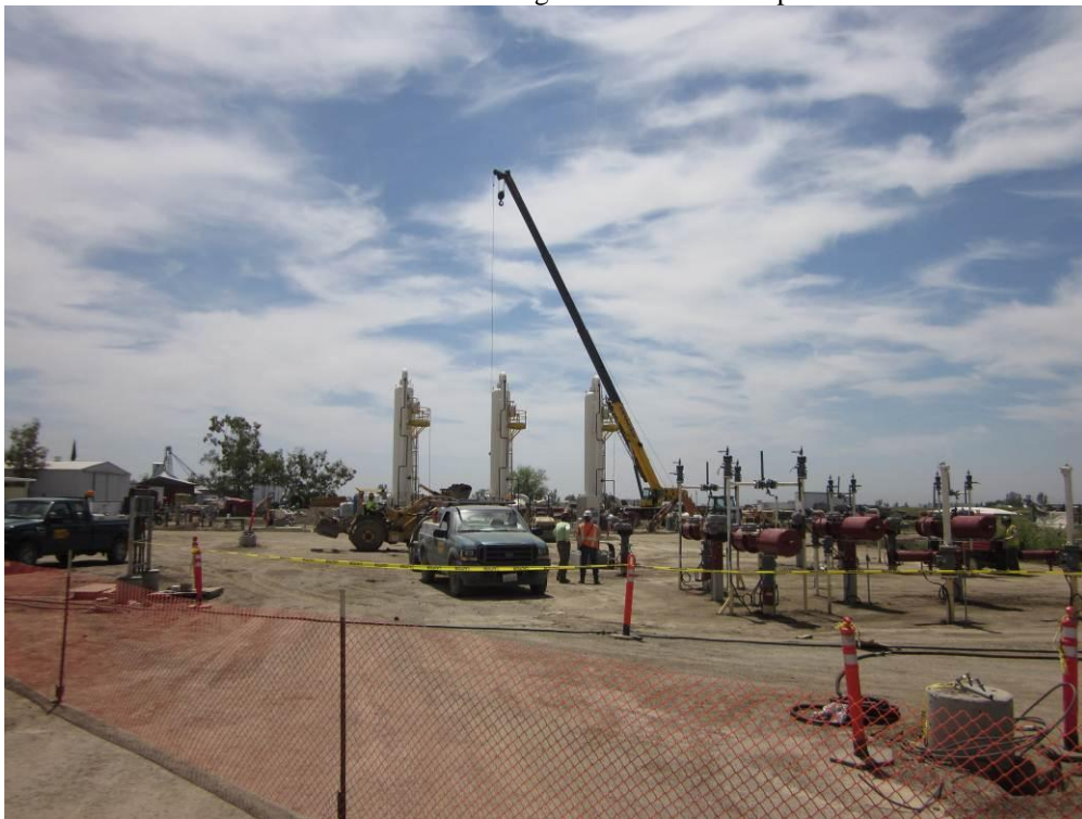
Photo 4: Work on one of the dehydration towers was underway at the Compressor Station site.
