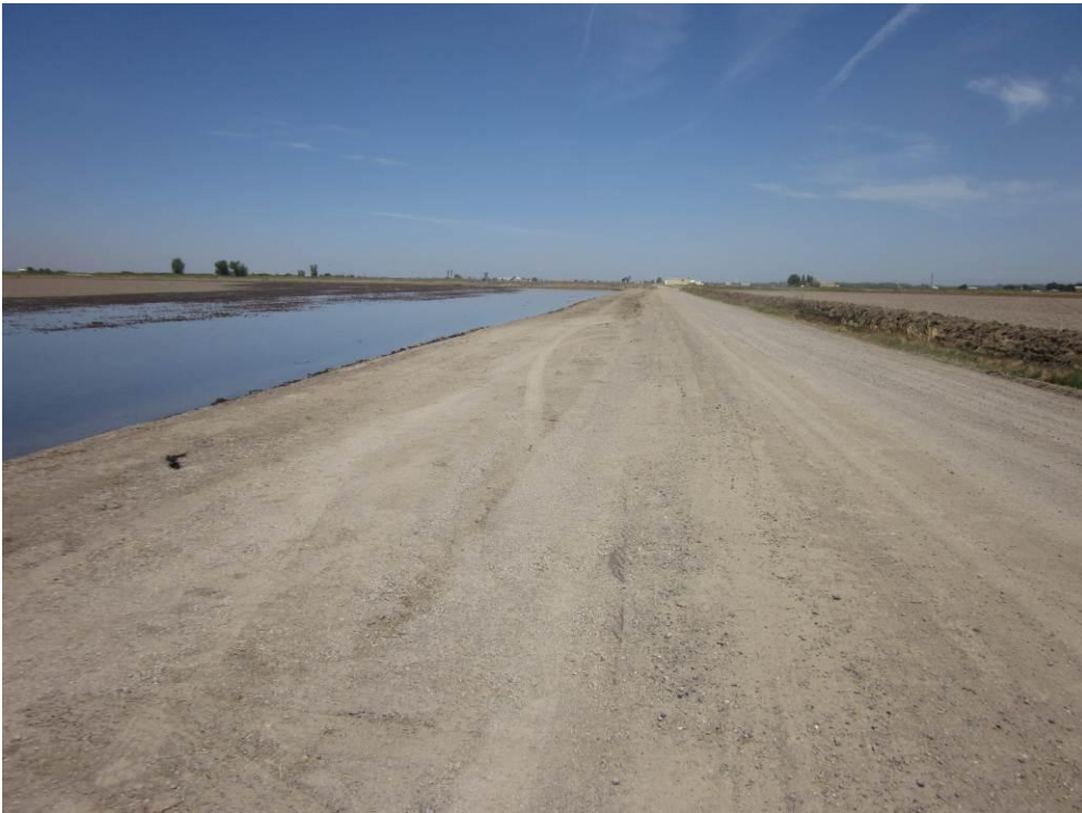
Photo 6: The soil stockpile previously stored at Storage Area 1, immediately north of the Compressor Station site and adjacent McAusland Road, has been removed and the area returned to its previous condition.
