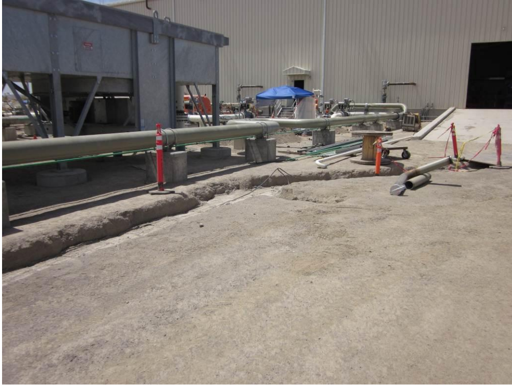
Photo 3: Electrical work was being conducted adjacent the compressor building. The buried electrical line trenches were also being backfilled in some portions of the site.
