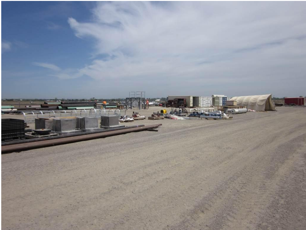
Photo 2: Materials are stored at the north end of the Compressor Station site and equipment framing fabrication was underway in this area.
