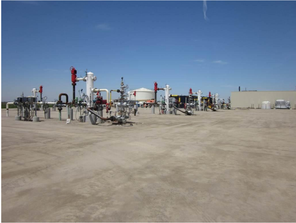
Photo 1: The Remote Well Pad site has been graded and much of the construction material removed.
