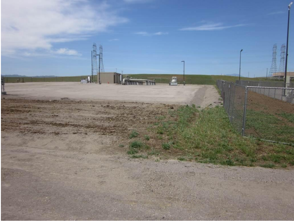
Photo 5: Final grading at the Metering Station site has been completed, with some final electrical tie-in work remaining. The temporary exclusion fence is also still in place at this site.
