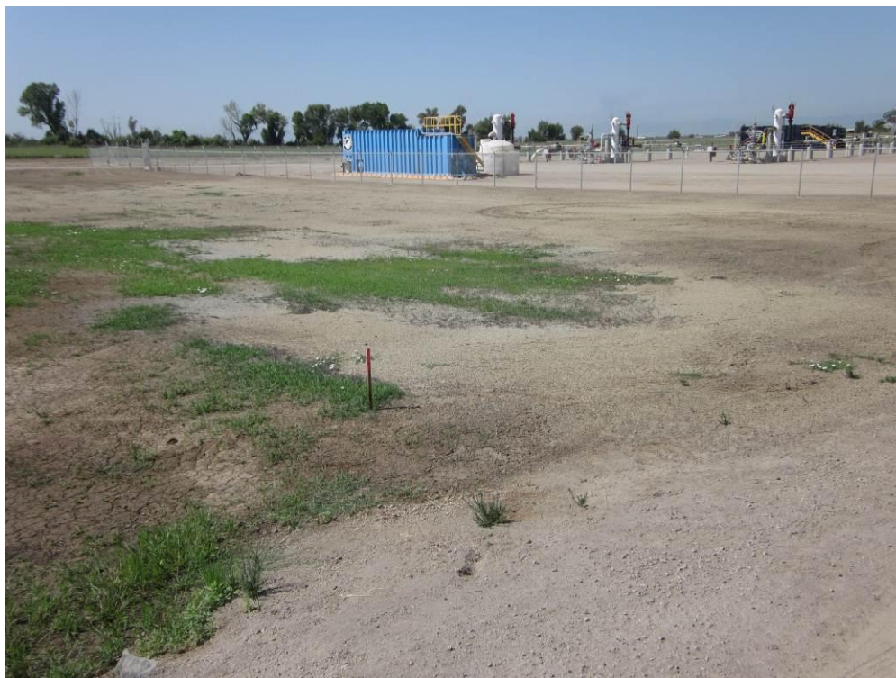
Photo 1: Remaining water tanks and materials at the Remote Well Pad site. The rest of the site has been graded and construction completed, with the exception of the anode bed wells).
