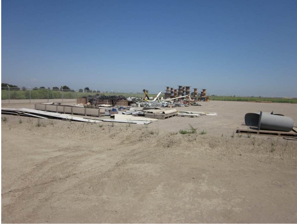
Photo 3: Construction materials remain in the northern portion of the Compressor Station site.
