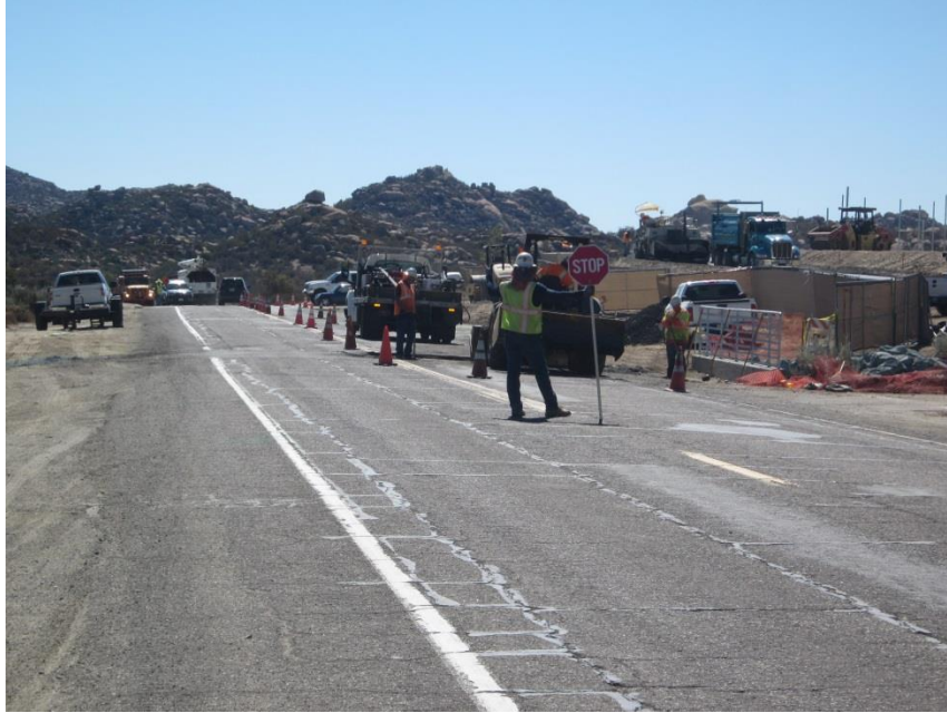
Photo 5: Traffic control was diligent in safely guiding local and project related traffic through work areas on Old Highway 80 in accordance with MM-TRA-1.
