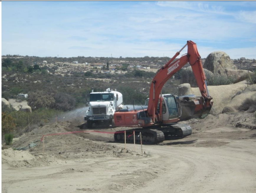
Photo 2: In accordance with MM-BIO4-A and MM-AQ-1, water trucks were used to control dust during finish grading of access roads north and south of Jewel Valley Road.
