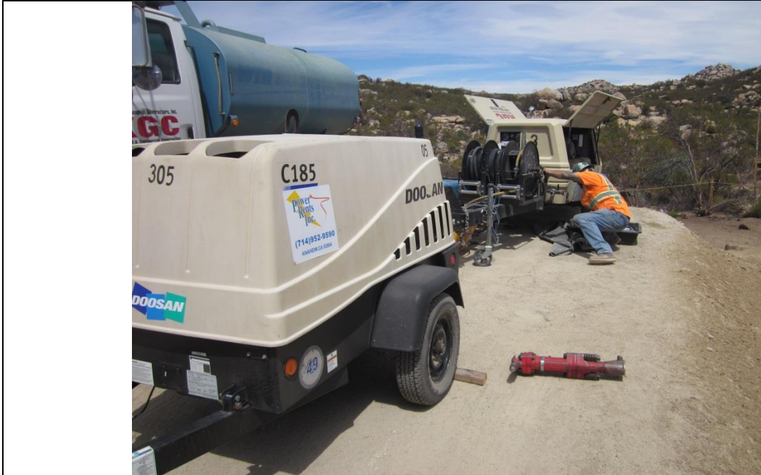
Photo 3: Crews at SP-50 were diligent in placing drip-pan containment under staged and active stationary equipment as required by MM-HAZ-1a.
