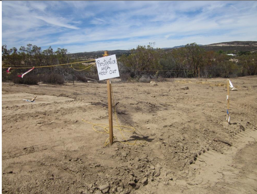
Photo 1: In accordance with Habitat Restoration Plan and MM-BIO-1d, topsoil is redistributed over a recontoured portion of Section 1 underground, and exclusion fencing has been installed to prevent access.
