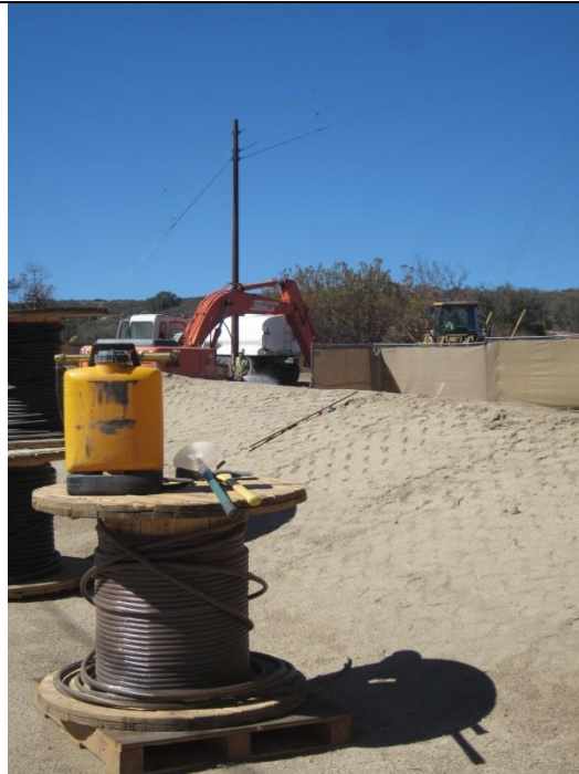
Photo 4: Throughout the substation, fire tools were set out at individual areas of work and attached to equipment for easy access in case of an emergency and in accordance with the Construction Fire Plan and MM-FF-1.
