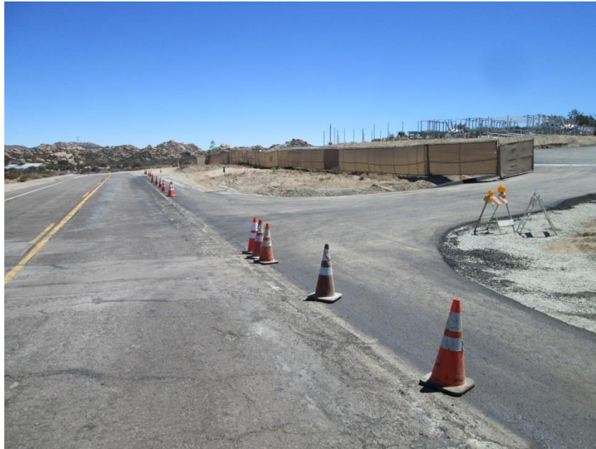
Photo 5: In accordance with MM-VIS-3a, the perimeter security fence includes screening material that is being maintained.
