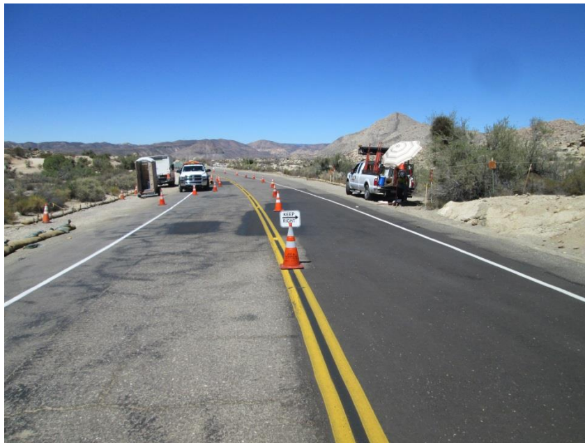
Photo 2: Traffic control measures consisting of signage and flaggers were observed being implemented during construction along Old Highway 80 in accordance with MM-TRA-1.
