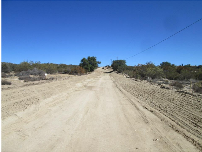
Photo 1: In accordance with Habitat Restoration Plan and MM-BIO-1d, construction crews return the right-of-way to pre-construction contour conditions.
