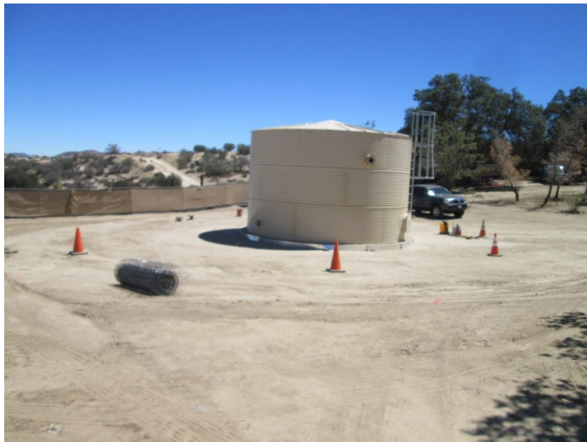
Photo 6: A 15,000 gallon water tank has been constructed at the Boulevard Substation Rebuild in accordance with MM-FF-4 and the Fire Protection Plan (FPP).
