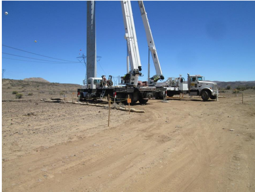
Photo 3: Erosion control measures consisting of straw wattles, silt fence and gravel bags are being maintained at steel pole pad sites in accordance with the SWPPP and MM-HYD-1.
