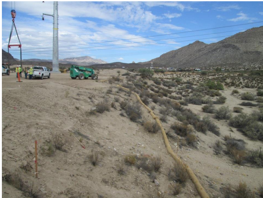
Photo 4: Biological monitors were on site to ensure construction activities remained within the approved work limits and to monitor for sensitive wildlife species (MM-BIO-1a and MM-BIO-1c).
