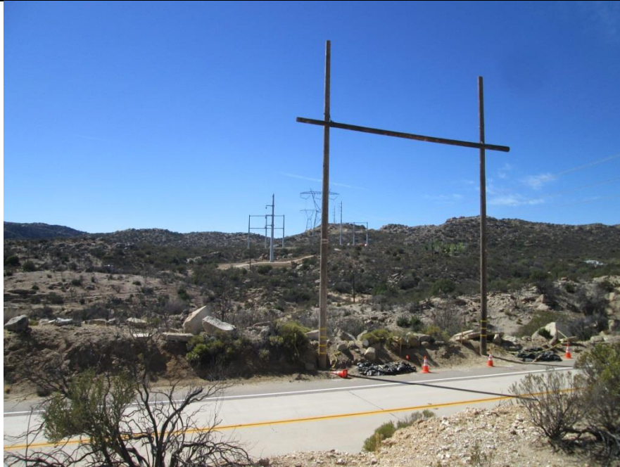
Photo 3: Temporary guard structures were observed constructed during activities associated with flying sock line to ensure safety for motorists along Old Highway 80.
