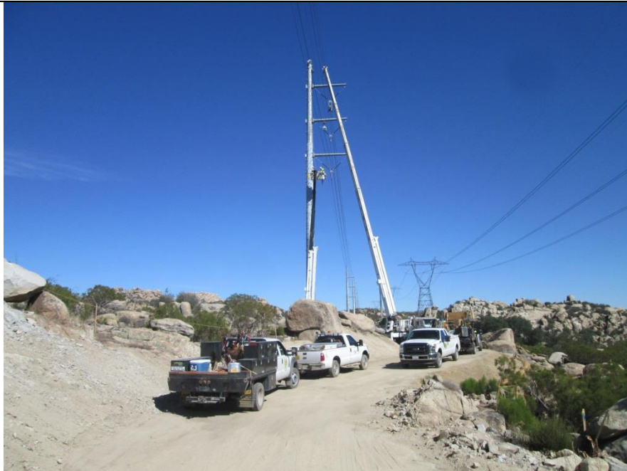
Photo 4: Crews were observed completing dead-end work at SP-48 within the approved work limits. Biological monitors were observed monitoring activities in accordance with MM-BIO-1c.
