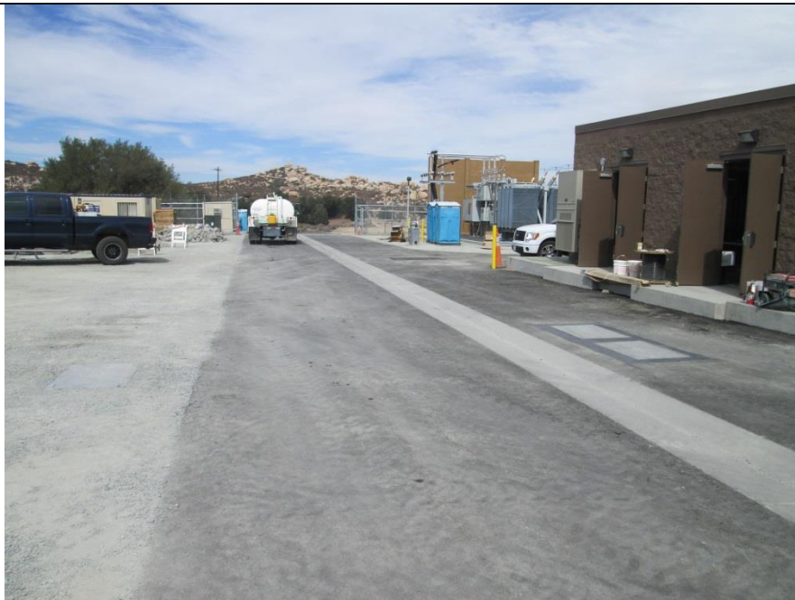
Photo 6: In accordance with the Surface Treatment Plan and MM-VIS-3g, the control shelter at the Boulevard Substation Rebuild have been surfaced treated “Otay Ranch Brown”.
