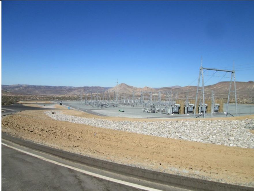
Photo 5: In accordance with the Surface Treatment Plan and MM-VIS-3g, the Transformer Fire Walls at the ECO Substation have been surfaced treated “Toffee Bar”.
