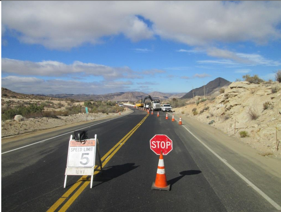
Photo 1: Traffic control measures consisting of signage, flaggers and escorts were observed being implemented along Old Highway 80 in accordance with MM-TRA-1.
