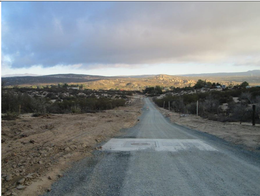
Photo 2: Class II base has been placed along the permanent access road for the 138 kV underground alignment. Restoration efforts consisting of decompacting soils adjacent to the permanent access road continued during this reporting period per MM-BIO-1D.
