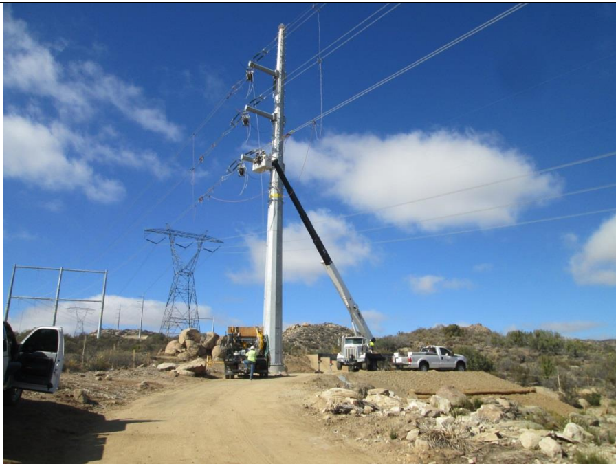
Photo 4: Crews were observed dead ending conductor at SP-65 within the approved work limits in accordance with MM-BIO-2A.
