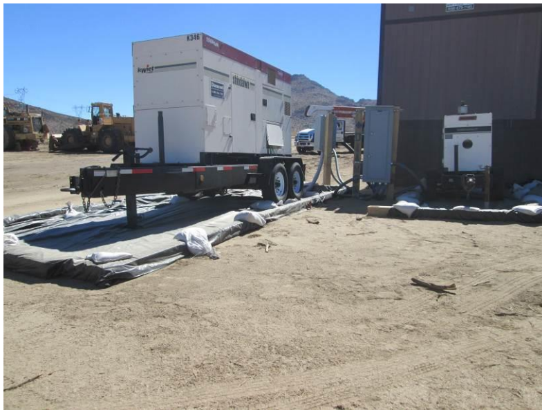
Photo 4: Secondary containment is observed under a generator to prevent leaks and spills in accordance with Mitigation Measure HYD-1 and the SWPPP.
