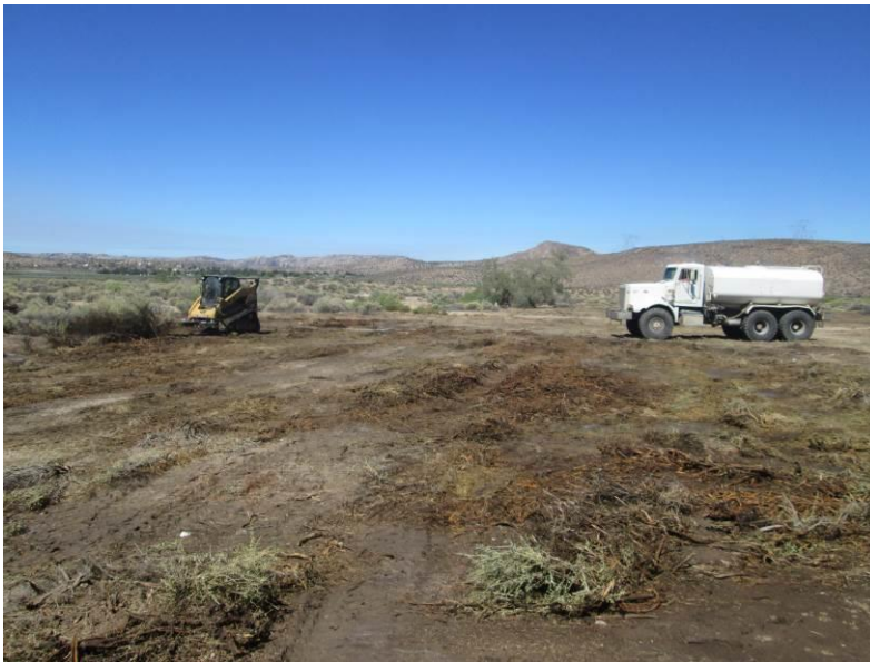
Photo 8: Construction crews are observed clearing and grubbing portions of Carrizo Gorge Fly Yards 1 and 2.
