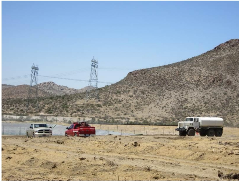
Photo 5: In accordance with Mitigation Measure FF-1, fire patrols are onsite during construction hours and for 1 hour after the end of daily construction.
