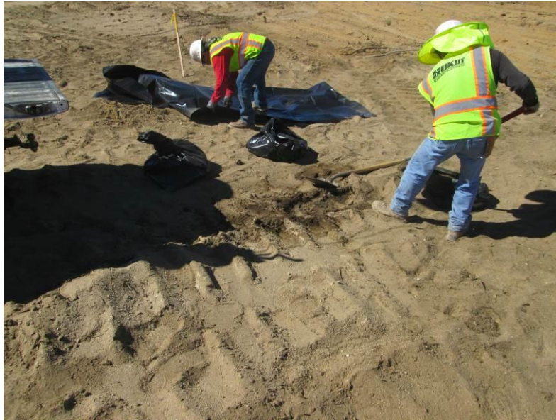
Photo 3: Construction crews clean an oil leak in accordance with Mitigation Measure HAZ-5a and the Spill Prevention Control and Countermeasure Plan.
