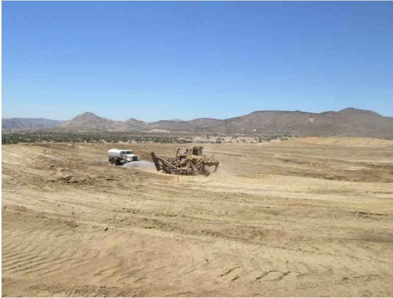
Photo 1: Water trucks are utilized during grading activities at the western portion of the ECO Substation to minimize fugitive dust in accordance with Mitigation Measure BIO-4a and the Dust Control Plan.
