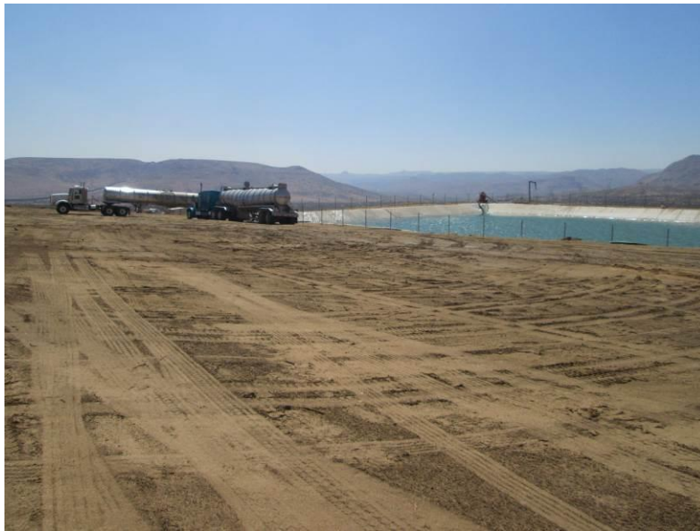
Photo 6: SDG&E continued to fill the temporary retention basin with water for the site-development phase of the ECO Substation.
