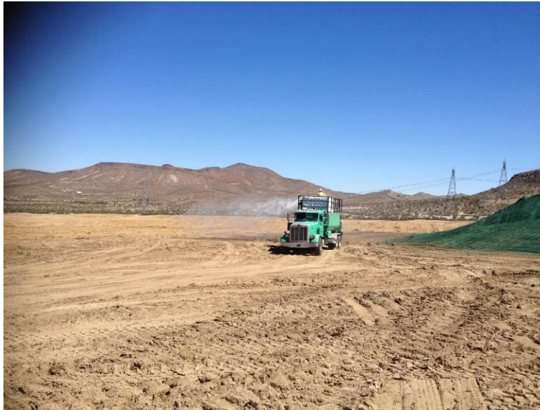
Photo 7: Soil stabilizer is placed along the temporary retention basin to minimize the potential for fugitive dust in accordance with Mitigation Measure AQ-1.
