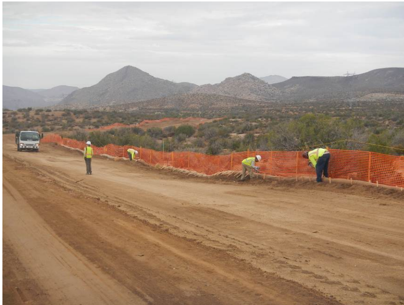
Photo 8: BMP's consisting of straw wattles and silt fencing are installed along the Southern Access Road in accordance with the SWPPP and Mitigation Measure HYD-4.
