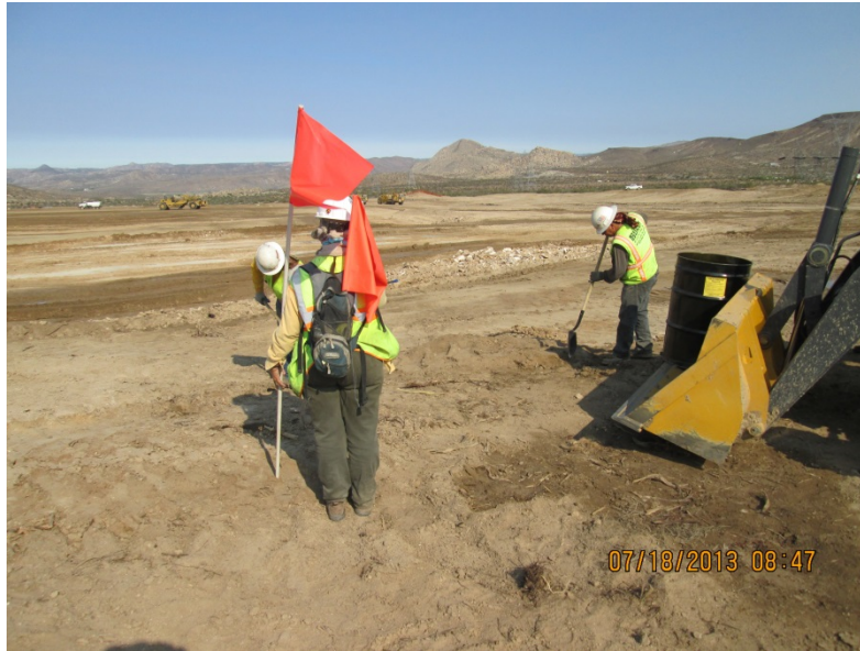
Photo 3: Construction crews remove stained soil in accordance with Mitigation Measure HAZ-5a and the Spill Prevention Control and Countermeasure Plan.
