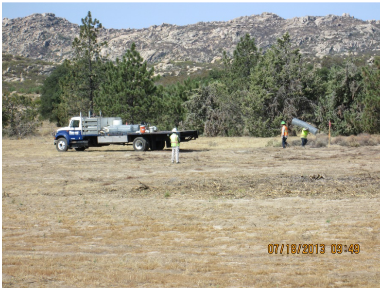
Photo 6: A biological monitor oversees construction activities associated with fence installation in accordance with Mitigation Measure BIO-1a.
