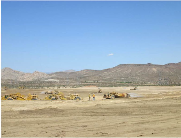
Photo 5: Water being utilized for dust control during earthwork activities in accordance with Mitigation Measure AQ-1
