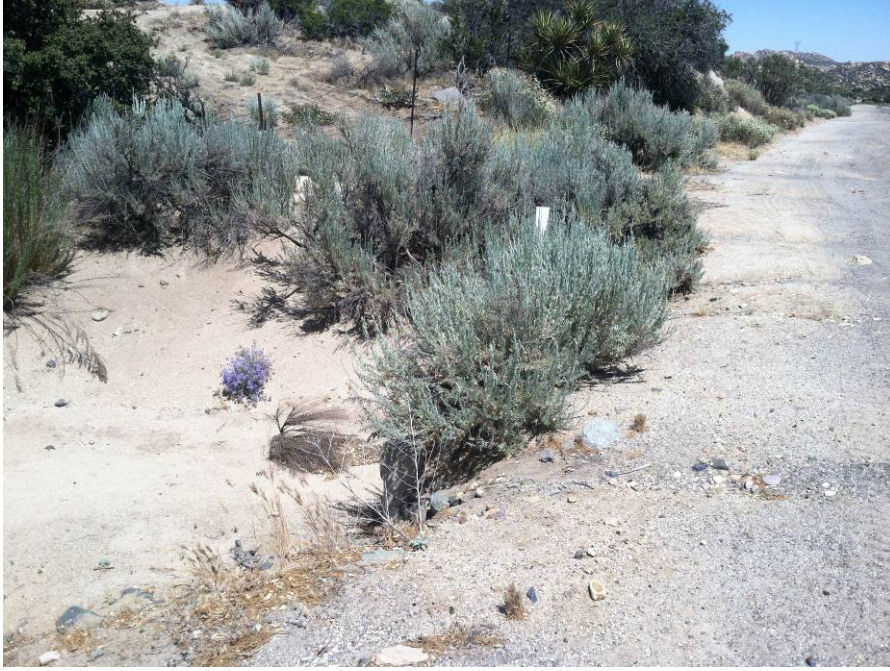
Photograph 1: View of the northern end of the culvert replacement site facing east.
