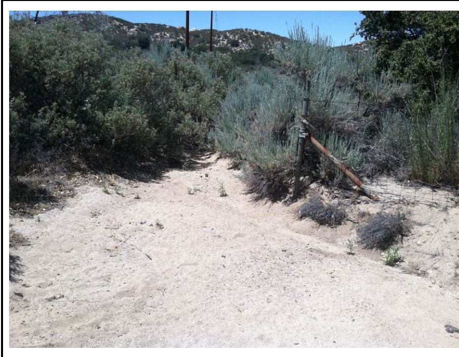
Photograph 5: View of the drainage to the north of the expanded culvert location, facing north.
