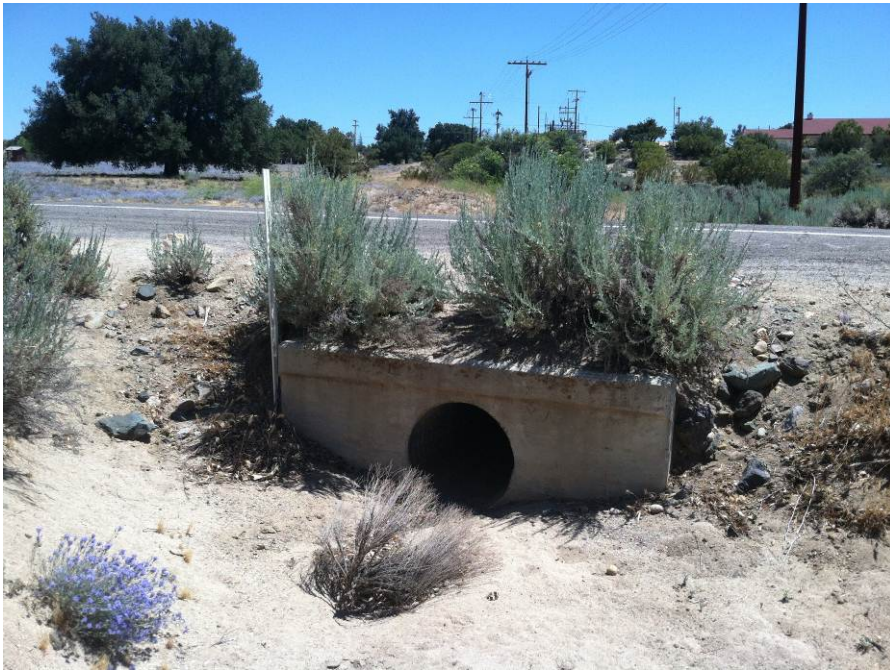
Photograph 2: View of the northern end of the culvert replacement site facing south.
